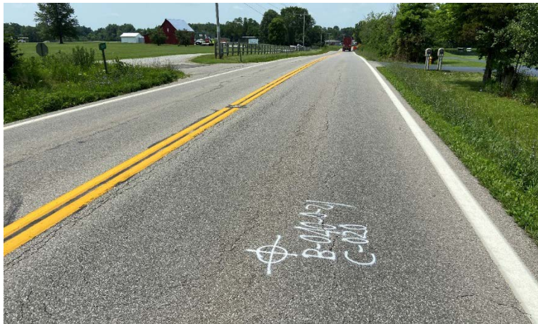
Photograph 3: Pavement condition of US-36 (Ohio Route 257 to Lehner Woods Boulevard)
