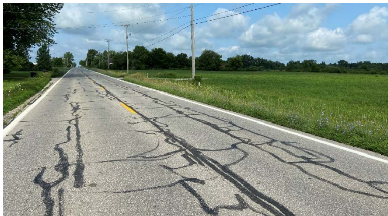
Photograph 1: Pavement condition of US-36 (County Line Road to North Main Street)
