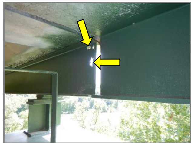
Photo 10 – 100% section loss in the right railing fascia stringer web (looking southeast at Stringer 11 at Pier 4).
