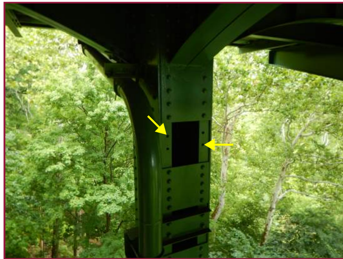
Four open holes in the south column angles of Column 1 (looking northeast).
