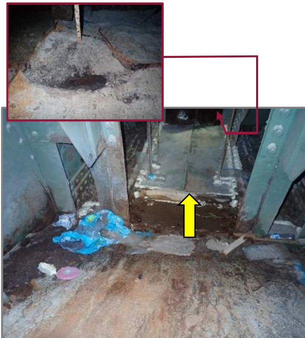
Photo 41 – Debris and water ponding in the south side of the Pier 6 cap with access to the column blocked by painting containment plywood (looking north). Inset: Looking east at blasting debris in the north half of the cap and 100% section loss in the bottom flange longitudinal stiffener.
