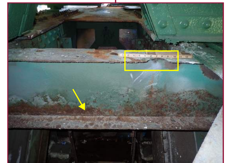
100% section loss in the top flange of the pier cap strut (looking south near Stringer 9). Note the typical corrosion in the pier cap.
