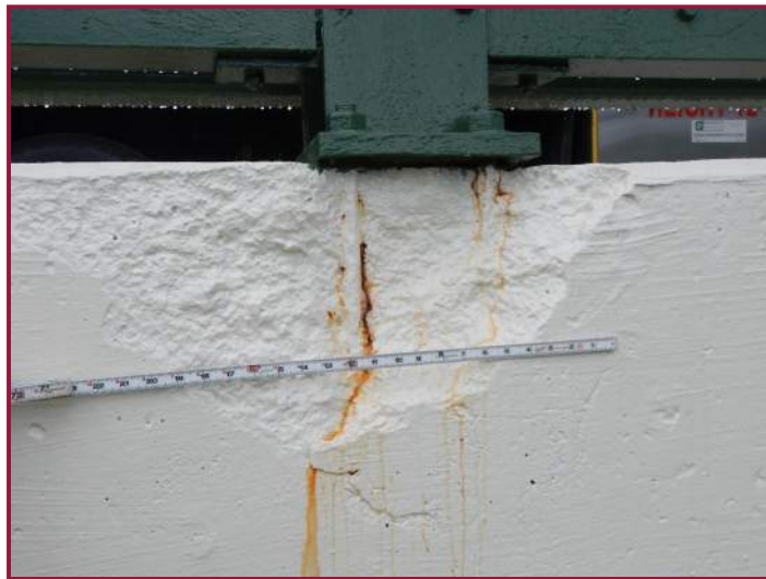
Spall with exposed railing post anchor bolts with minor rust staining in the concrete portion of the left railing (looking south).
