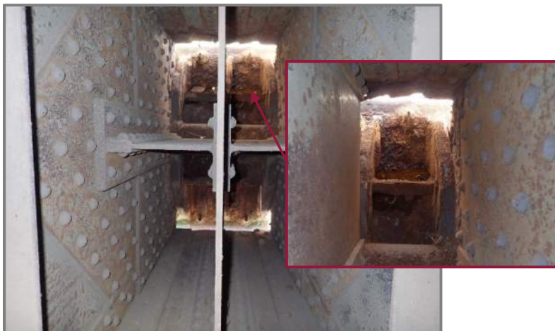
Photo 28 – Moderate laminate corrosion on the web plates and stiffeners at the Span 5 left arch bearing (looking east at the Pier 5 bearing). Note the anchor bolt nut with up to 100% loss on the uphill side.
