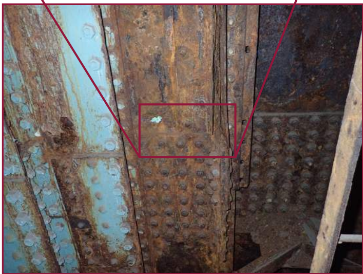
Corrosion hole in the north web plate and 2" thick pack rust between outstanding stiffener angle legs (looking north in the lower half of the Pier 7 left column).
