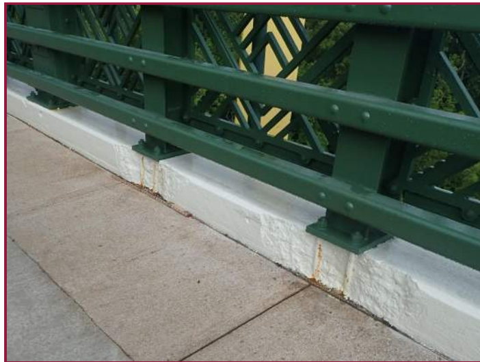
Spalls with exposed railing post anchor bolts in the concrete portion of the left railing (looking northwest).
