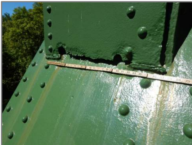
Photo 24 – Typical poor quality welds between the spandrel column web plates and the arch top flange and 100% section loss in the column web plate (looking west at the forward web plate of Column 11 at the top flange of the right arch in Span 5).
