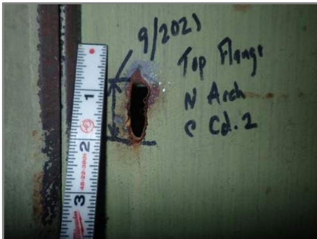
Photo 22 – Corrosion hole in the Span 8 left arch top flange plate at Column 2 (looking west at the interior).
