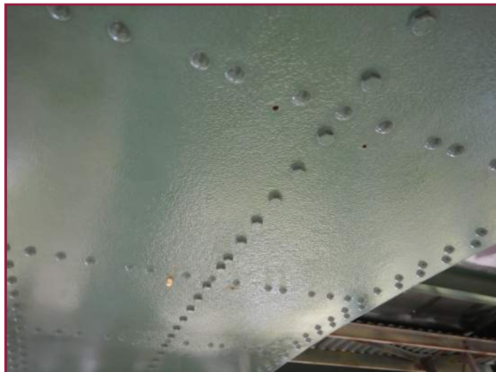
1/16" deep pitting throughout the underside of the pier cap (looking south).
