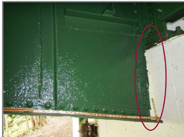
Photo 15 – Beam 11 at the Rear Abutment with 100% section loss in the transverse stiffener and painted over pitting throughout the web and flanges (looking south).
