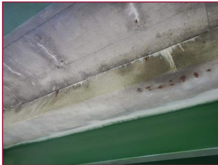
Hairline transverse cracks with efflorescence in the sidewalk underside and efflorescence at the joint with the deck (looking northwest).
