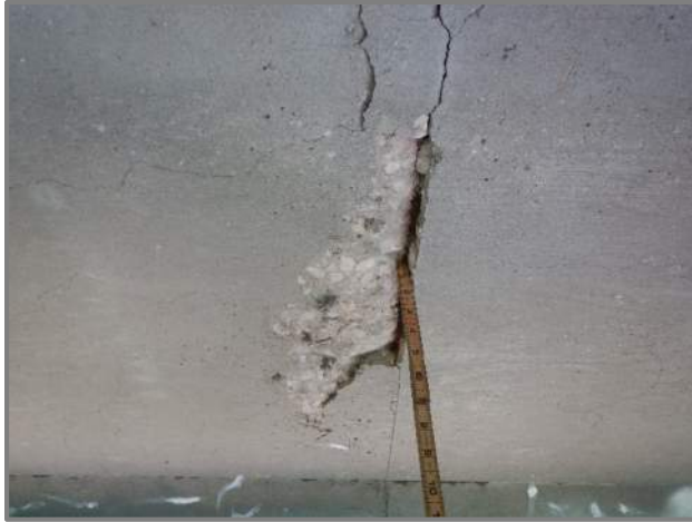
Photo 2 – Spall in the deck underside at the right forward end of Span 7 (looking up and south between Floorbeams 11 and 12).
