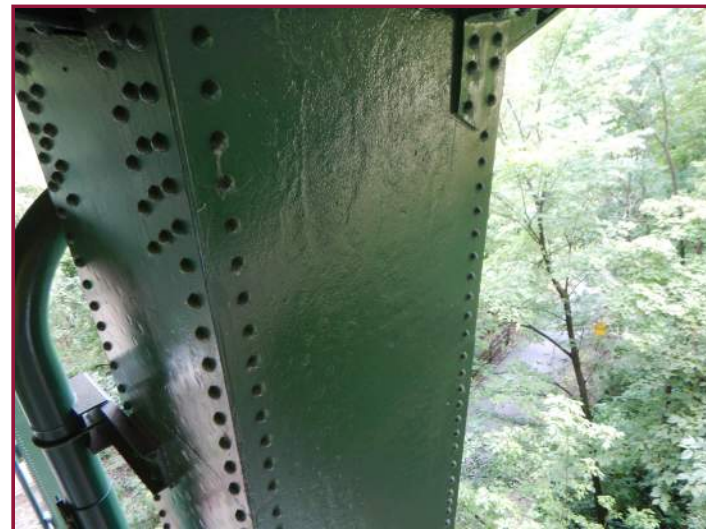
Pitting up to 1/8" deep in the rear face of the Pier 2 column (looking southeast).
