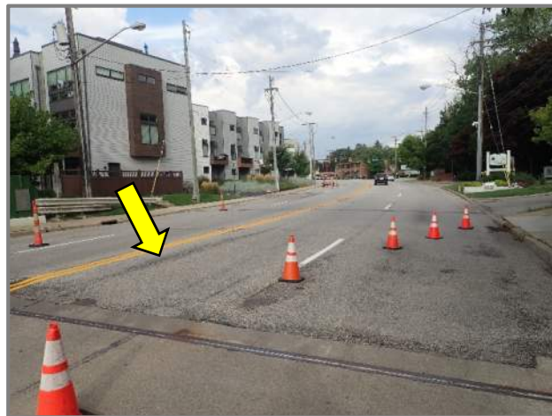
Photo 46 – Full length longitudinal cracks and deteriorating asphalt patches in the rear approach wearing surface (looking west).
