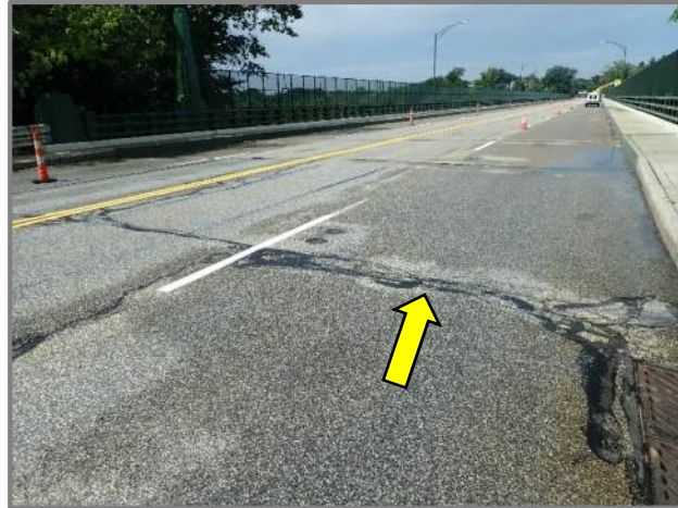
Photo 45 – Forward approach slab with transverse map cracking along the forward edge (looking west).
