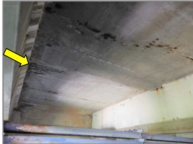
Photo 14 – Forward Abutment slab underside with full length longitudinal cracks and a spall with exposed reinforcement at the left rear end (looking north).
