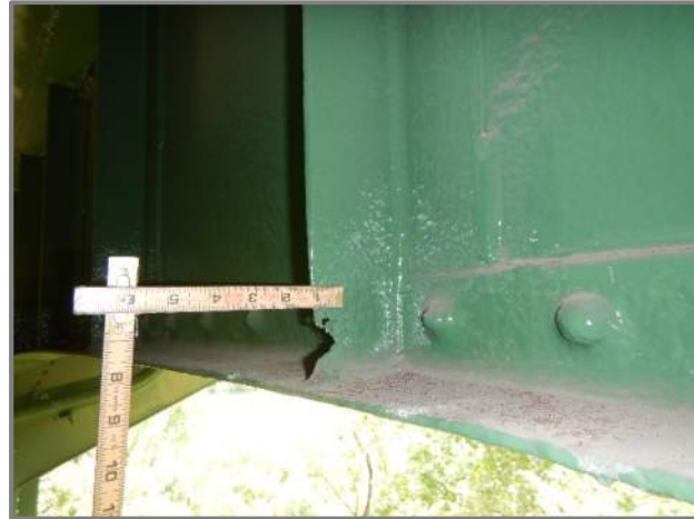
Photo 17 – Beam 3 transverse stiffener with 100% section loss at the bottom 3" (looking southeast at midspan of Span 4).
