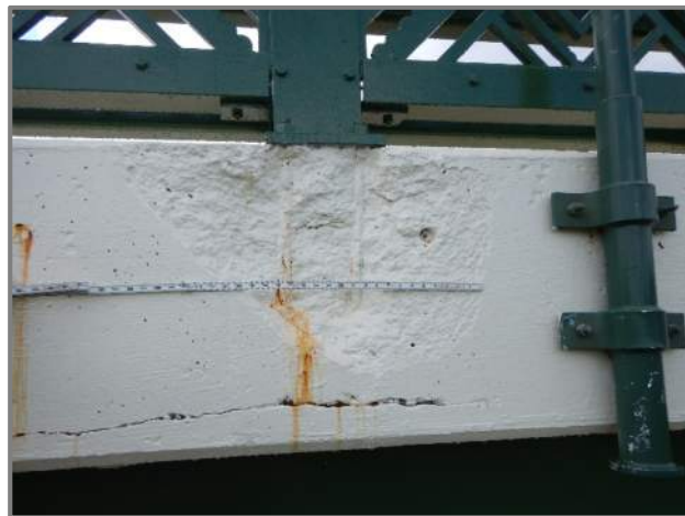
Photo 9 – Typical spall in the concrete portion of the railings with exposed railing post anchor bolts (looking south near midspan of Span 7).
