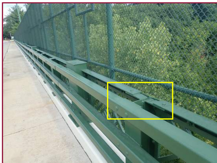
Missing railing post cap plate with minor section loss in the top of the post (looking west).
