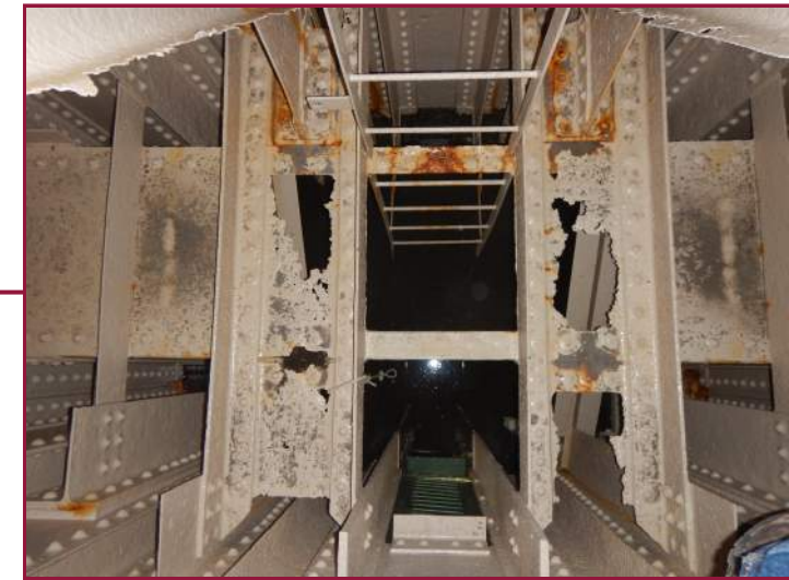
Painted over 100% section loss in the column interior diaphragms (looking down and south near the base). Note the water ponding at the bottom of the column due to the clogged drainage pipe.
