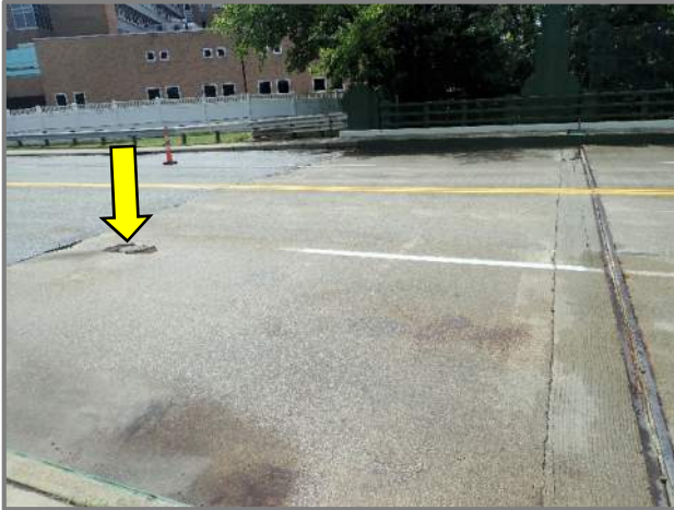
Photo 5 – Overall view of the Forward Abutment slab wearing surface with a 2' diameter spall at a failing asphalt patch (looking south).
