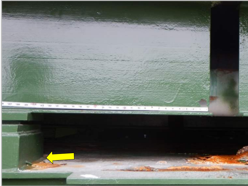
Photo 1 – Tower pier cap top flange at the stringer bearing plate attached by fillet welds with no transition radius ( Category E' ). The north end of the pier cap top flange at the Stringer 1 bearing is shown (looking south).
