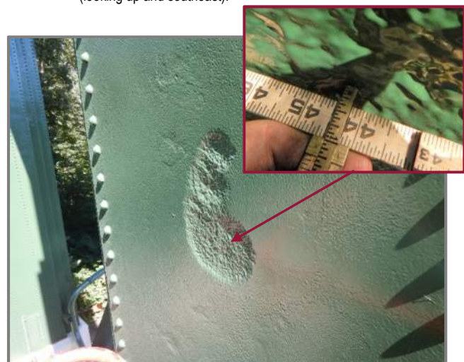
Photo 36 – Pier 6 right column exterior with 3/8" deep pitting in the rear web plate (looking northeast).
