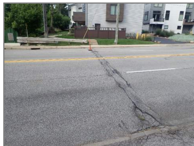
Photo 47 – Overall view of the rear approach relief joint which is heaved upwards (looking south).
