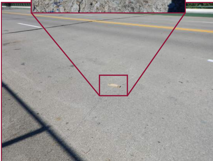
Hairline diagonal and transverse cracks in the wearing surface (looking northwest).
