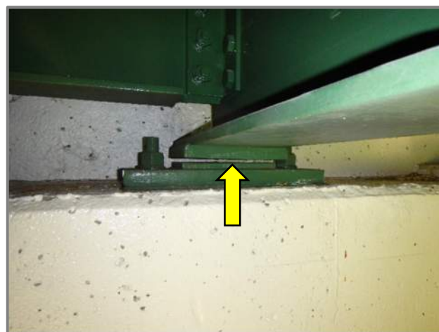
Photo 16 – Beam 10 floating at the Rear Abutment due to a missing shim plate (looking west).
