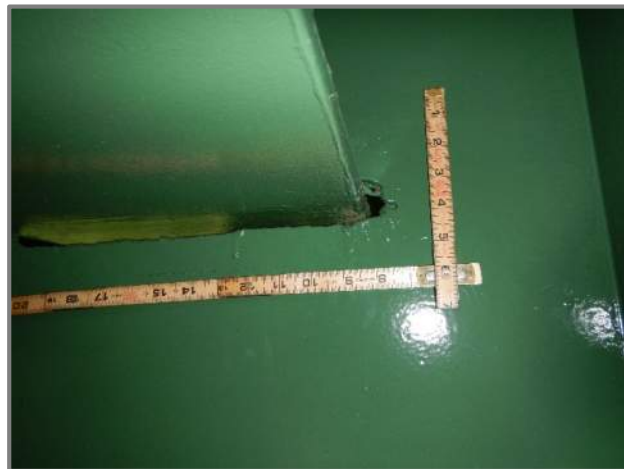
Photo 40 – 1/4" long overcut in the rear face of the Pier 3 web at the Beam 6 bottom flange (looking east).
