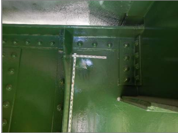
Photo 26 – Construction damage in the web of Floorbeam 3 in Span 6 (looking east at the rear face between Stringers 7 and 8).
