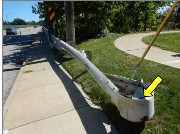
Photo 48 – Impact damage to the left rear guardrail; note the broken and missing end post (looking east).
