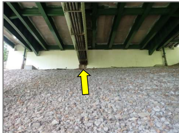
Photo 49 – The conduit at the Rear Abutment with 100% section loss in the underside of the conduit and minor water staining on the abutment wall below (looking west).
