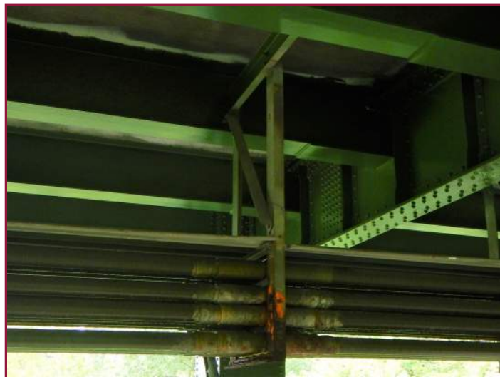
Corrosion at the bottom of the utility hanger (looking southwest).
