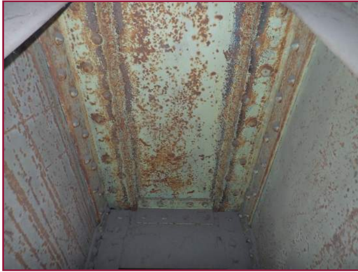
Typical minor surface corrosion at the interior of the arch (looking east).
