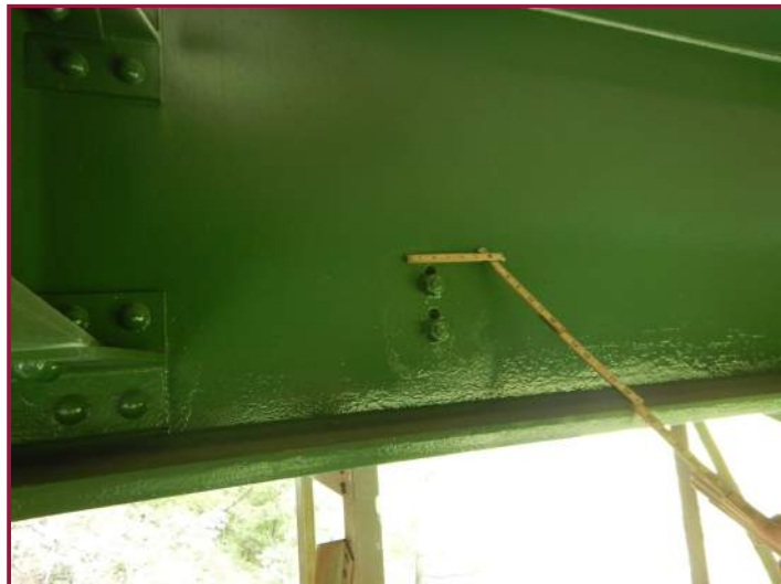
Typical misdrilled holes in Beams 7 and 8 at the utility bracket connections (looking south).
