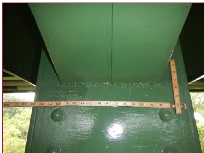
Poor quality weld between the floorbeam bottom flange and the spandrel column (looking north).
