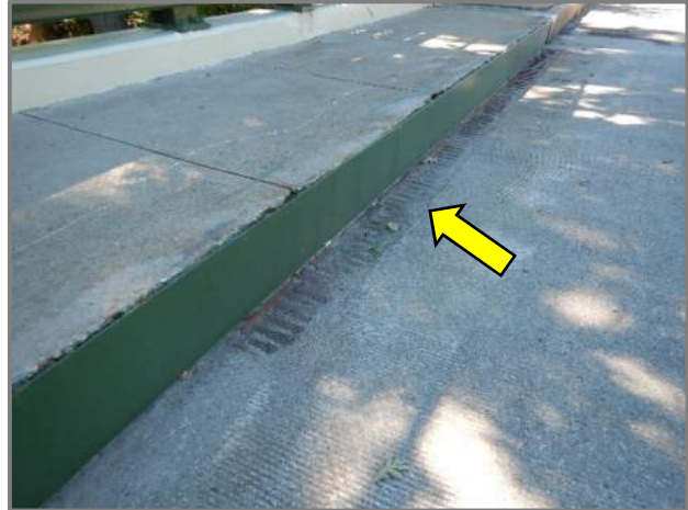
Photo 11 – Scuppers at the right rear end of Span 1 full of debris (looking southwest).
