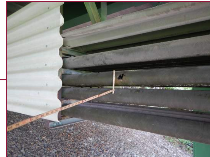
3" diameter hole in the utility conduit below Pier 1 (looking northwest).
