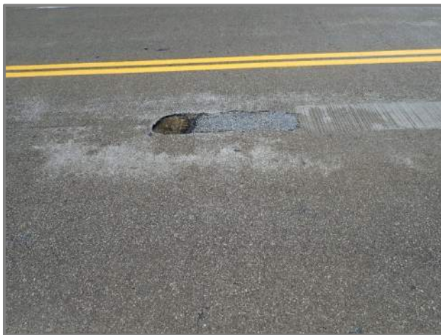
Photo 4 – 1 1/2" deep spall in the wearing surface with water ponding at a failing asphalt patch (looking south at the forward end of Span 9).
