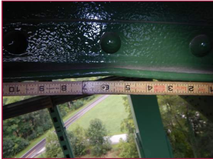
Minor distortion in the jack arch bottom flange with the left angle outstanding leg bent up 1/4" over 6" (looking south).
