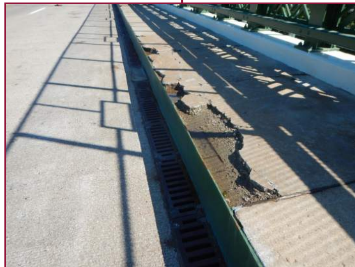
Spalls with exposed reinforcement and water ponding in the right sidewalk (looking east).
