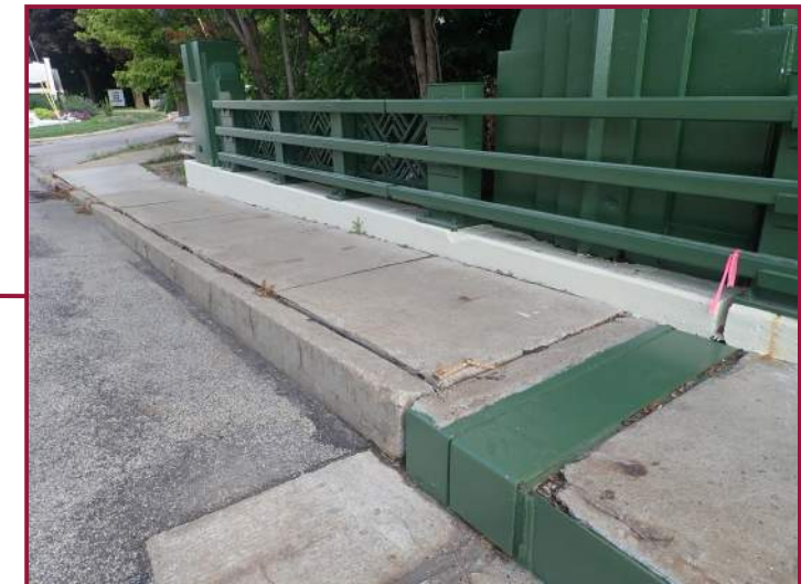
2" vertical misalignment between the left rear approach sidewalk and the bridge (looking northwest).
