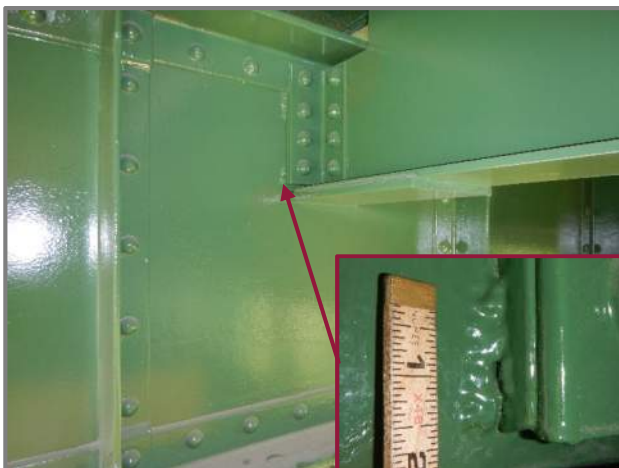
Photo 25 – Cracked tack weld at Floorbeam 4 at the Stringer 6 connection angle fill plate in Span 6 (looking southeast).
