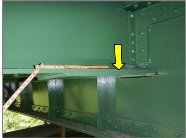
Photo 34 – Typical partial length welded moment cover plate at the beam/stringer flange at the floorbeams (looking southwest in Span 4 at the Beam 6 bottom flange near Pier 3).
