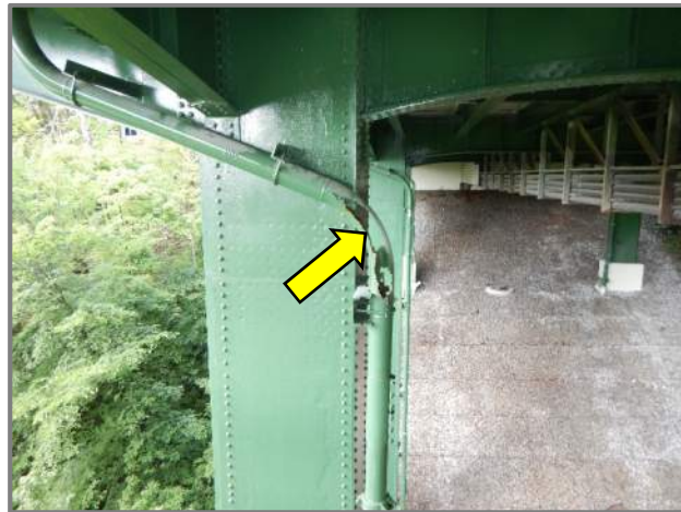
Photo 12 – 100% section loss in the downspout at the right side of Pier 3 (looking west).
