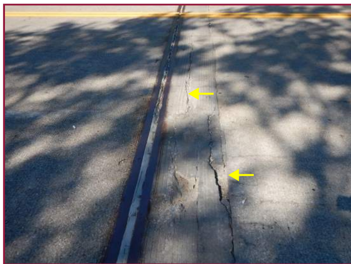
Spalls and transverse cracks in the joint header (looking north).
