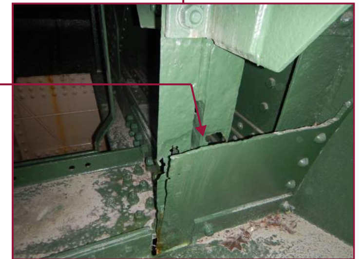
Painted over 100% section loss in the pier cap interior stiffener angles (looking northeast near the south end of the pier cap).
