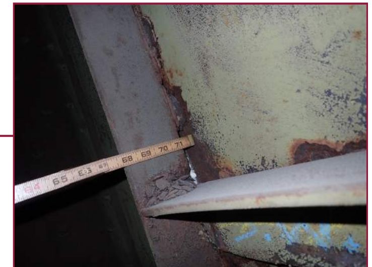
Up to 3/4" thick pack rust between the south web and the intermediate hatch door (looking southeast in Bay 12 of the arch interior).
