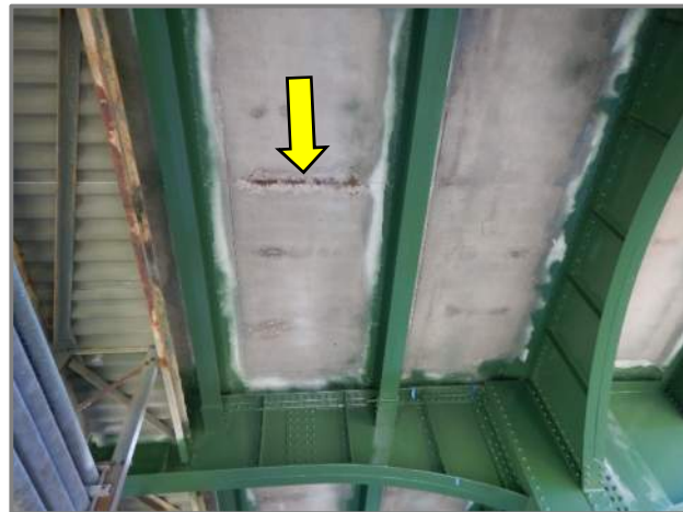
Photo 1 – Isolated spall with exposed reinforcement and adjacent typical hairline transverse cracks in the deck underside (looking up and east at the right forward end of Span 8).
