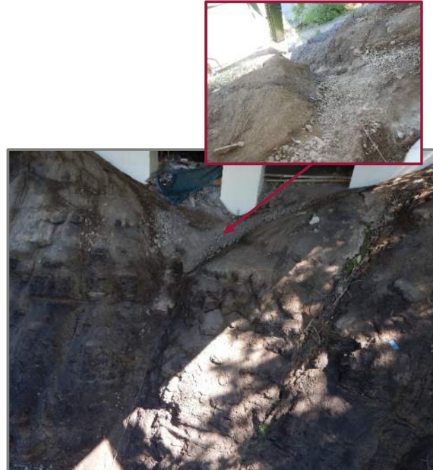
Photo 43 – Erosion channel at the Forward Abutment (looking east).
