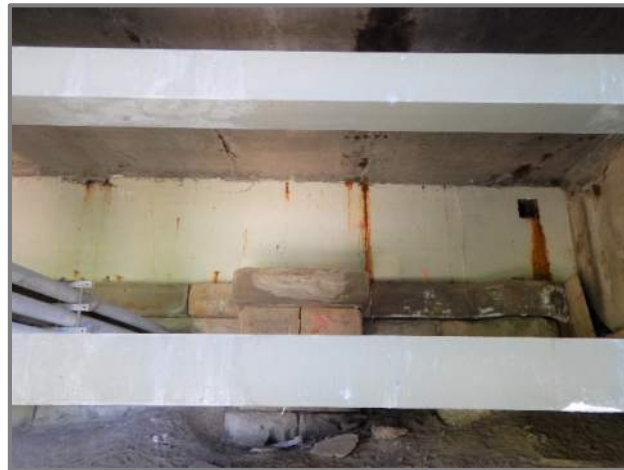
Photo 39 – Vertical hairline cracks and rust staining on the reinforced concrete portion of the forward wall at the Forward Abutment (looking east).
