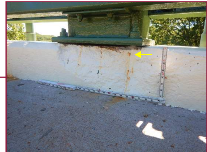
Typical sealed spall in the concrete portion of the railing with an exposed metal railing anchor bolt (looking south).
