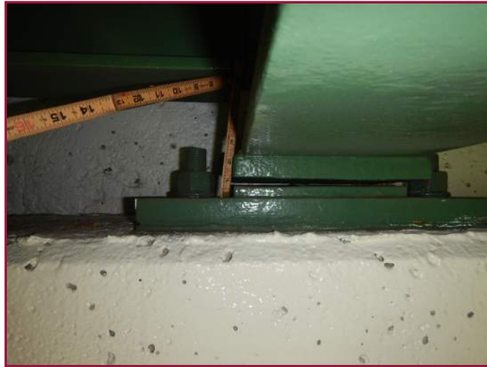
Missing shim plate with a 1/4" gap between the sole plate and the masonry plate (looking west).
