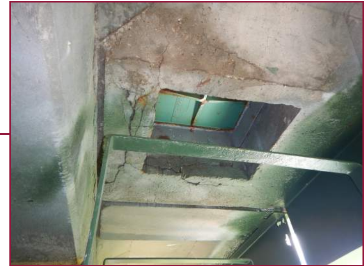
Delaminations and minor water staining in the underside of the sidewalk at the pier cap access hatch (looking east).
