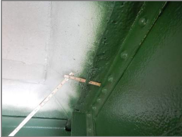
Photo 23 – 100% section loss in the top flange angle of the Span 7 right jack arch (looking east near Pier 7).
