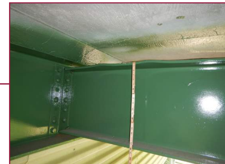
Diaphragm top flange bent up 1/2" over 9" in two locations (looking east).
