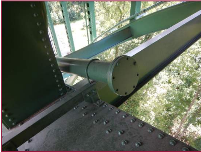
Only 2 of 8 bolts in place at the drainage cover plate (looking southeast).
