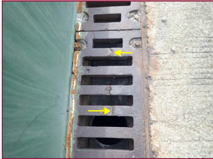
Scupper grate with full depth cracks in five of the bars (looking east near the left curb).
