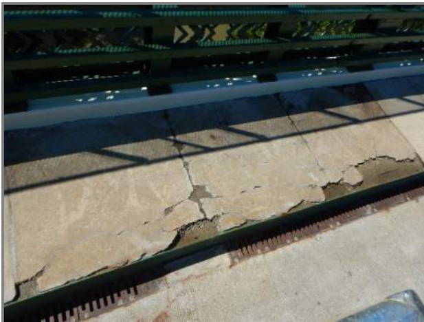
Photo 6 – Spalls with exposed reinforcement in the right sidewalk with water ponding (looking south near midspan of Span 8).
