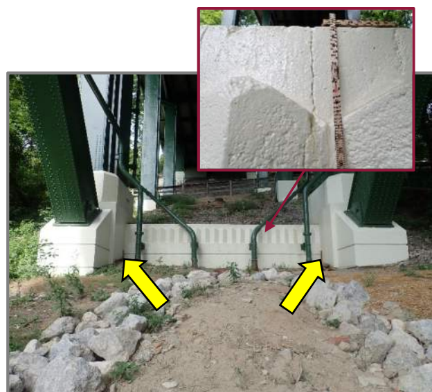
Photo 38 – Pier 4 reinforced concrete pier wall with a typical sealed vertical crack and minor rust staining below the column drainage holes (looking west).
