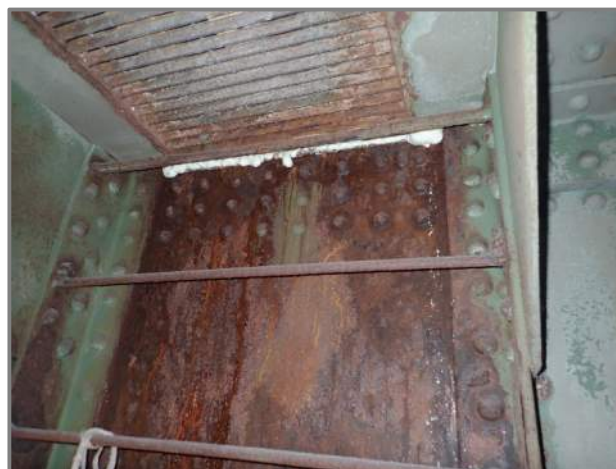
Photo 42 – Laminated corrosion at the top of the Pier 6 right column below the painting containment (looking up and south).
