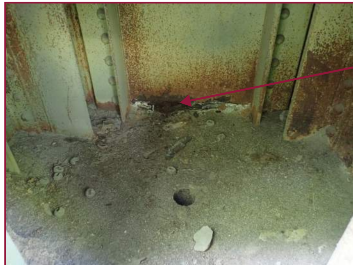
Pitting up to 5/32" deep in the interior face of the Pier 3 left column forward web at the concrete interface (looking east).
