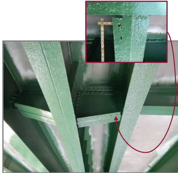
Photo 30 – 100% section loss in the bottom flange of the diaphragm between Beams 10 and 11 at midspan of Span 4 (looking west). Inset: Looking up and south at the forward bottom flange angle.
