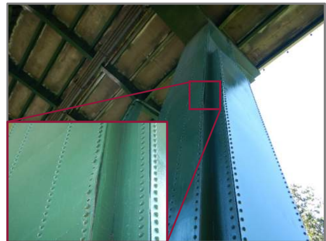
Photo 35 – Missing fasteners at the left rear corner of the Pier 5 right column (looking up and southeast).
