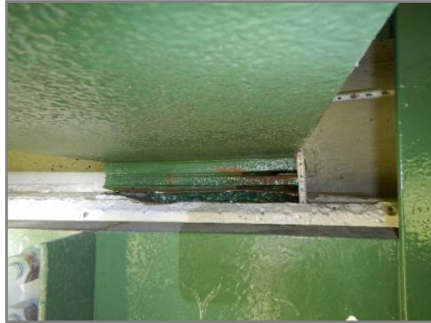
Photo 29 – Gaps up to 3/8" high between the right edge of the shim plates at the Forward Abutment fixed bearings (looking east at the Beam 8 Forward Abutment bearing).
