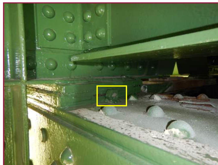
Nut painted to the top flange of the pier cap (looking northeast).
