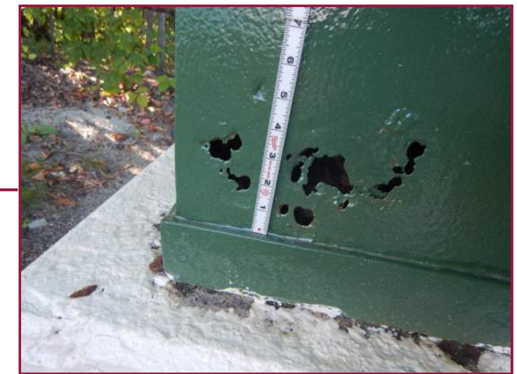
100% section loss near the base of the decorative railing obelisk (looking south).
