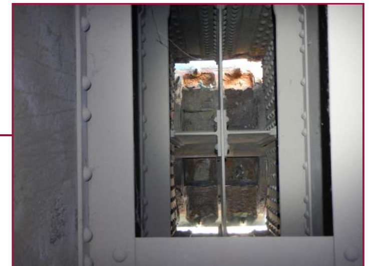
Typical laminate corrosion and bearing anchor bolt and nut section loss at the arch pins (looking west).
