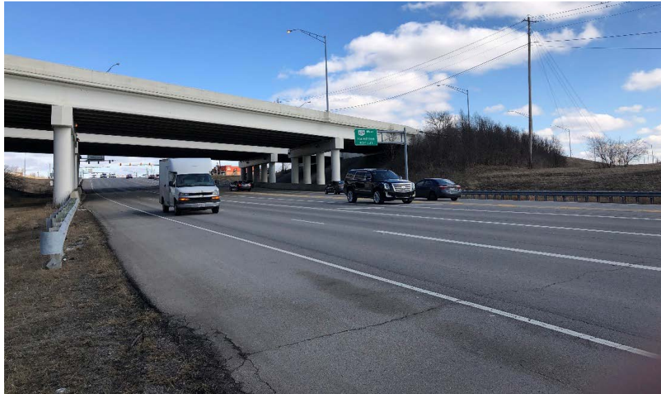
Photograph 1. Overall Pavement Condition of C.R. 19
