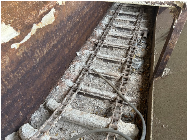
View of stockpiled material inside the concrete mixing machine in the building.
