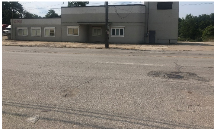
Photograph 1: SR-14 pavement condition at about STA 385+00 (end of project)
