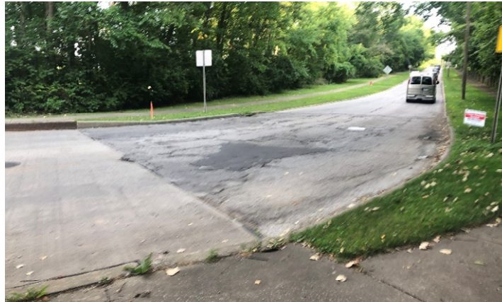
Photograph 2: Henry St pavement condition
