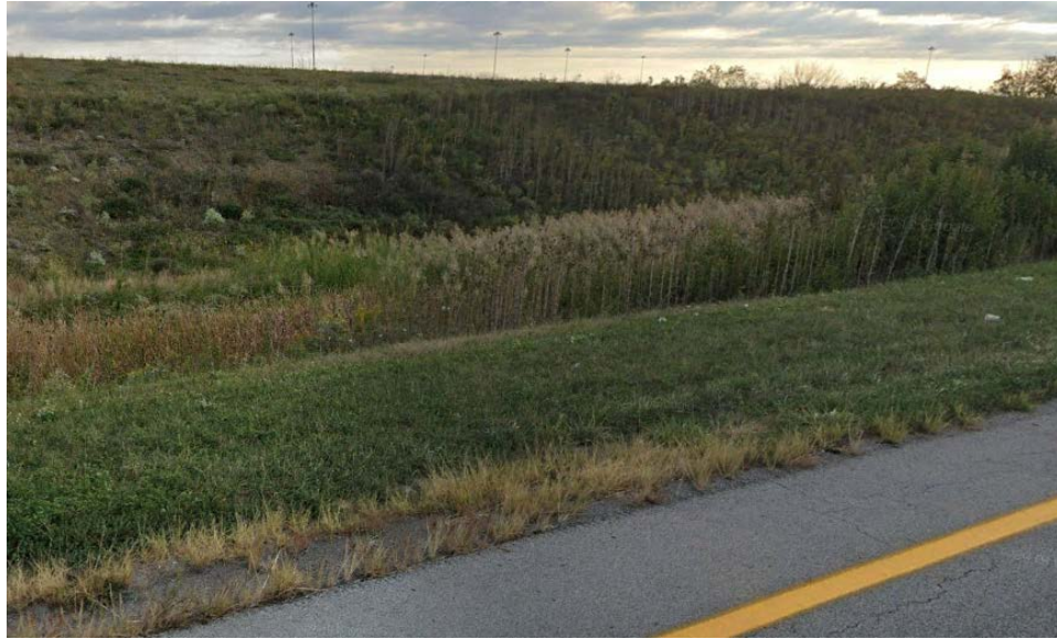
Photograph 2: Signs of Standing Water in Drainage Ditch
