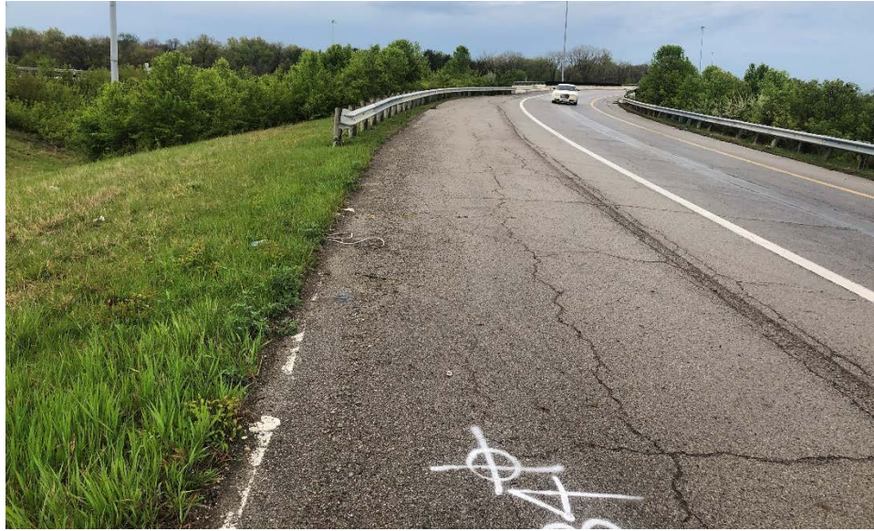
Photograph 8: Overall Pavement Condition of Ramp K West of IR-71
