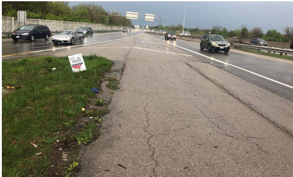
Photograph 7: Overall Pavement Condition of Ramp K East of IR-71
