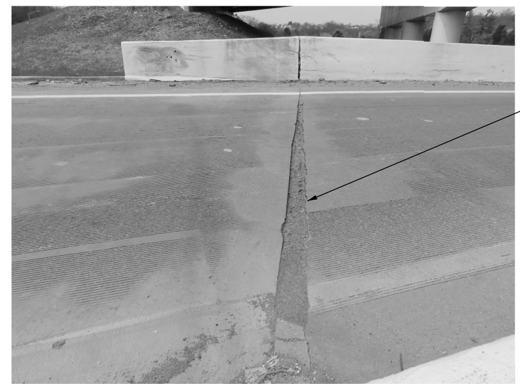
DECK DETERIORATION AT FORWARD ABUTMENT
