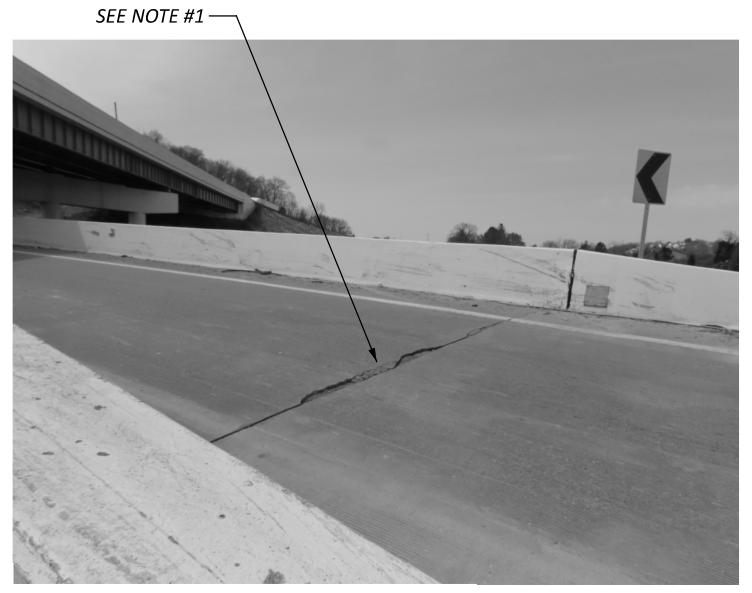
DECK DETERIORATION AT REAR ABUTMENT
