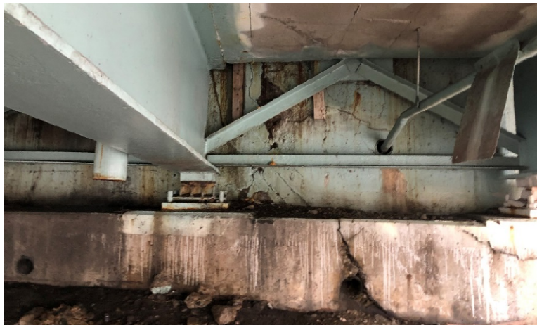
Photograph 2: Spalling, Cracking and Exposed Rebar Observed at Each Abutment
