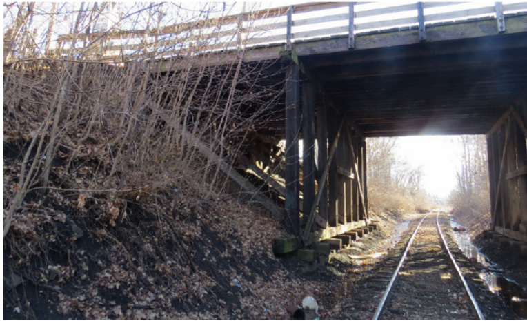
Photograph 2: Corrosion underside of bridge deck and deteriorated wooden beams
