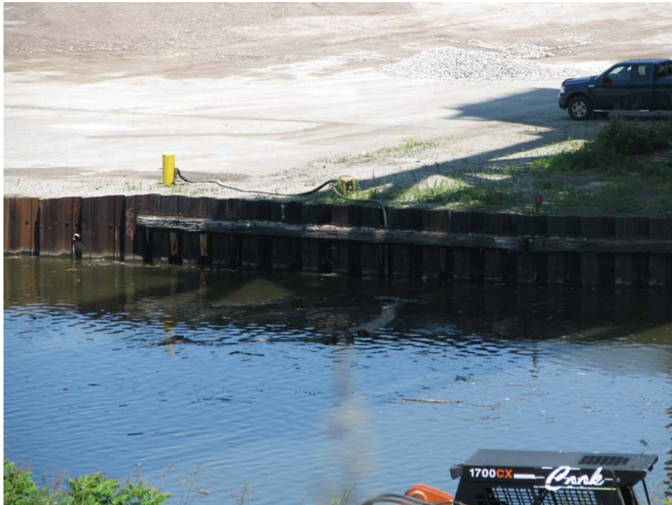
Photo 4: East bank bulkhead to be replaced.
