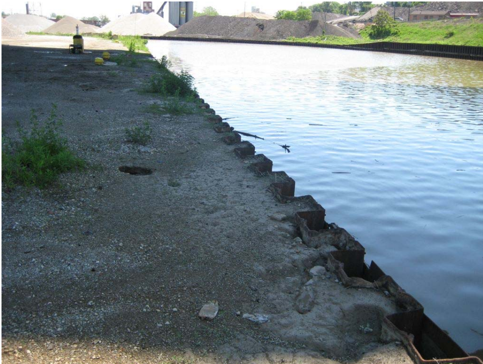
Photo 6: South facing view of east bank of the Cuyahoga River bulkhead to be replaced.
