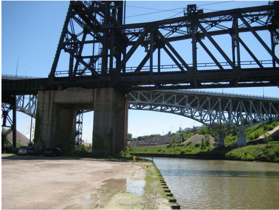
Photo 7: South facing view of east bank of Cuyahoga River bulkhead to be replaced.
