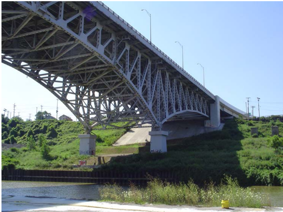
Photo 2: West facing view of west bank of Cuyahoga River bulkhead to be replaced.
