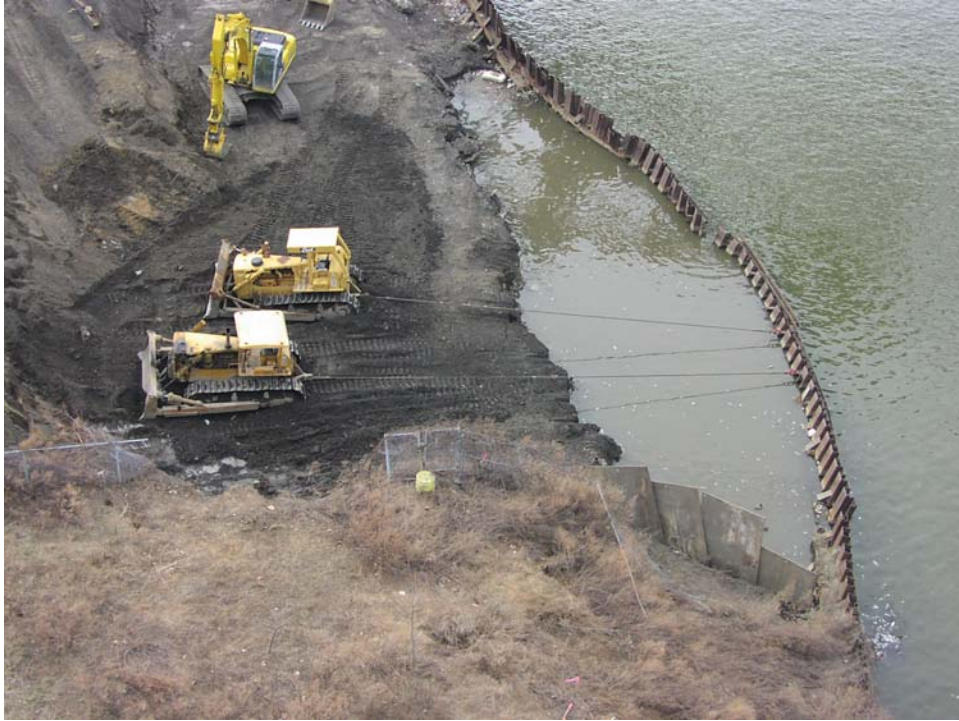
Photo 5: Failed West bank bulkhead to be replaced.
