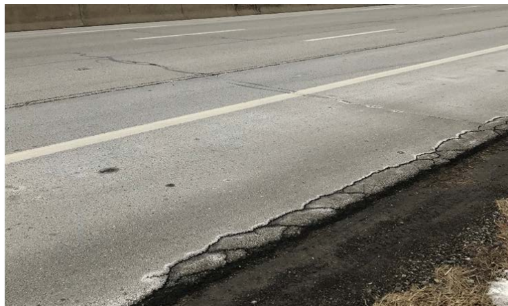
Photograph 1: IR-76 and IR-277 Pavement Wear
