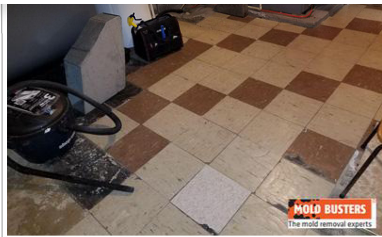
asbestos floor tiles
