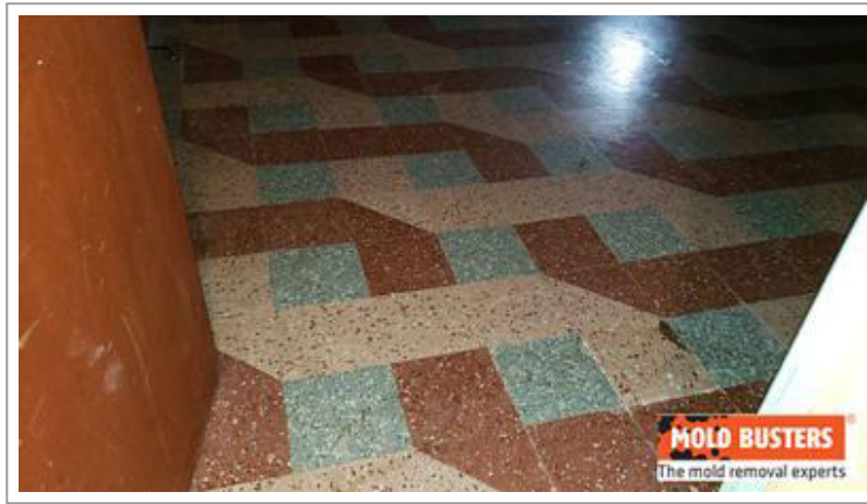
asbestos floor tiles
