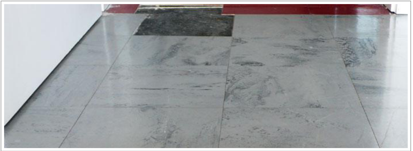
Vinyl Tiles with Asbestos
