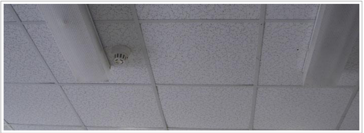
Acoustic Ceiling Tiles with Asbestos
