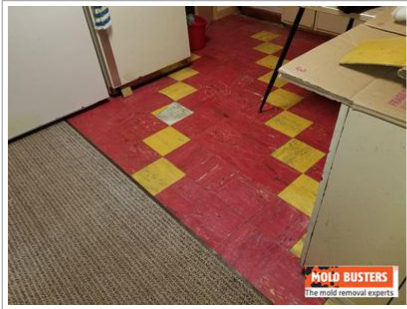
asbestos floor tiles
