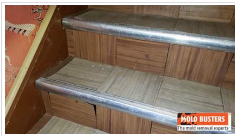
asbestos floor tiles
