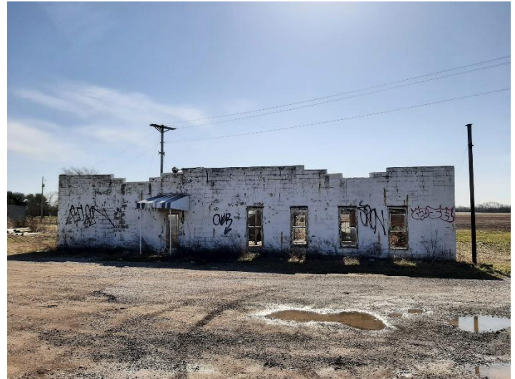
View of dilapidated building
