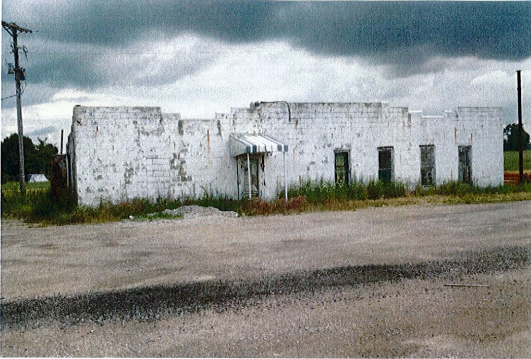
View looking southeast at dilapidated structure
