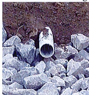
below-PVC outlet with animal guard and stone protection
