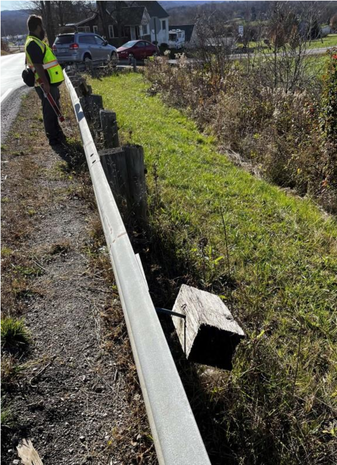
(Rotted, dislocated, and/or missing posts)
