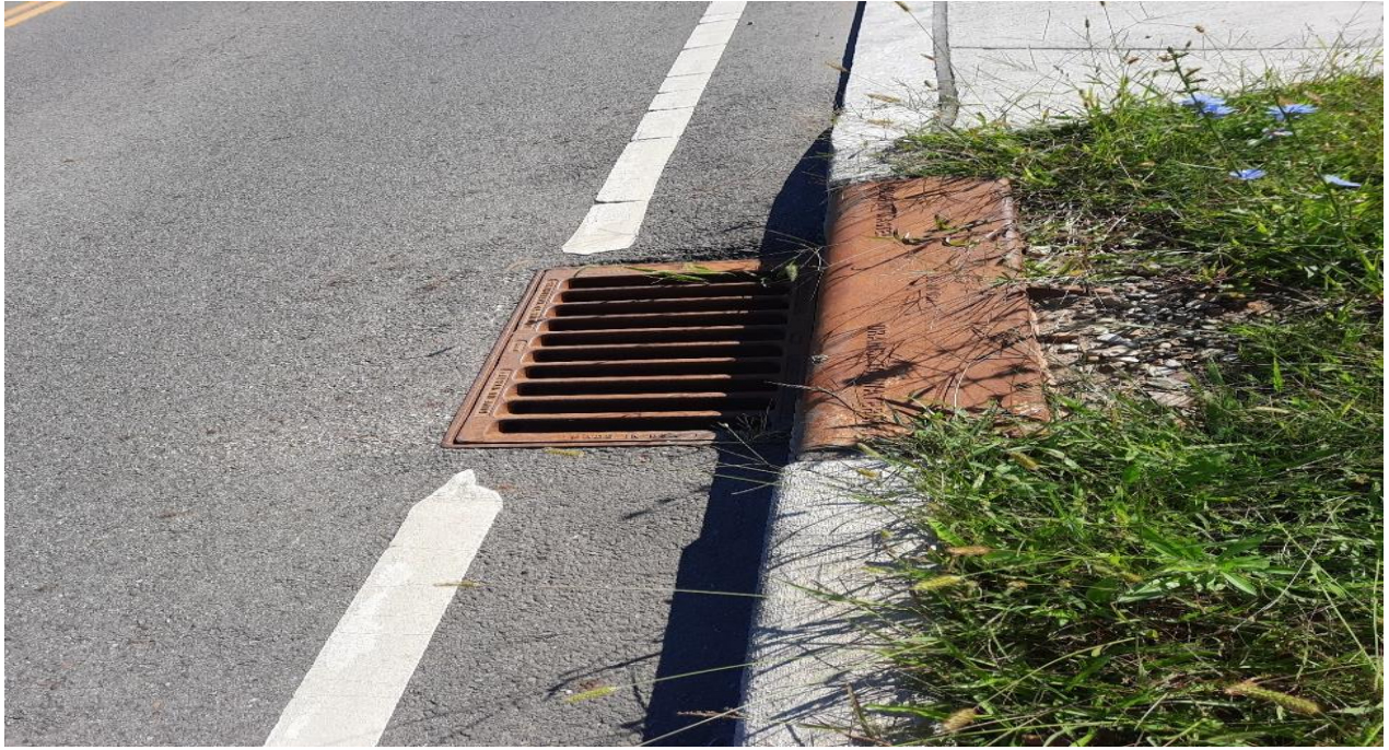
(Drain cover near baseball field is facing against the flow of right-hand traffic)
