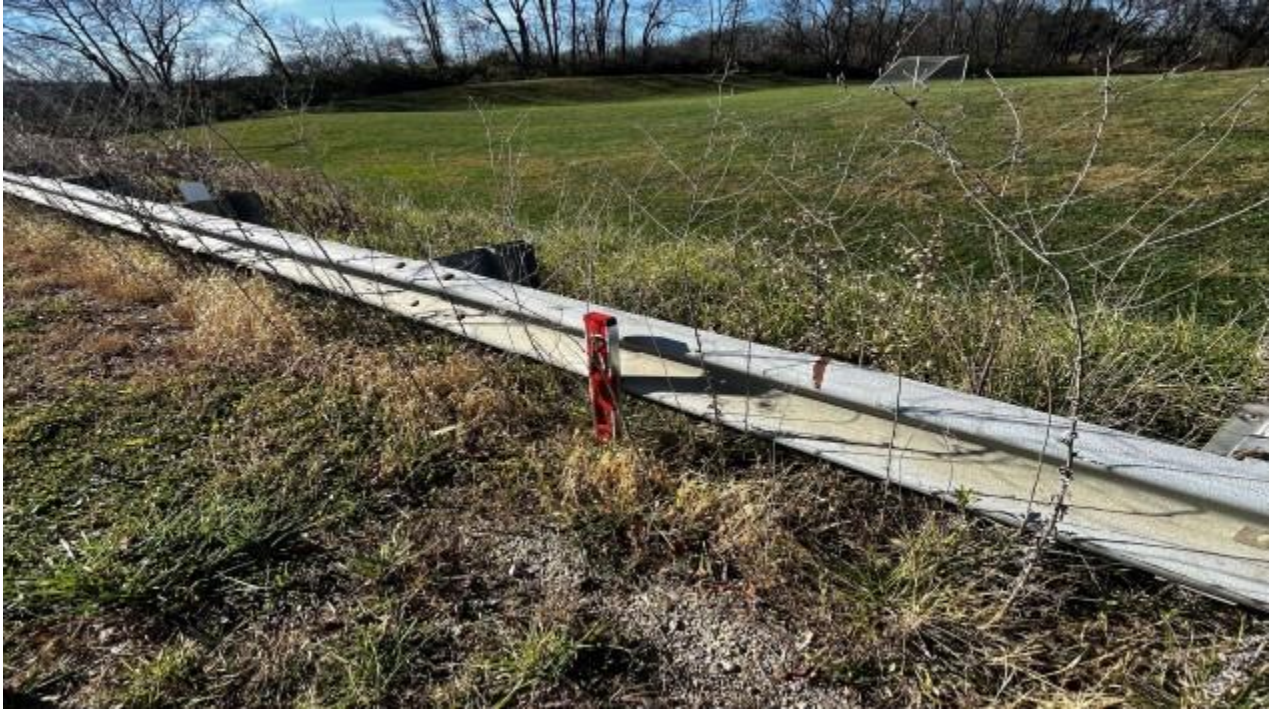
(Guardrail under 2 feet in height as appose to 3-foot standard)
