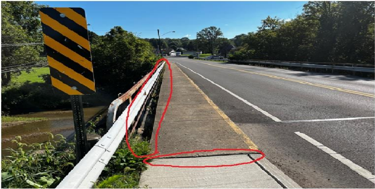
(6-7-inch gap between guardrail and sidewalk)
