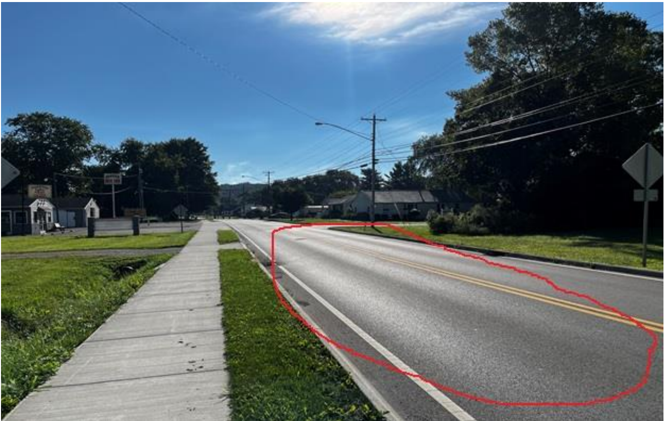
(Road deformation and aggregate polish)
