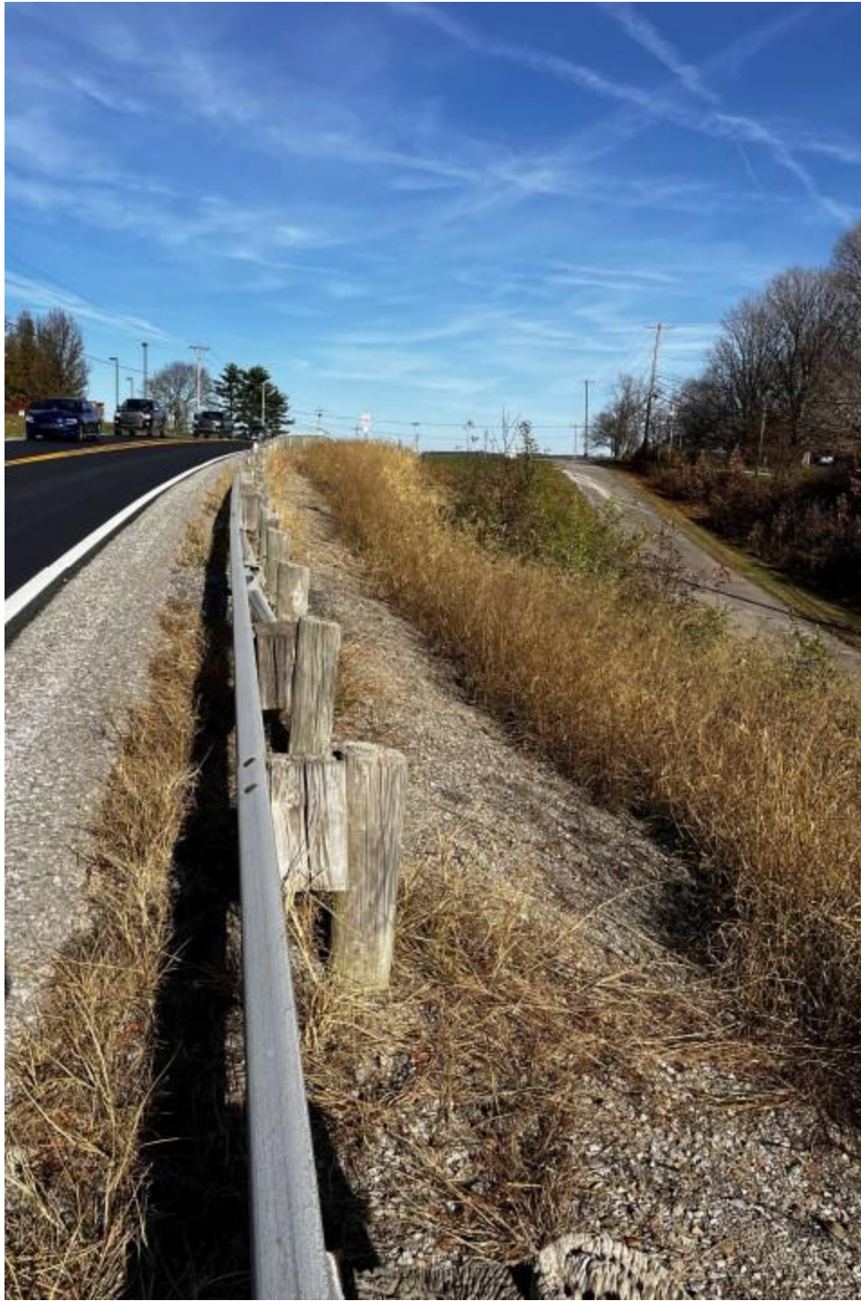
(Rotted posts and blocks)
