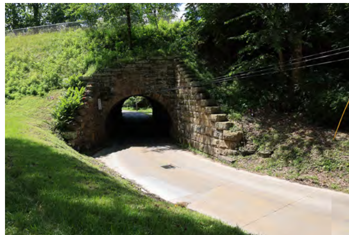
Connection to Old Hanover through the Tunnel is currently a barrier for Pedestrians, and not ideal for Cyclists.
