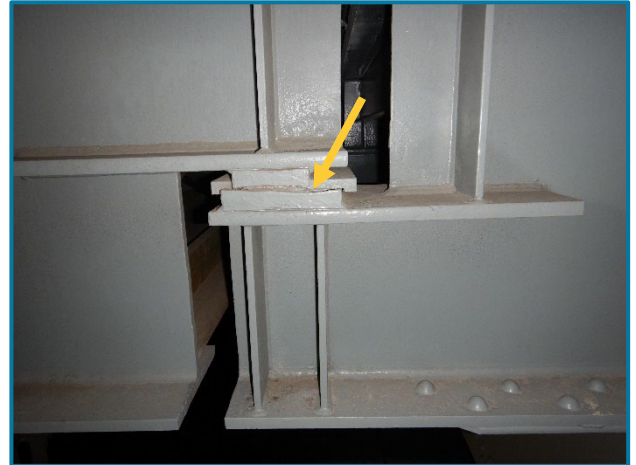
Photo 47 – Typical area of section loss painted over on the bearing plates near Pier 4A (looking west).
