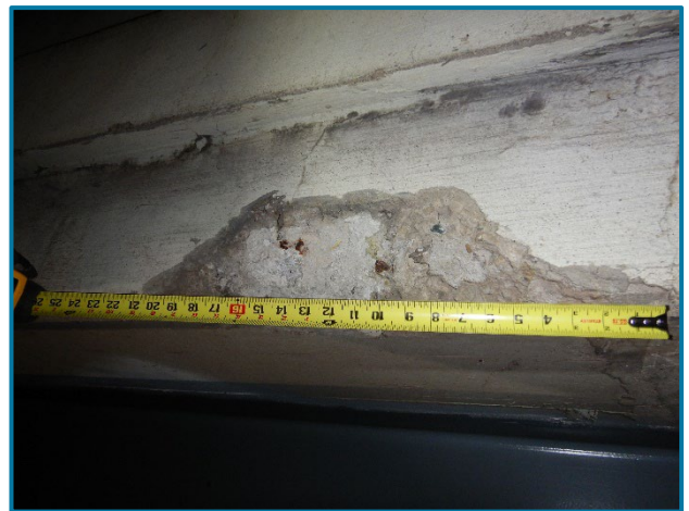
Photo 6 – 21" long by 12" wide by 1" deep spall on the east face of the east overhang near midspan of Span 1A (looking west).
