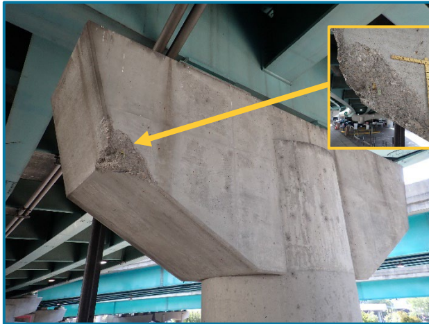
Photo 134 – 2' wide by 2' high by 4" deep corner spall with exposed reinforcement on the west face of Pier Cap 2 (FWW) (looking southeast).
