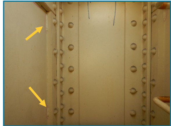
Photo 109 – 2"-3" tack welds at east end bearing fill plate (looking east inside of Pier Cap 9A).
