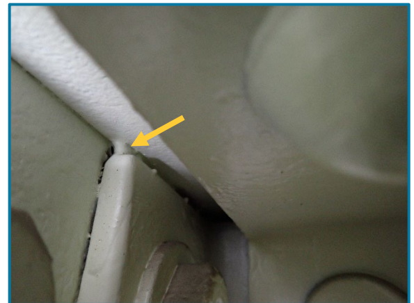
Photo 89 – 2" long tack weld along the south edge of the bottom flange plate below Girder F (looking south on the inside of Pier Cap 5A).
