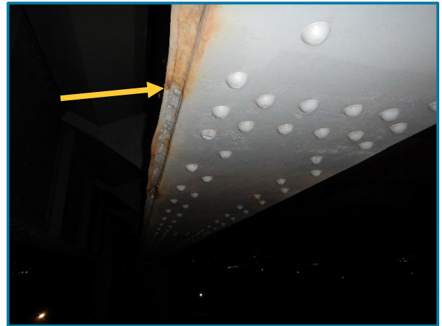
Photo 60 – Pack rust between the south web plate and bottom flange angles on the exterior of the River Pier Cap (looking west).
