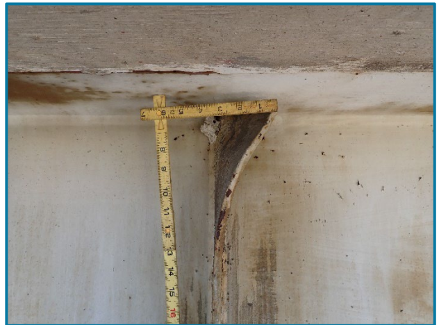
Photo 28 – Bent stiffener near the top flange on the east side of Girder E near Pier 21B in Span 22B (looking west).
