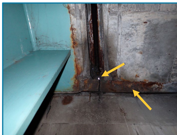
Photo 15 – Daylight shining through tears in the strip seal material between HAM-71-0000L and HAM-50-2091L (looking north). Note the rust and water staining to the underside of deck surrounding the torn strip seal.
