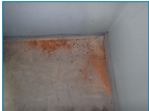
Photo 132 – Area of minor surface corrosion on the bottom flange plate near the east bearing on the interior of Pier 2 (FWW) (looking north).
