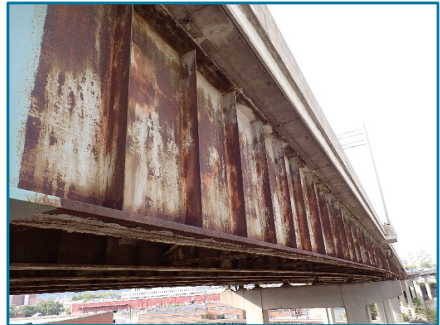
Photo 24 – Active corrosion throughout the east fascia girder in Span 16A (looking northwest).
