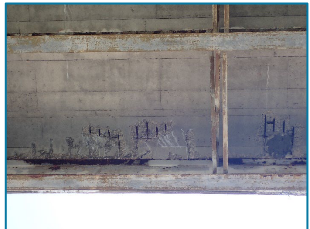
Photo 3 – Four spalls with exposed reinforcement in the underside of the deck between Girders D and E in Span 26B (looking up and west).
