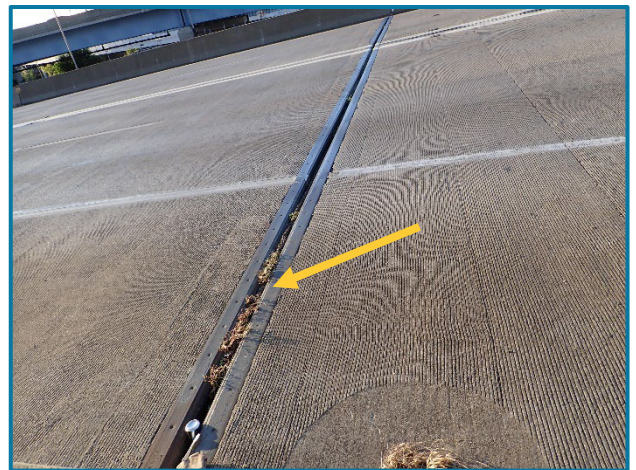
Photo 14 – Heavy debris impaction and vegetation growth in the strip seal expansion joint at the Wall Pier (looking south from the north railing).
