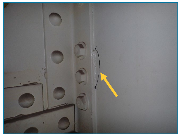
Photo 94 – 3" tack weld on the south web and girder diaphragm connection angles between Girders D and E (looking southeast inside of Pier Cap 6A).
