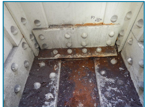
Photo 96 – Corrosion throughout the bottom flange plate and angles at the west end of Pier Cap 7A (looking down and west).
