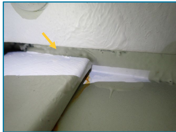
Photo 118 – 2"-3" tack welds on bottom moment plate and web plate (looking north on the inside of Pier Cap 11A).
