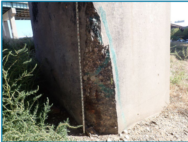
Photo 57 – Spall with exposed reinforcement at the northwest corner of Column 2 at Pier 24B (looking southeast).
