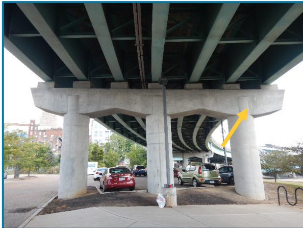
Photo 135 – Typical hairline cracks with minor efflorescence throughout the west face of Pier Cap 6 (FWW) (looking east).
