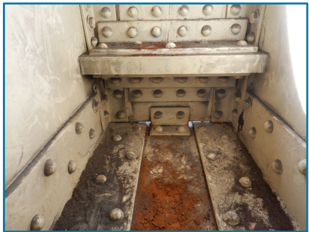
Photo 124 – Typical granular debris and dust throughout the bottom of the Pier Cap 13A interior (looking east near the west end of the cap).
