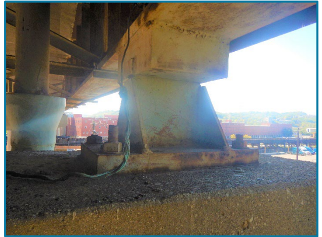
Photo 38 – Typical surface corrosion throughout fixed bearings (looking southwest at Girder A bearing at Pier 21B).
