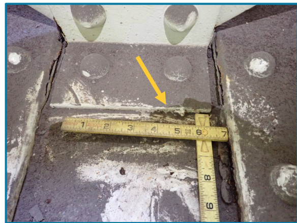
Photo 83 – 2" transverse tack weld between the bottom flange plate and the connection angle on the west side of Girder G diaphragm (looking east on the inside of Pier Cap 4A).
