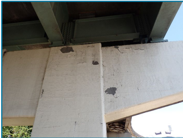
Photo 137 – Typical FRP wrapping with isolated areas of peeling/failing protective coating (looking north at the south face of Pier 23B).
