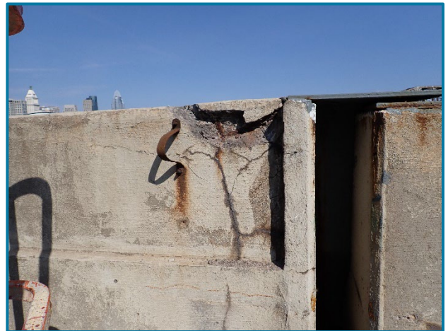
Photo 17 – Spall with exposed reinforcement at the top edge of the west railing at the River Pier (looking east).
