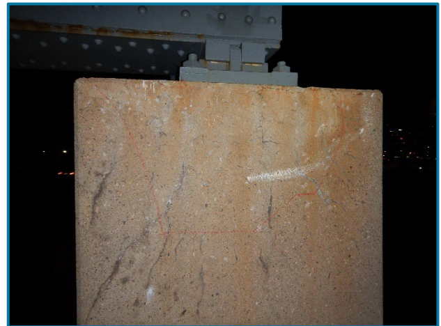
Photo 51 – Typical delamination and hairline cracking throughout the concrete column (looking north at Column 2 of Pier 8A).
