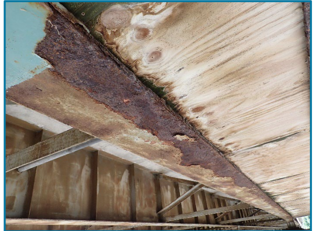
Photo 27 – Laminate corrosion with up to 1/8" deep section loss to the underside of the bottom flange of Girder A in Span 20A (looking southeast).
