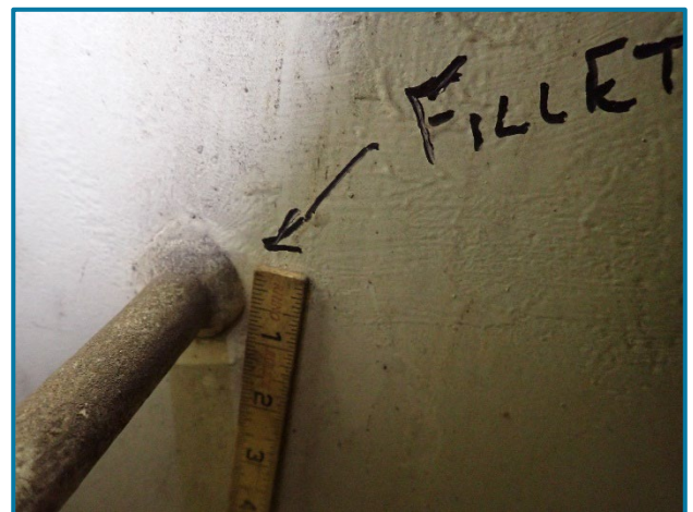
Photo 69 – Typical fillet weld at the ladder rungs on the interior of the north web plate of Pier 1A Cap (looking north).
