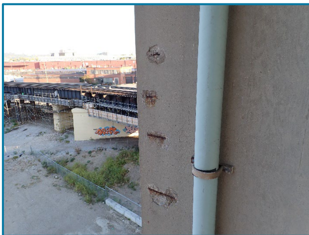
Photo 55 – Spalls with exposed reinforcement on the south face of Column 1 at Pier 17A (looking northwest).
