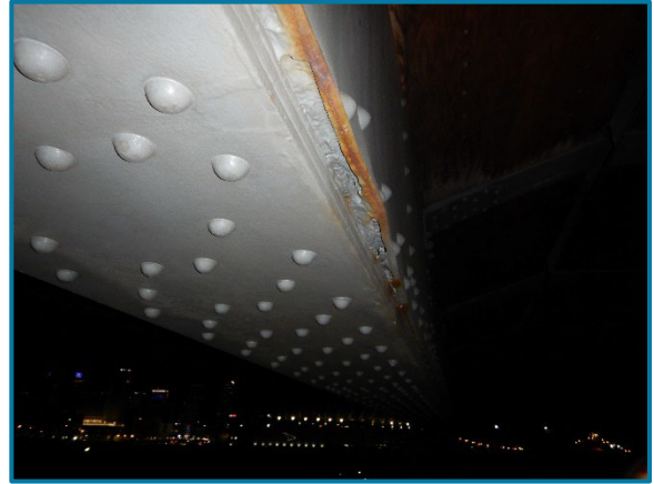
Photo 100 – Pack rust between the south web plate and south bottom flange angle (looking west below Girder C at the underside of Pier Cap 8A).
