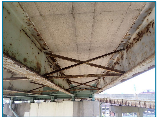
Photo 49 – Typical crossframes with minor surface corrosion in the original spans (looking south in Span 24B between Girders A and B).
