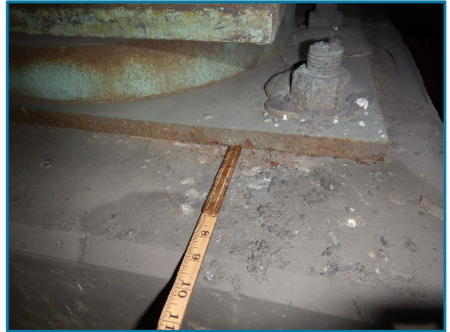
Photo 58 – Spall at the east bearing masonry plate of Pier Cap 29B (looking north).
