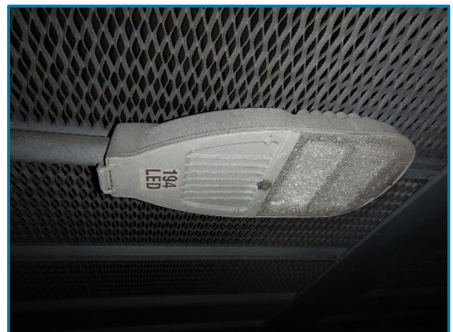
Photo 142 – Roadway light with shattered lens between Girders B and C at midspan in Span 11A (looking north).
