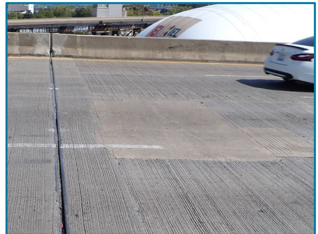
Photo 12 – Typical concrete patches near the expansion joint at Pier 8A (looking east).
