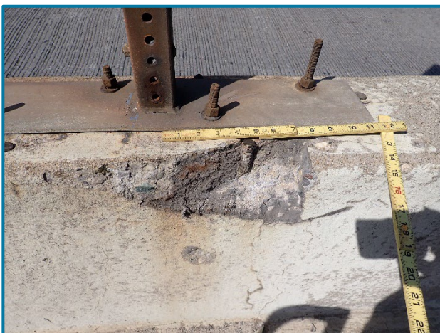
Photo 18 – Spall with exposed reinforcement at the top edge of the east railing at the base of a sign connection (looking west).
