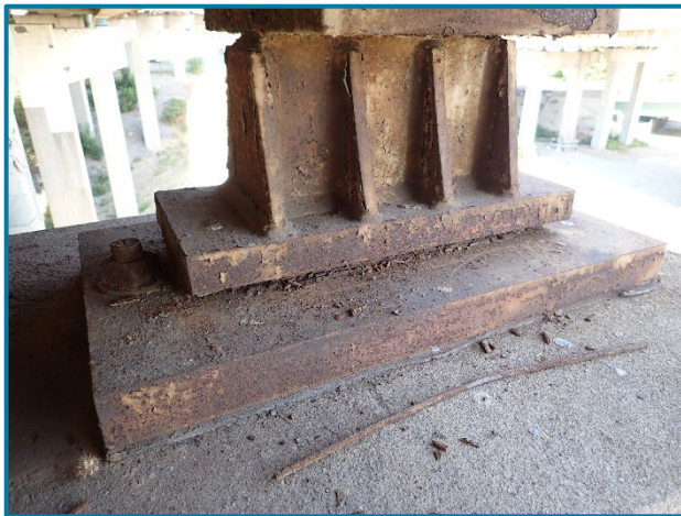
Photo 34 – 1/4" thick pack rust between the masonry plate and rocker bearing of Girder E at Pier 22B (looking north).
