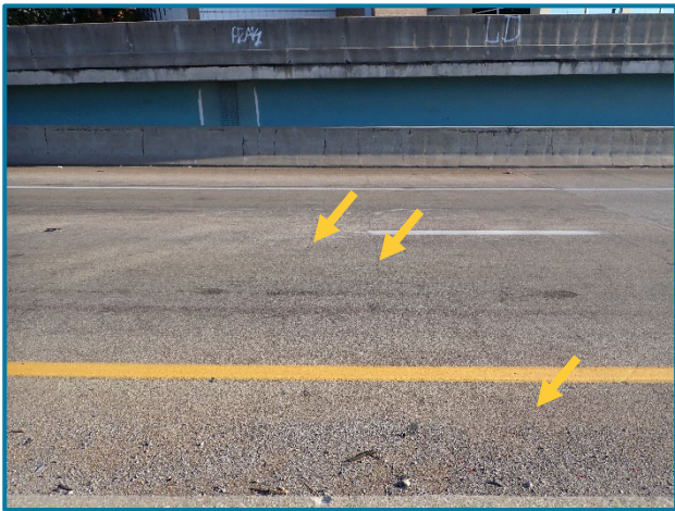
Photo 9 – Typical wearing surface with hairline transverse cracks throughout (looking northwest in Span 3 (FWW) at Pier 2 (FWW)).
