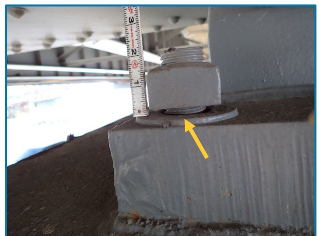
Photo 37 – Loose anchor bolt nut at the Girder B bearing of Pier 13A (looking southeast).
