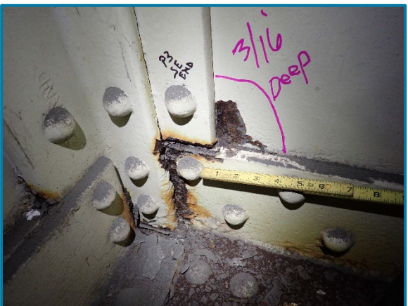
Photo 77 – 3/16" deep pitting in the south web plate and the south bottom flange angle at the east end of Pier Cap 3A (looking southeast).
