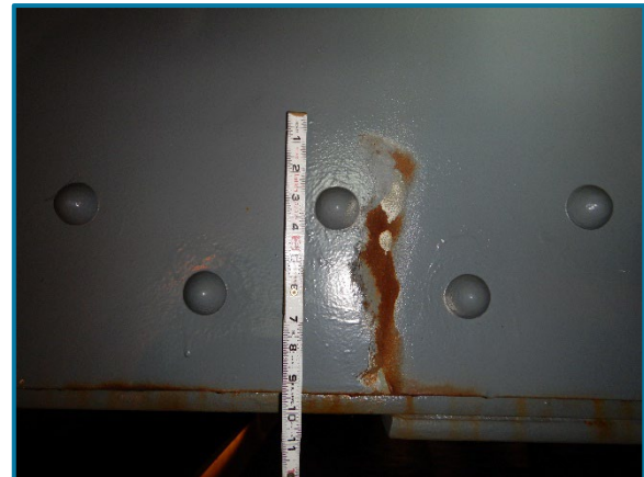
Photo 110 – Scrape on the north face of the north web plate of Pier Cap 10A east of the splice plate (looking south).
