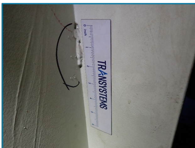
Photo 73 – Typical tack welds to interior transverse stiffeners inside of Pier Cap 2A (looking southeast).
