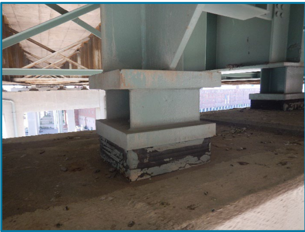
Photo 31 – Typical elastomeric bearing (looking southwest at the Girder D bearing at Pier 19A).
