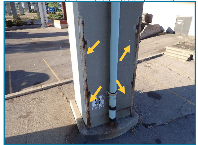
Photo 54 – Spalls at the corners of the existing protection brackets at Pier 16A (looking south at the north face of Column 1).
