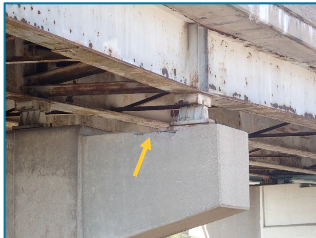
Photo 139 – 2' long by 1' wide by 3" deep spall extending onto the south face of Pier Cap 27B (looking north).
