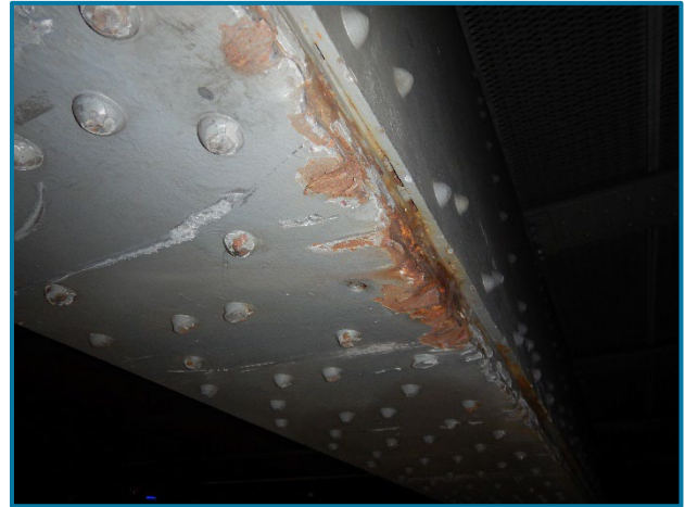
Photo 65 – Section loss at the base of the Girder C stiffening diaphragm at Pier Cap 1A (looking east).
