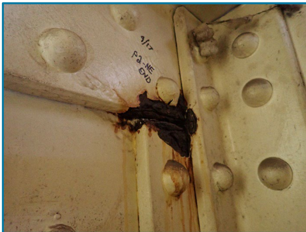
Photo 71 – Active laminate corrosion and section loss at the top corner of the north web plate, vertical angle, and top flange angle at the east end of Pier Cap 2A (looking northeast).
