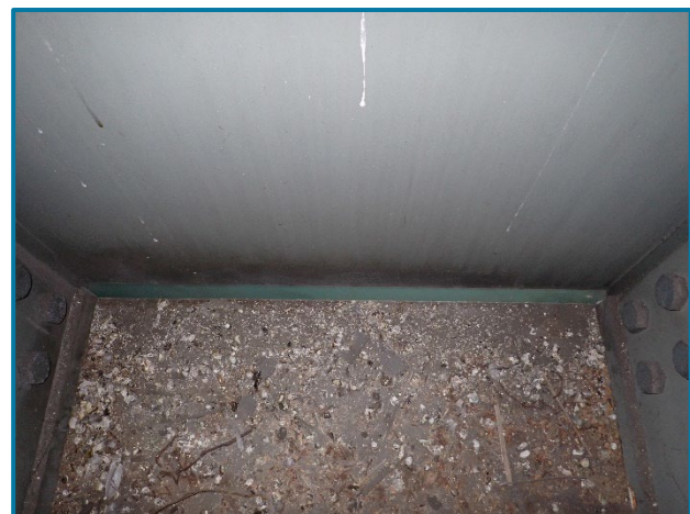
Photo 133 – Gap between bottom flange plate and web plate on the interior of Pier 2 (FWW) at the west end (looking west). Note the bird debris throughout the surface of the bottom flange plate.
