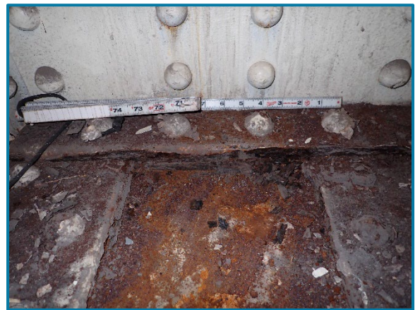
Photo 76 – Active corrosion along the bottom flange plate and bottom flange angle in the interior of Pier Cap 3A (looking east).
