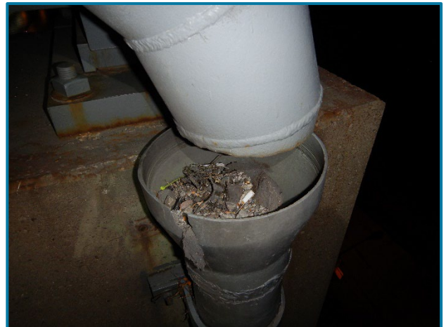
Photo 21 – Drainage bell clogged with debris at the west column on the north side of Pier 8A (looking southwest).
