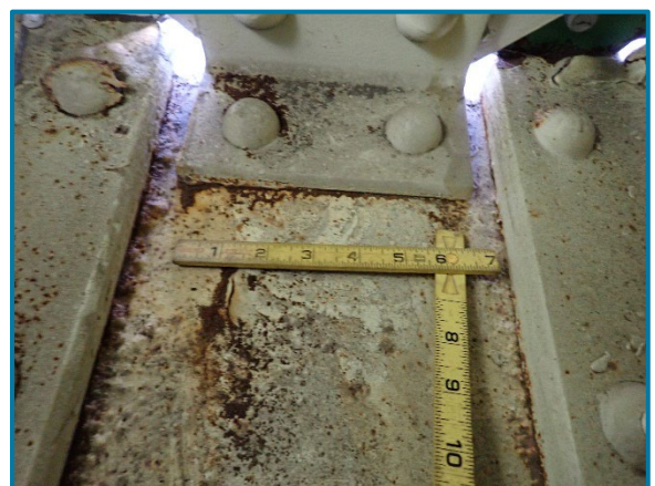
Photo 120 – Typical active corrosion and pitting throughout the bottom flange plate at the west end (looking west inside of Pier Cap 12A).
