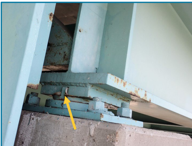
Photo 40 – Teflon pad extruded from the Girder 6 bearing at Pier 7 (looking southwest).
