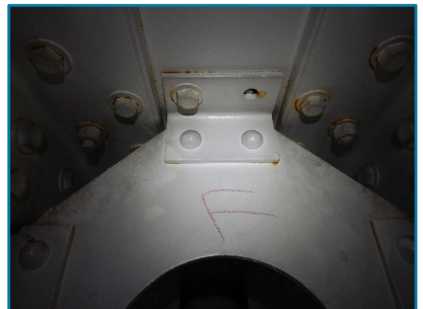
Photo 106 – Missing bolt in the east horizontal angle leg at the top flange connection of Girder F diaphragm (looking west on the inside of Pier Cap 9A).
