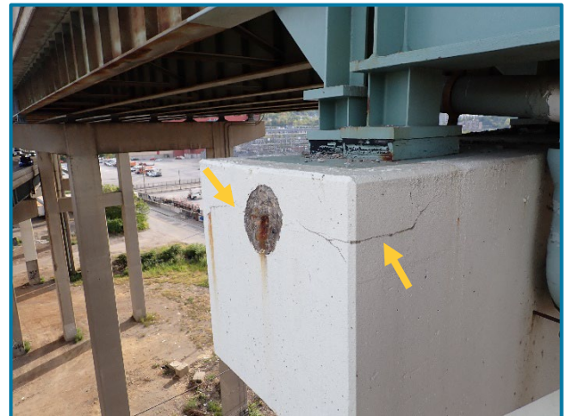
Photo 138 – 1' diameter by 1" deep spall on the east face of Pier Cap 15A (looking southwest). Note the longitudinal cracks extending from spall.
