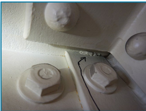
Photo 97 – Cracked tack weld between the north web plate and stiffening diaphragm of Girder A inside of Pier Cap 7A (looking northeast).
