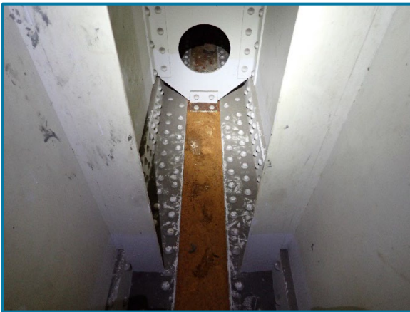
Photo 116 – Granular debris throughout the interior of Pier Cap 11A (looking west near east end).
