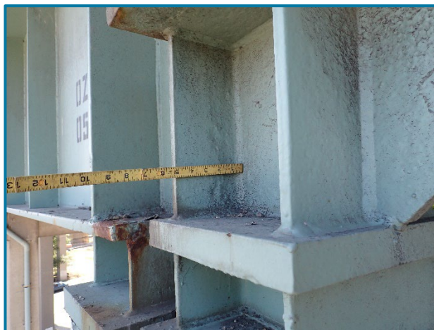
Photo 33 – Typical painted over pitting throughout the elastomeric bearing assembly (looking southwest at the Girder E bearing at Pier 23B). Note the corrosion on the south bearing.
