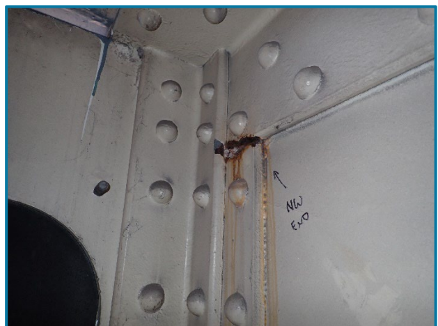
Photo 67 – Active corrosion along the interface between the north vertical web angle and top flange angle at the west end of Pier Cap 1A (looking northwest).
