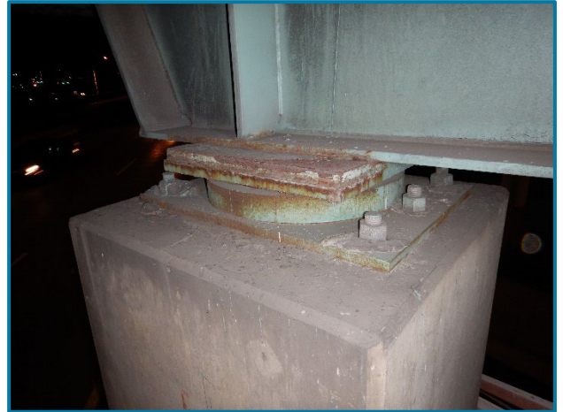
Photo 39 – Corrosion throughout the bearing at Girder 6 of Pier 29B (looking southeast).
