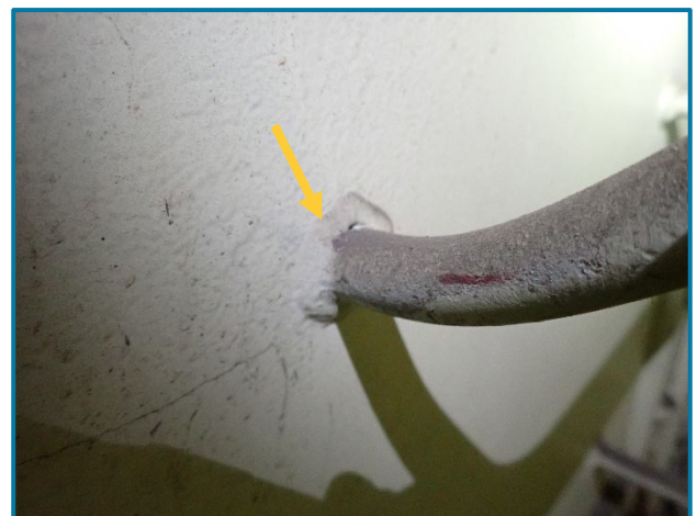
Photo 64 – Fillet weld at the ladder rung on the north web plate on the inside of the River Pier Cap (looking northeast).
