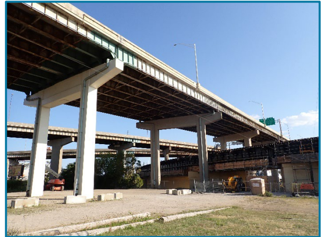
Photo 50 – Typical concrete piers in the original spans with FRP wrapping throughout (looking southeast at Piers 17A-19A).
