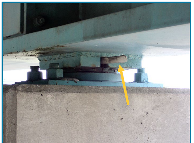
Photo 41 – Teflon pad extruded from the Girder 7 bearing at Pier 6 (looking northeast).
