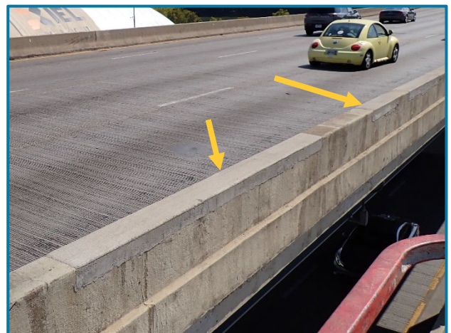
Photo 19 – Typical concrete patches at the top of the railing (looking southeast at the west railing in Span 7A).
