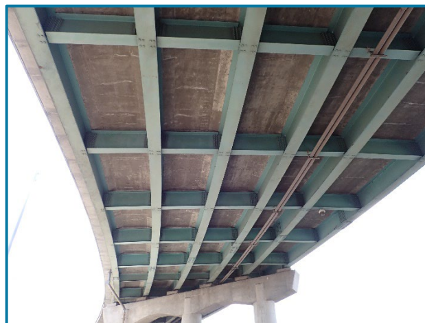
Photo 46 – Typical paint condition in the FWW spans (looking west in Span 8).
