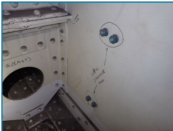
Photo 102 – Typical bolted drainpipe support bracket connection on the interior of the pier cap web (looking northwest near east end of Pier Cap 8A).
