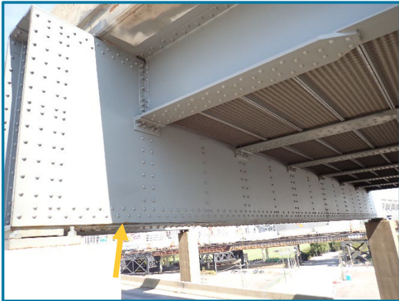
Photo 95 – Pack rust between the south web plate and the bottom flange angle with reactivating rust (looking northeast at the south face of Pier Cap 7A).
