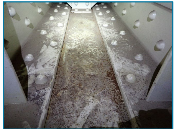
Photo 119 – Typical granular debris throughout the bottom of the interior of Pier Cap 12A (looking east near the west end of the cap).
