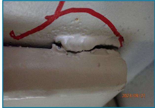
Photo 121 - Typical tack welds between the top angle and girder diaphragms (looking east near the top of Girder B inside of Pier Cap 12A).
