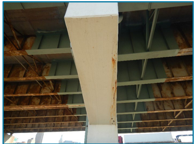
Photo 43 – End 10' of steel members at Pier 19A expansion joint painted during 2017 rehabilitation (looking east).
