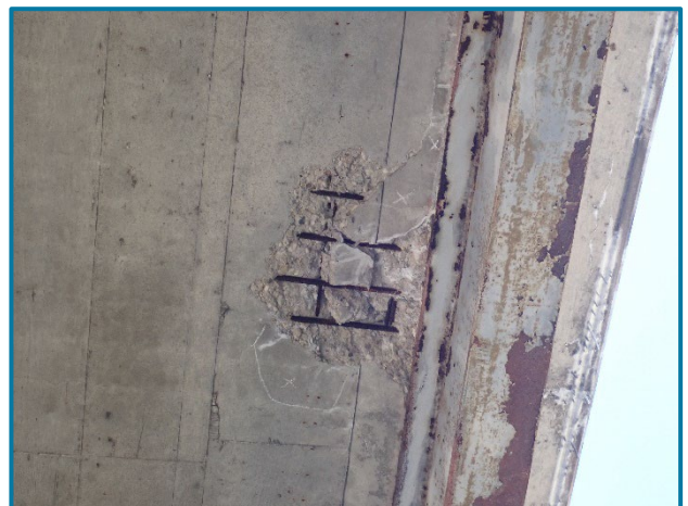
Photo 4 – Underside of deck spall between Girders D and E in Span 27B (looking up).
