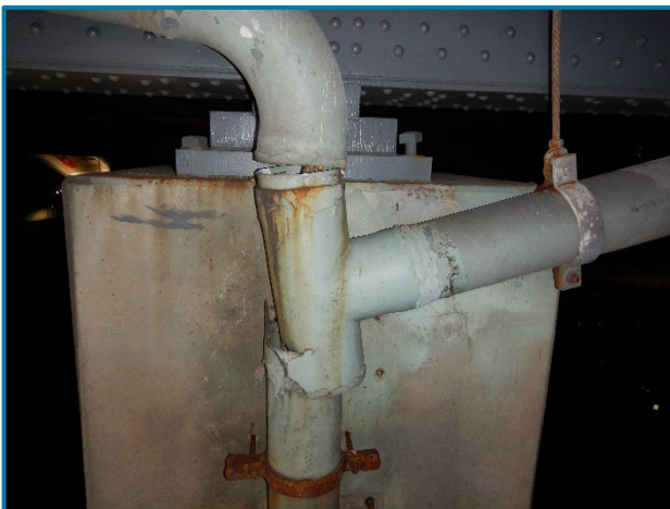
Photo 22 – Disconnected downspout T-joint on the north face of Column 1 at Pier 12A (looking south). Note the tearing of pipe.
