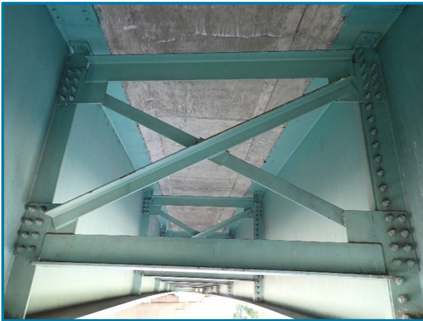
Photo 48 – Typical crossframe with minor surface corrosion in Span 5 (FWW) between Beams 9 and 10 (looking south).
