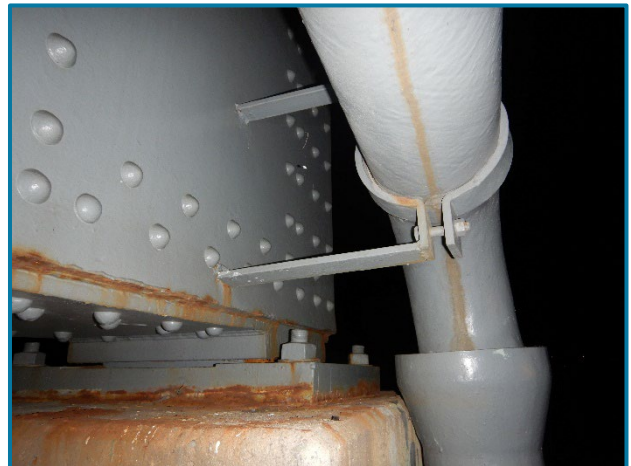
Photo 66 – Welded drainage support bracket on the north web near the west end of Pier Cap 1A (looking west).
