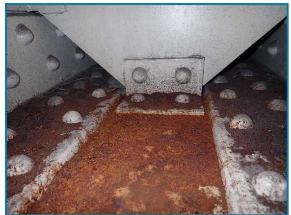
Photo 91 – Pier Cap 6A interior bottom flange plate just west of Girder A diaphragm (looking east).
