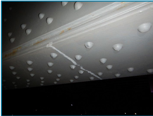
Photo 70 – Minor scrape/gouge on the underside of the bottom flange plate of Pier Cap 2A below Girder F (looking northwest).
