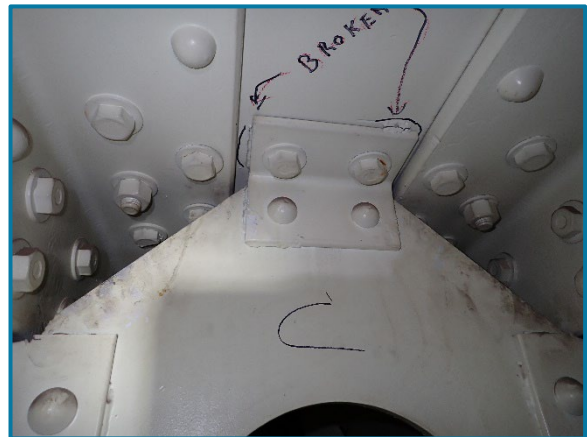
Photo 101 – Typical cracked tack welds along the Girder C diaphragm connection angle to top flange plate (looking east inside of Pier Cap 8A).
