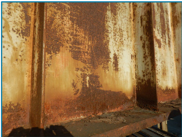
Photo 26 – Section loss throughout bottom flange and web on the east face of Girder H in Span 18A (looking northwest).
