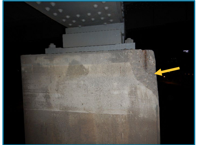
Photo 53 – Spall with exposed reinforcement at the top northeast corner of Column 2 at Pier 11A (looking north).
