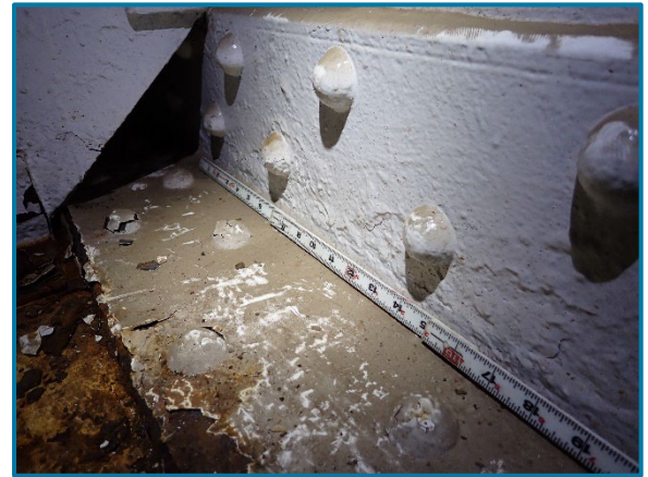
Photo 112 – Painted over pitting along the bottom flange connection angle and bottom flange plate of Pier Cap 10A (looking southeast near midspan).
