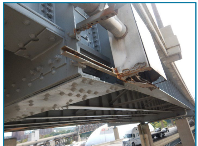
Photo 141 – 100% section loss throughout the utility junction box at the west access hatch at Pier 13A (looking southeast).
