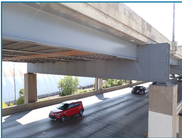
Photo 42 – Typical protective coating system condition in Spans 1A-14A (looking southeast towards Pier Cap 5A).
