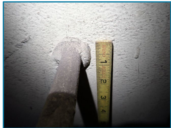
Photo 79 – Typical fillet weld at the ladder rungs on the interior of the north web plate at the east end of Pier 3A (looking north).
