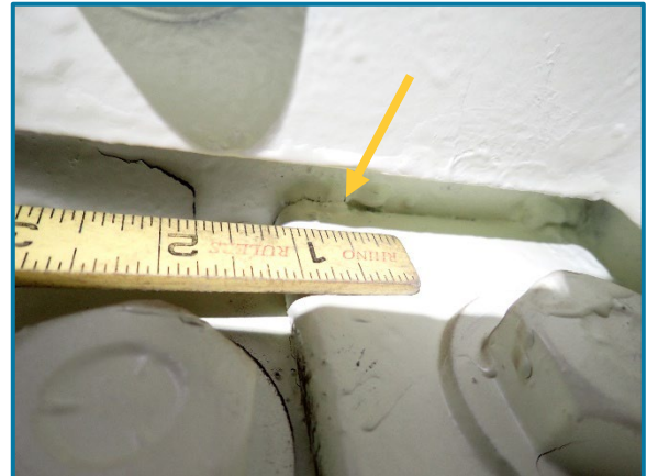
Photo 87 – Cracked tack weld between Girder E bottom flange and diaphragm connection angle (looking southwest at the south web plate of Pier Cap 5A).
