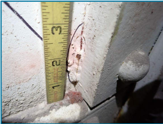
Photo 108 – Cracked tack weld between the east edge of the west bearing diaphragm fill plate and south web plate (looking southwest inside of Pier Cap 9A).
