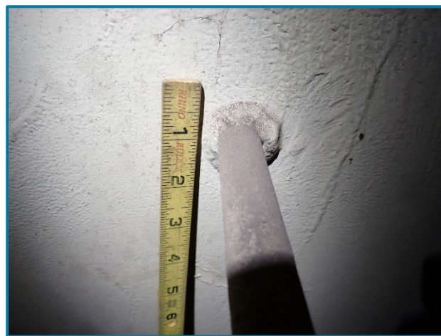
Photo 74 – Typical fillet weld at the ladder rungs on the interior of the north web plate of Pier 2A Cap (looking north).
