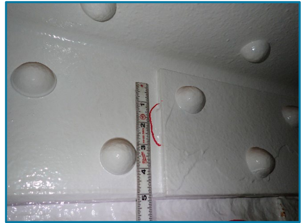
Photo 114 – Typical tack weld at the interface between the splice plates and the interior flange angles (looking northwest on the inside of Pier Cap 10A).
