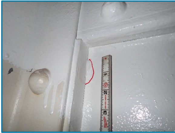
Photo 113 – Typical tack weld along the north web plate and transverse stiffener angle of Pier Cap 10A (looking south between Girder G and F).
