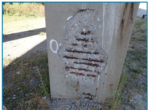
Photo 56 – Spall with exposed reinforcement on the south face of Column 2 at Pier 23B (looking north at the base).
