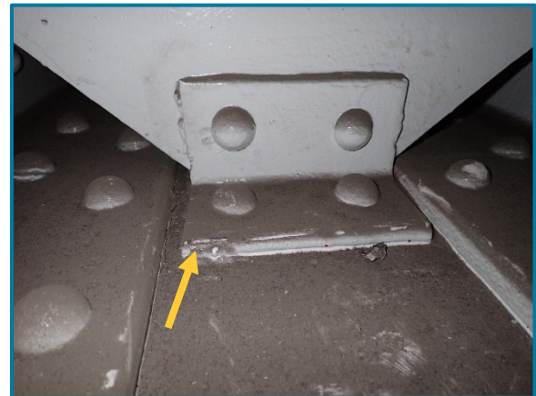
Photo 103 – Tack welds between the bottom plate and east connection angle of the Girder diaphragms (looking west inside of Pier Cap 8A).
