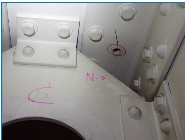
Photo 125 – Missing bolt at the connection between the north top flange angle and north web plate at Girder C (looking west inside of Pier Cap 13A).
