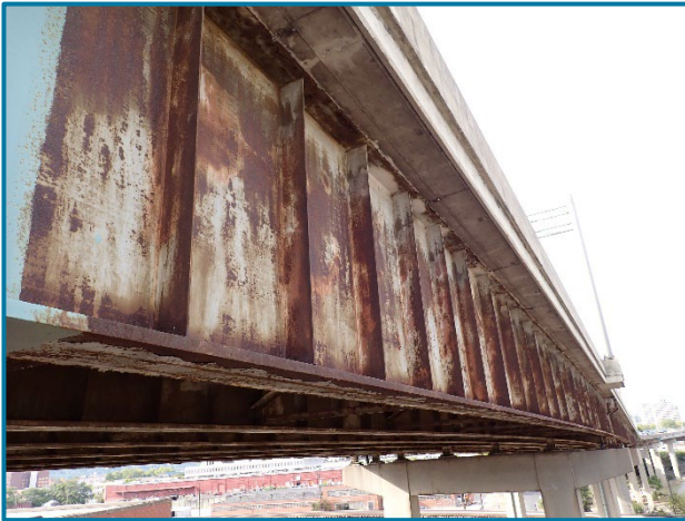
Photo 44 – Typical surface corrosion throughout Spans 15A-28B (looking northwest at Girder H in Span 16A).
