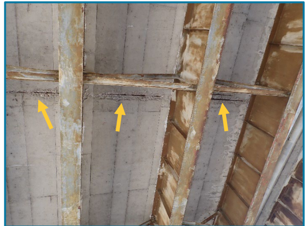
Photo 2 – Full width underside of deck spall at midspan of Span 21B (looking up and south).
