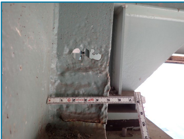
Photo 29 – Painted over corrosion hole in the web behind the bearing stiffener of Girder D at Pier 19B (looking west).
