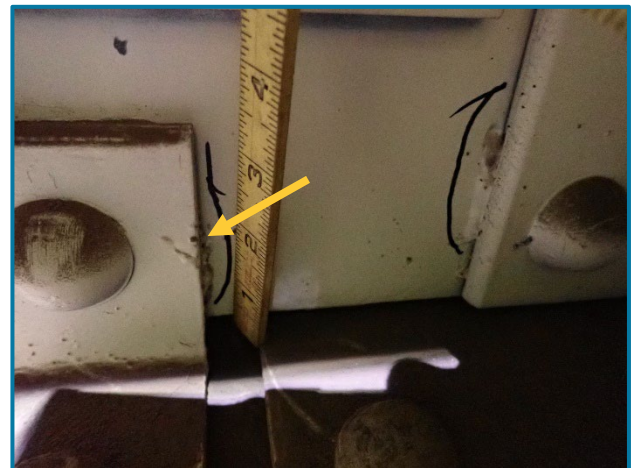
Photo 127 – Tack welds between the top and bottom angles and girder diaphragms (looking west inside of Pier Cap 13A).
