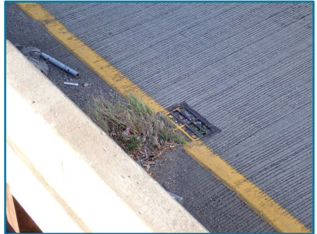
Photo 20 – Typical clogged scupper (looking south in Span 17A near Pier 16A).
