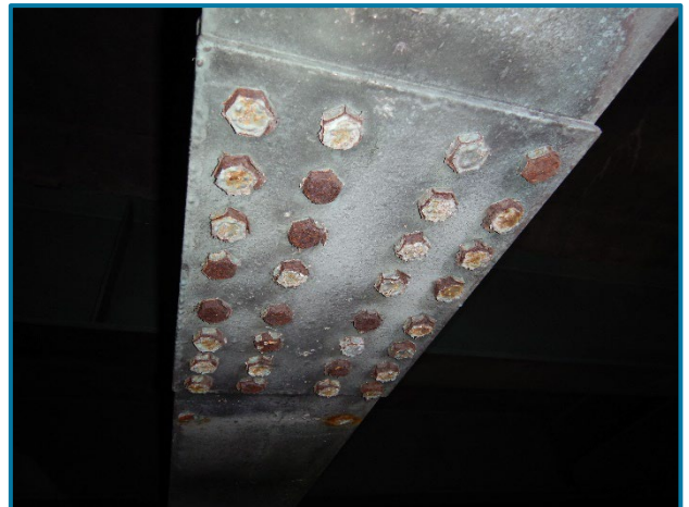
Photo 130 – Surface corrosion throughout the bolts in the bottom flange splice plate of Pier 29B (looking east).
