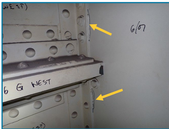
Photo 93 – Two 3" tack welds between the south web plate and connection angles on west side of Girder C (looking southeast inside of Pier Cap 6A).
