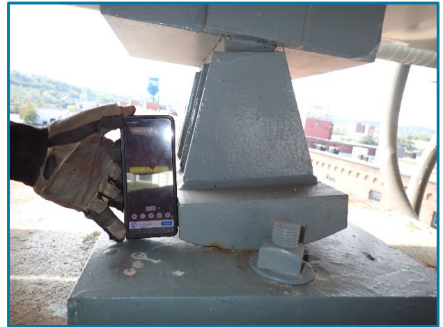
Photo 35 – Girder A bearing at Pier 14A contracted 7° to the south at Pier 14A (looking west).
