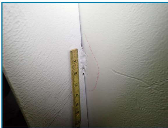
Photo 82 – Typical tack welds to transverse stiffeners and web plates on the interior of Pier Cap 4A (looking southeast).
