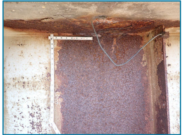
Photo 45 – Typical failed paint on the exterior face of the fascia girder with areas of measurable section loss (looking east at the west face of Girder A in Span 23B).
