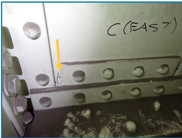
Photo 126 – Tack weld between the diaphragm fill plate and diaphragm plate at Girder C (looking west inside of Pier Cap 13A).
