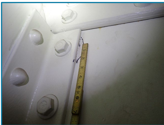
Photo 98 – Typical tack welds between the south web plate and the connection angle on each side of every girder diaphragm (looking south on the inside of Pier Cap 7A).
