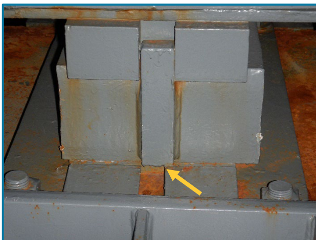
Photo 36 – Misaligned bearing at the east end of Pier Cap 11A (looking north).
