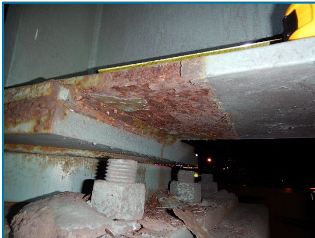
Photo 129 – Active rust with peeling paint on the Pier 29B bottom flange at the north bearing (looking northeast).
