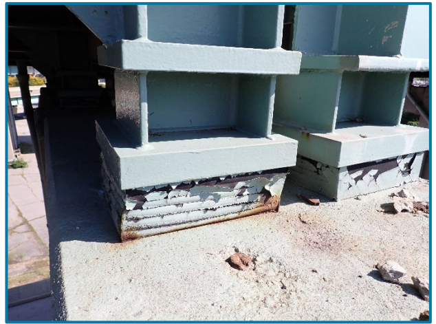
Photo 32 – Bearing pads expanded beneath Girder A in Spans 23B and 24B at Pier 23B (Looking east).
