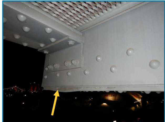
Photo 123 – Pack rust between the bottom flange plate and north bottom angle below Girder G at Pier Cap 13A (looking southeast).
