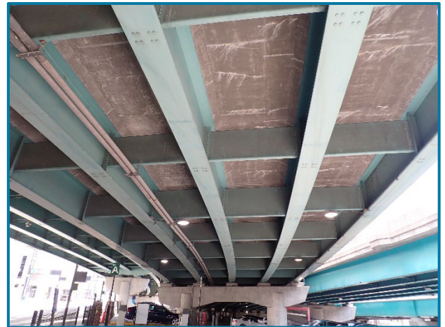
Photo 1 – Typical underside of deck with transverse cracking and efflorescence throughout (looking northeast in Span 2 (FWW)).
