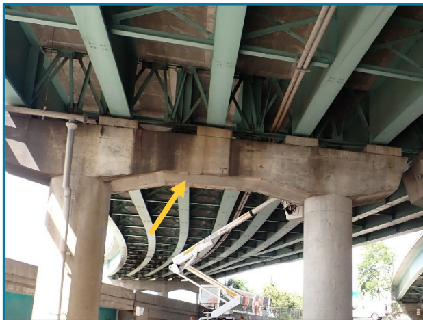
Photo 136 – Flexural cracks between the pier columns at Pier 4 (FWW) (looking west).
