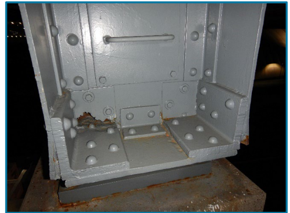
Photo 105 – 100% section loss at the bottom of the west end vertical access plate (looking east at Pier Cap 9A).
