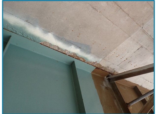
Photo 5 – Typical haunch spalls along the top flange of Girder A in Span 20B (looking northwest).
