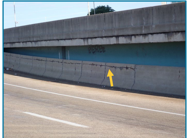
Photo 16 – Typical longitudinal cracking on the interior face of the concrete railing (looking northwest in Span 3 (FWW)).
