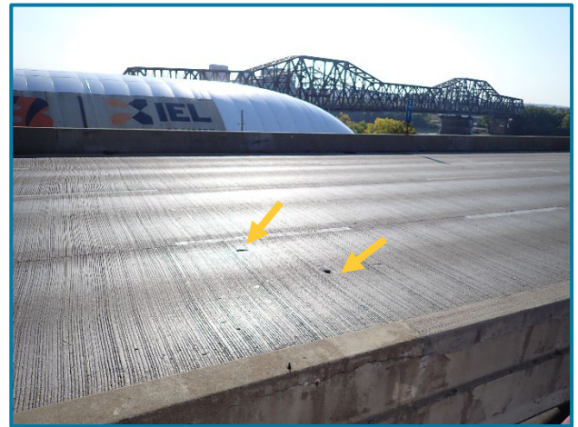
Photo 10 – Typical shallow pop-out spalls in the wearing surface in Span 3A (looking east).
