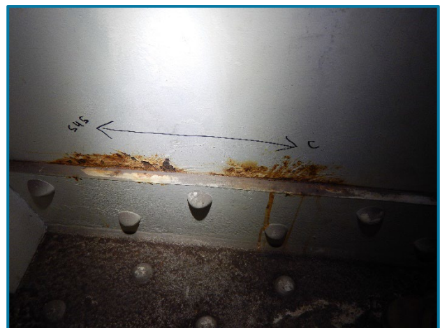
Photo 62 – Active corrosion along the bottom flange angle at the north web plate between Girders C and D inside the River Pier Cap (looking north).
