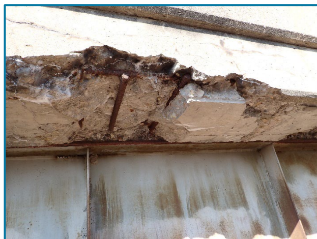
Photo 7 – East overhang spall with exposed reinforcement near Pier 19A in Span 20B (looking west).
