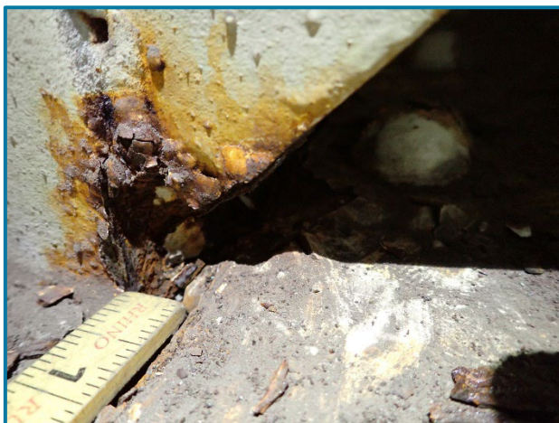
Photo 72 – Section loss at the base of the Girder G stiffening diaphragm on the interior of Pier Cap 2A (looking east).
