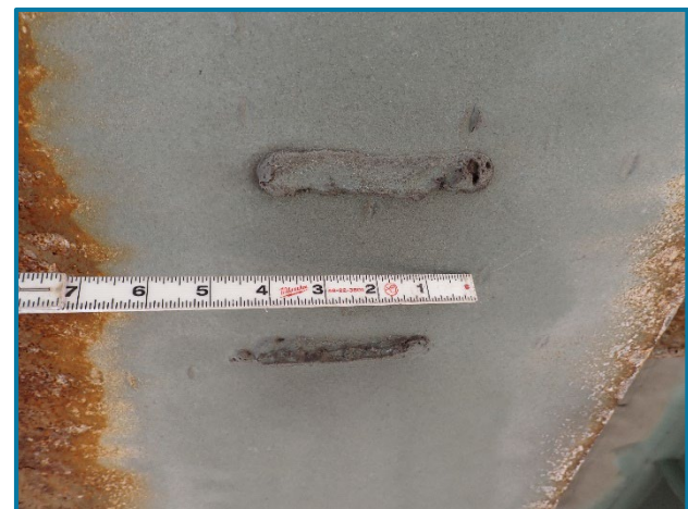
Photo 30 – Fatigue-prone welds on the underside of the girder bottom flange in Span 15A (looking south at Girder F).
