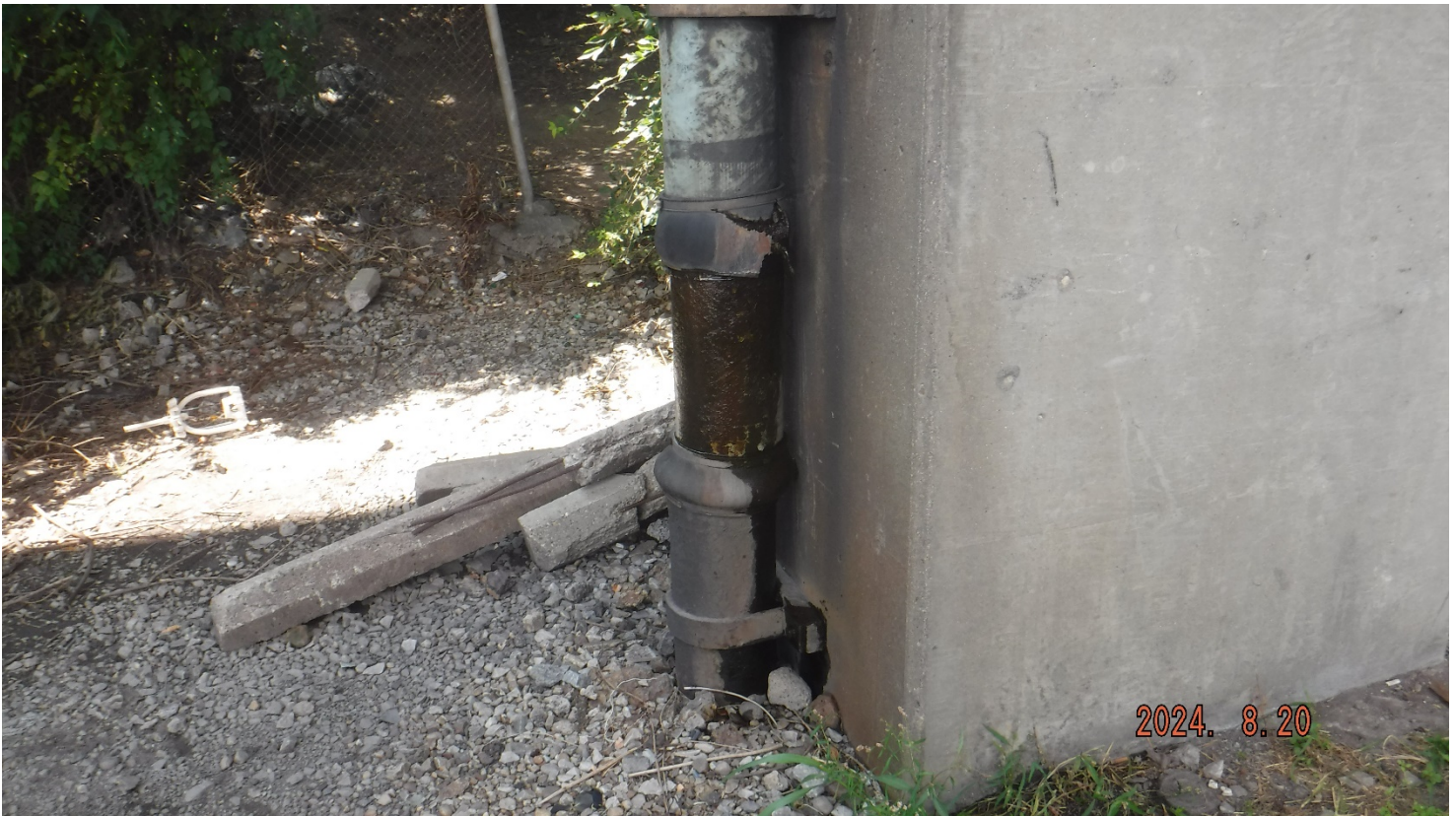
PHOTO 4. DRAINAGE PIER 23A COLUMN 1, CRACKED AND LEAKING GASKET IN THE DRAINAGE PIPE
