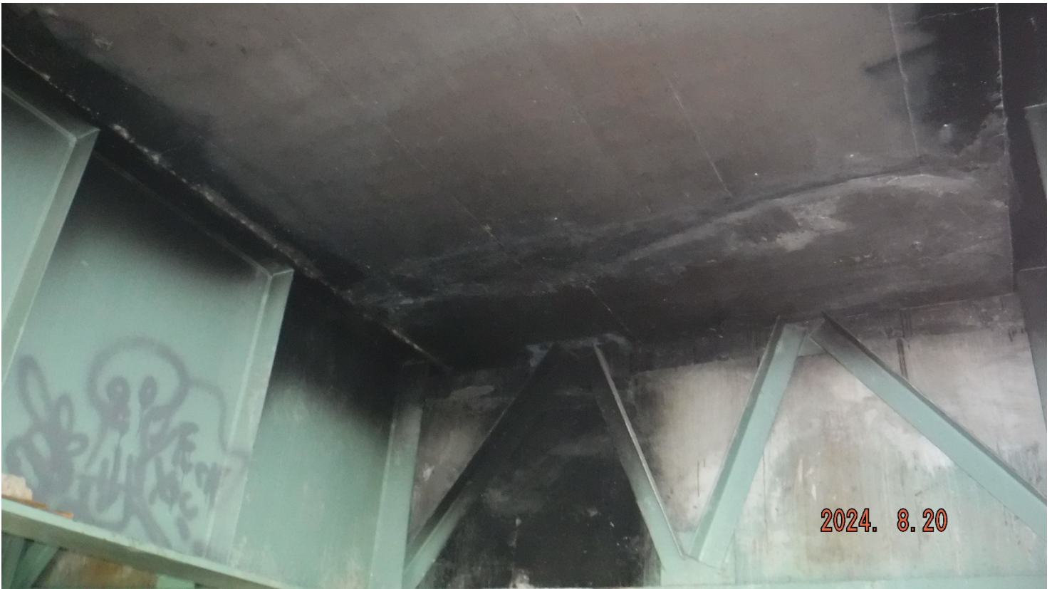
PHOTO 10. BACKWALL BAY 3, FIRE DAMAGE WITH HAIRLINE CRACKING THROUGHOUT BACKWALL
