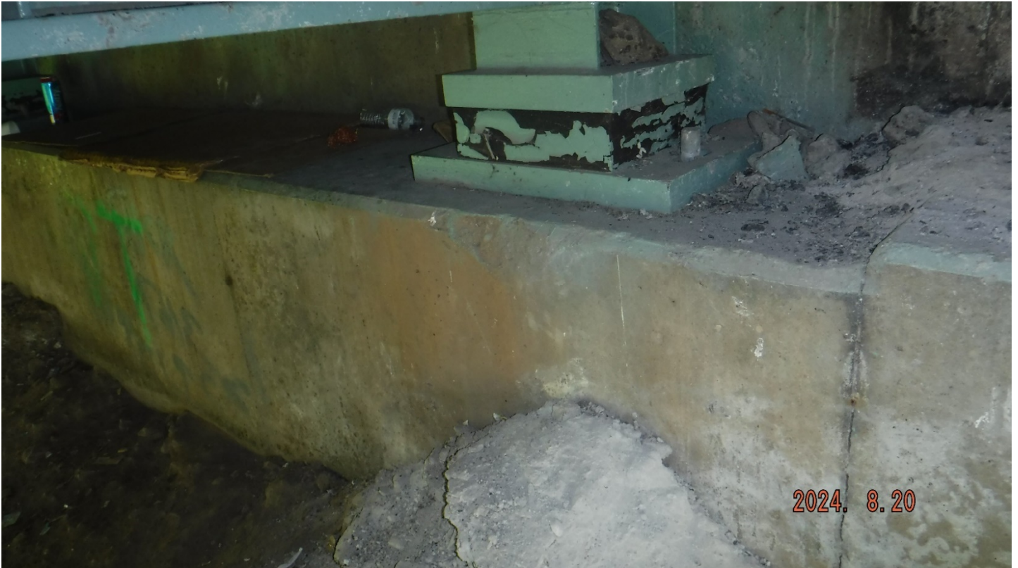
PHOTO 7. ELASTOMERIC BEARING C ABUTMENT, 12" L X 6" W X 1" DEEP SPALL BELOW BEARING GIRDER C
