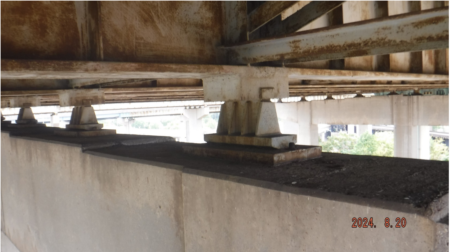
PHOTO 9. MOVABLE BEARING B PIER 21A MOVABLE, MISSING NUT ON BOLT
