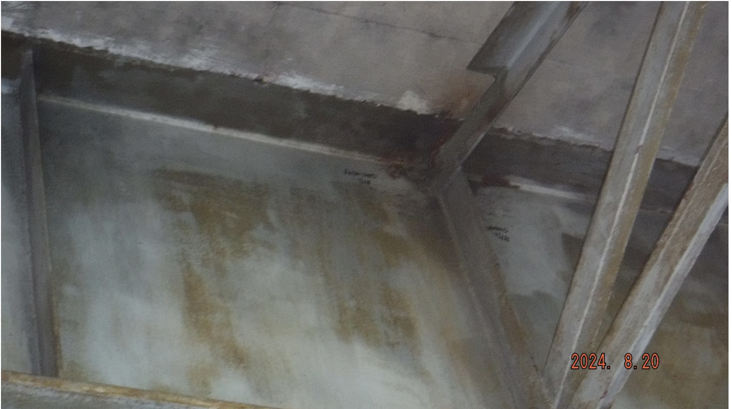
PHOTO 6. GIRDER 25A GIRDER C, MULTIPLE CRACKS IN WEB AND TRANSVERSE STIFFENER WELDS. ALL CRACKS REPAIRED WITH ARREST HOLES AND NO INDICATION OF CONTINUED PROPAGATION
