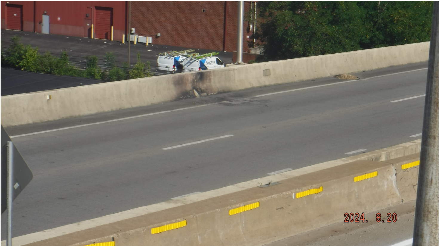
PHOTO 3. WEARING SURFACE SPAN 21, FIRE DAMAGE OR CHEMICAL IN RIGHT LANE SHOULDER
