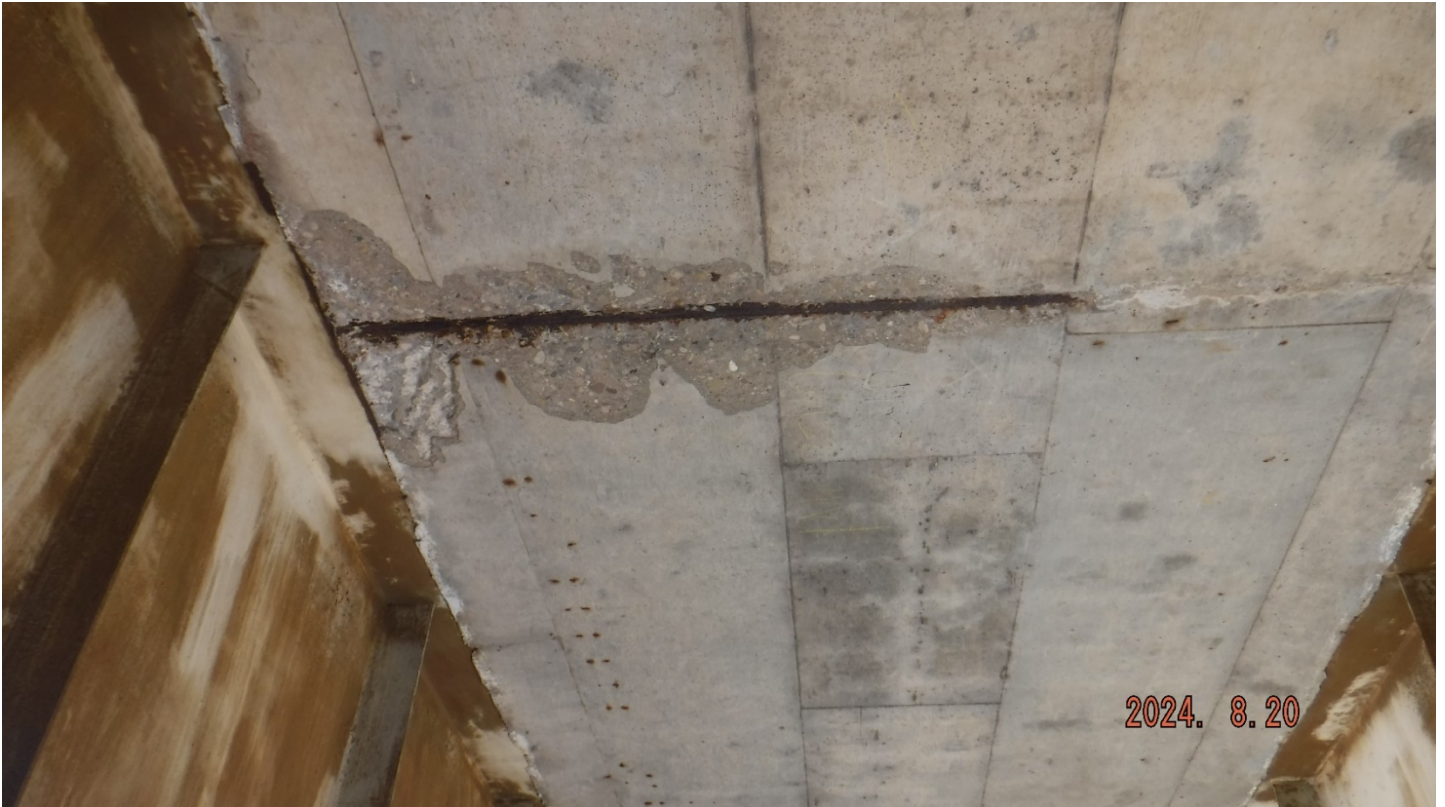
PHOTO 1. DECK SPAN 21 BAY 1, 2SQFT SPALL WITH EXPOSED REINFORCEMENT AT 2 LOCATIONS
