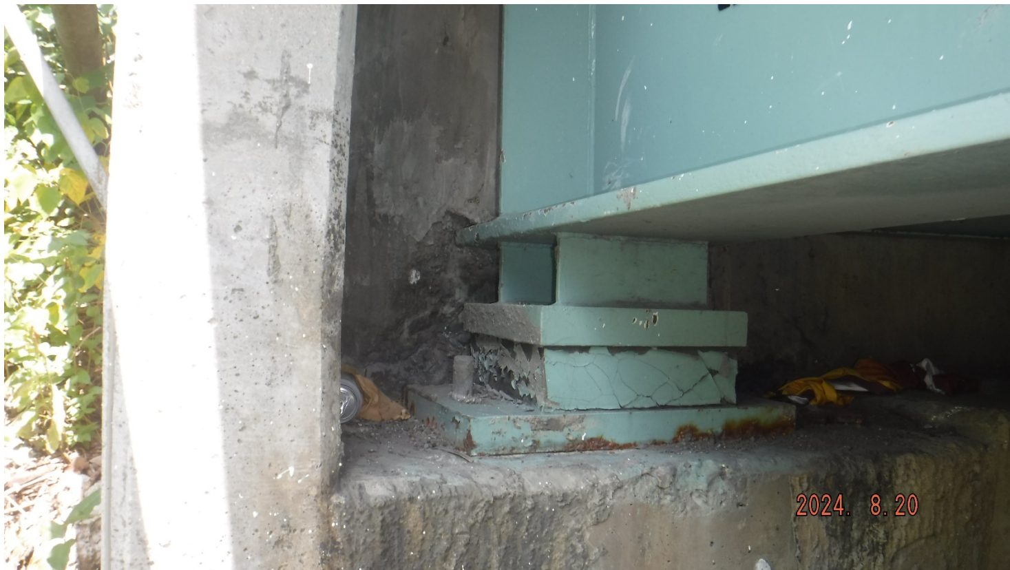
PHOTO 11. BACKWALL GIRDER A, 2" DIAMETER X 1' DEEP SPALL BEHIND BEARING
