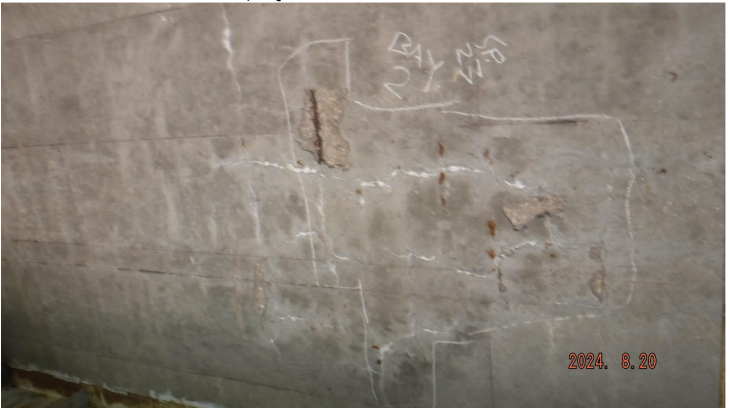
PHOTO 2. DECK SPAN 23A BAY 2, 8'LX8'WX1" DEEP AREA OF DELAMINATION AND 2' SPALL WITH EXPOSED REINFORCEMENT
