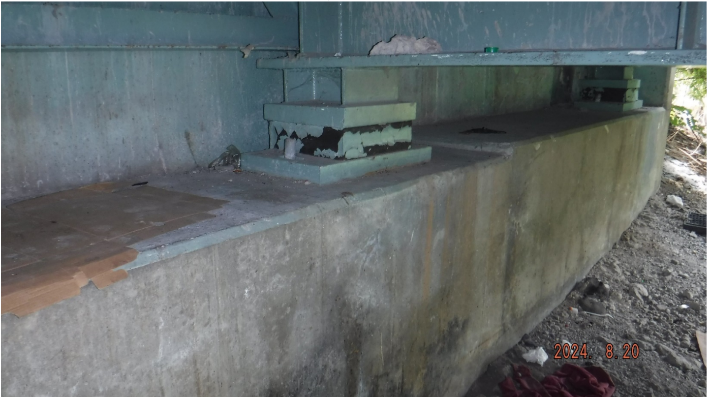
PHOTO 8. ELASTOMERIC BEARING D ABUTMENT, 4" L X 2" W X 1" DEEP SPALL BELOW THE BEARING OF GIRDER D
