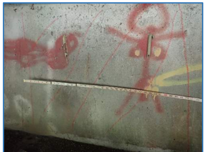
Photo 88 - Delaminated area along backwall of forward abutment
