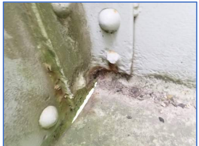
Photo 53 - Up to 50% section loss in rivet heads in Span 3, Floorbeam 4, gusset plate clip angle connection, south end, looking west
