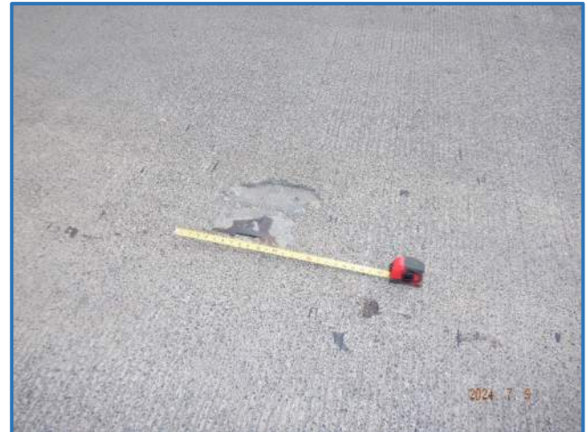
Photo 6 - Spall in Span 1, east side of span
