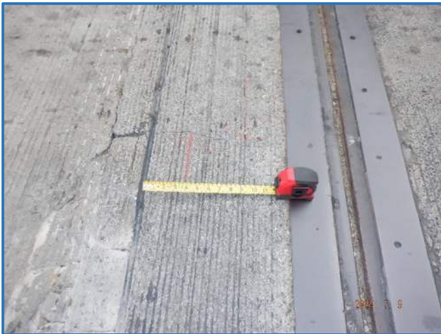
Photo 90 - Longitudinal crack in top of header of rear abutment, looking north
