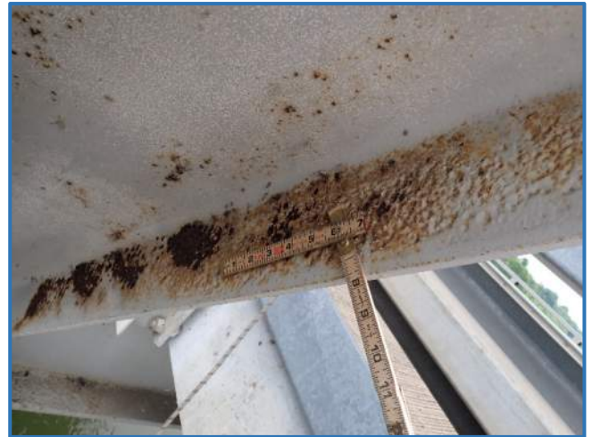
Photo 43 - Pitting on interior of flange in Span 1, South Truss, member L5U6, looking northwest
