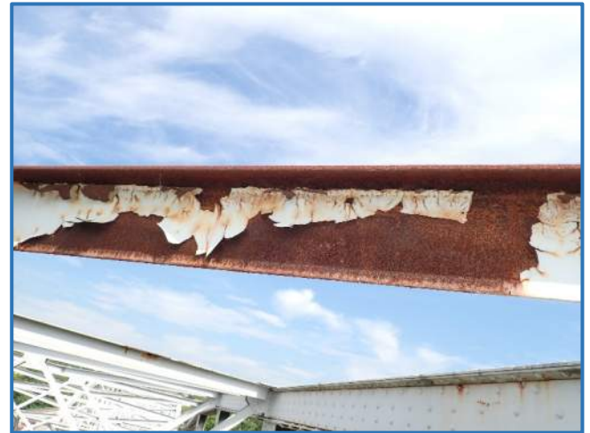
Photo 70 - Paint failure with surface corrosion on upper lateral brace in Span 3, between Panel Points 5 and 6, looking northwest
