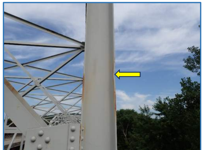
Photo 41 - Impact damage to north flange in Span 3, North Truss, at Panel Point 6, looking west
