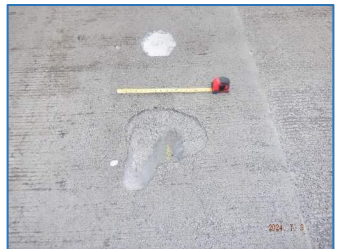
Photo 5 - Spalls in wearing surface on Span 3, left lane, between Panel Points 2 and 3
