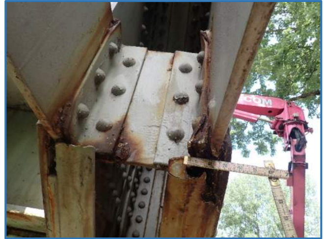
Photo 17 - Bowing in lower chord northeast diaphragm angle due to pack rust, 1 1/2" over 4", Span 4, North Truss, member L0L1
