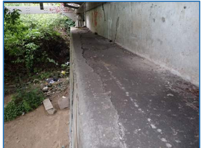
Photo 87 - Bearing seat of rear abutment with delaminations, looking south
