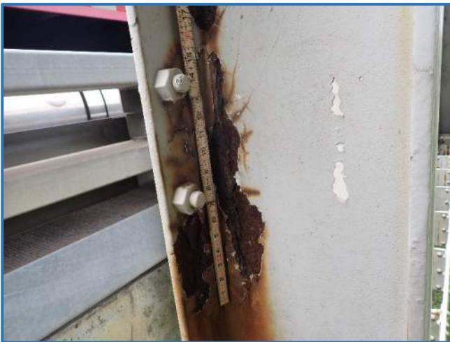
Photo 39 - Laminar corrosion on flange and web of vertical member in Span 3, North Truss, at Panel Point 9, looking west
