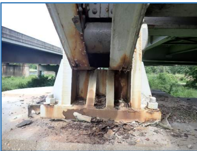
Photo 59 - Typical corrosion and section loss on bearings. Shown is Span 3, movable bearing on Pier 4, looking east
