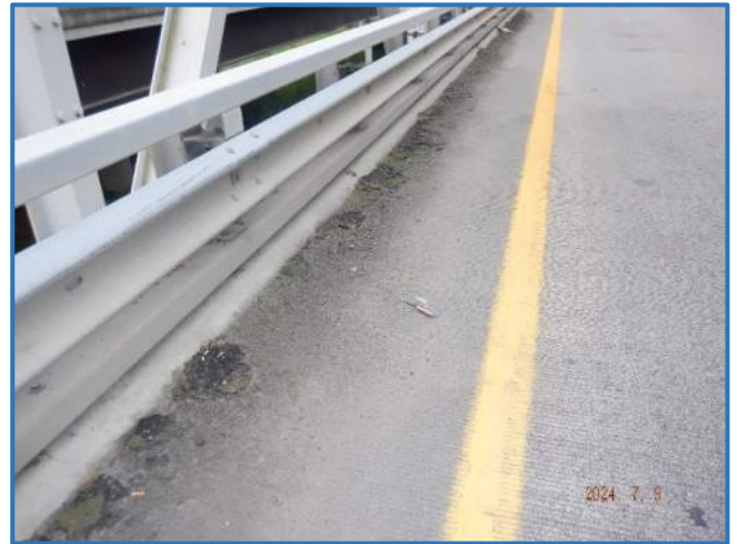
Photo 11 - Typical debris accumulation along edge of bridge deck, shown Span 4, south lane
