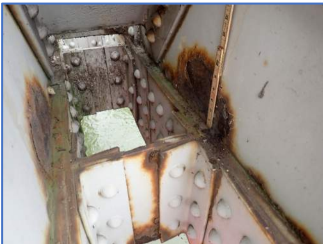
Photo 55 - Laminar corrosion with section loss on interior lower gusset plate. Span 2, North Truss, Panel Point 6, 3" long by 3" wide by 1/8" deep, looking west
