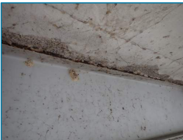
Photo 12 - Typical haunch spalling along outside stringers with surface corrosion along top flange. Shown Span 2, Stringer 1, looking northeast
