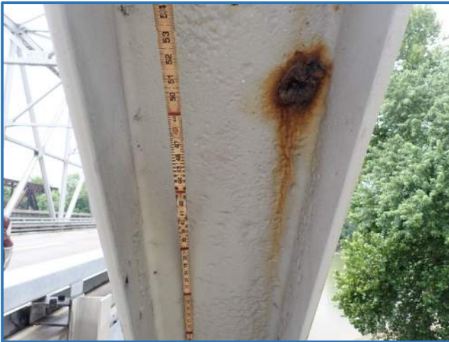
Photo 42 - Pitting on underside of web in Span 2, North Truss, member L8U9, looking west
