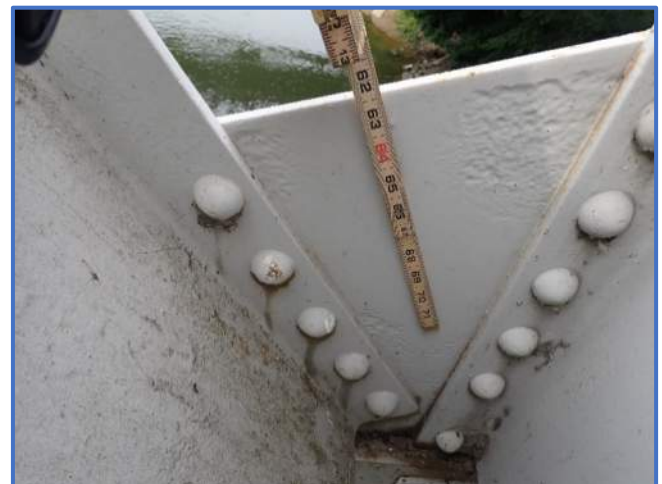
Photo 56 - Typical coated pitting on interior gusset plate. Shown Span 1, South Truss, at Panel Point 4, looking south
