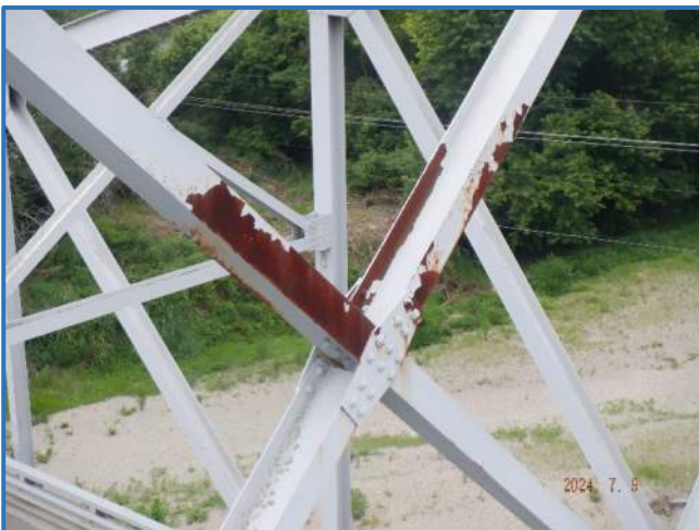
Photo 72 - Surface corrosion on diagonal sway braces in Span 3, at Panel Point 3, looking west
