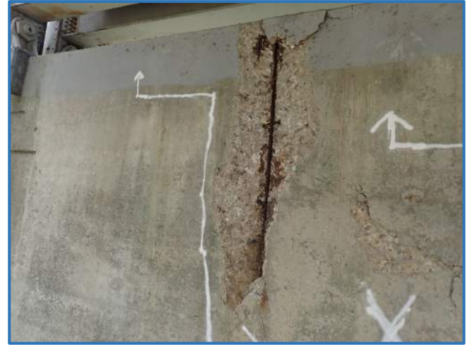
Photo 78 - Spall in west face of Pier 3 under Stringer 2, with exposed rebar with section loss
