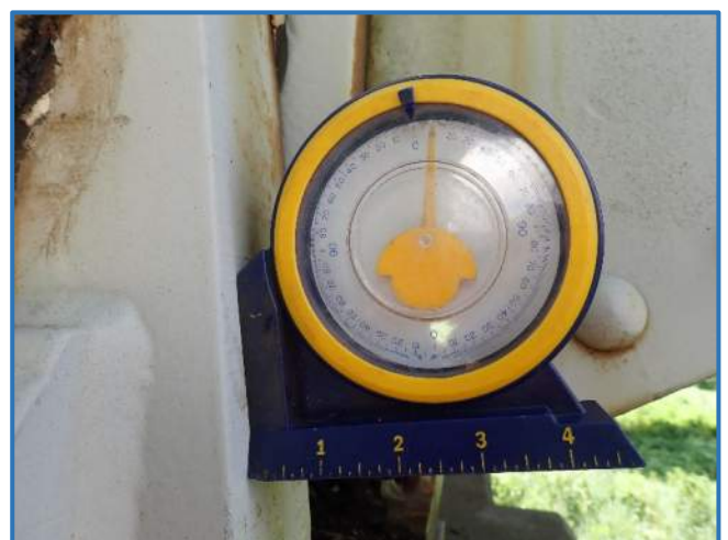
Photo 60 - 9-degree tilt of bearing in Span 3, north bearing on Pier 4, looking south
