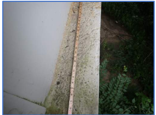
Photo 46 - Typical pitting on top face of bottom flange. Shown is 3.5' long by 1/16" deep pitting on Floorbeam 1, south end, Span 1, looking north
