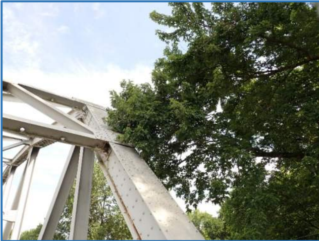
Photo 95 - Tree encroaching on end post in Span 3, North Truss, between Panel Points 9 and 10, looking northwest
