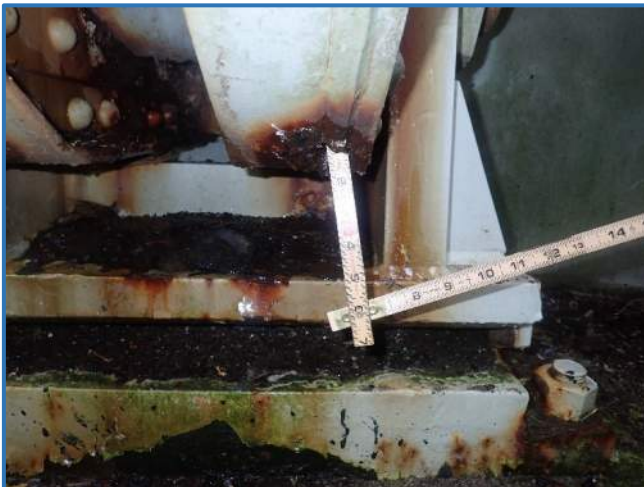
Photo 22 - Up to 100% section loss on the lower chord stiffener, Span 4, North Truss, at L8, looking east
