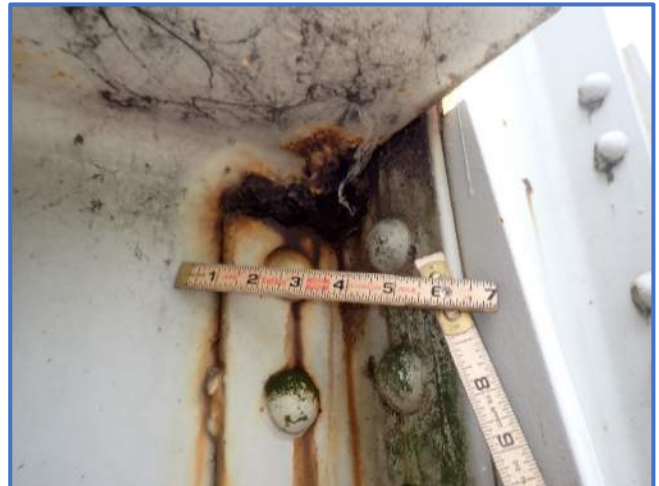
Photo 54 – Corrosion along top flange and clip angle in Span 2, Floorbeam 9 west face, north end, looking west. Note tack weld at clip angle to floorbeam web connection.
