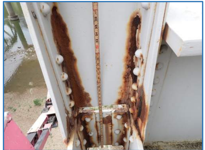
Photo 40 - Active corrosion with section loss along flanges and web of vertical member in Span 2, South Truss, at Panel Point 9, looking west
