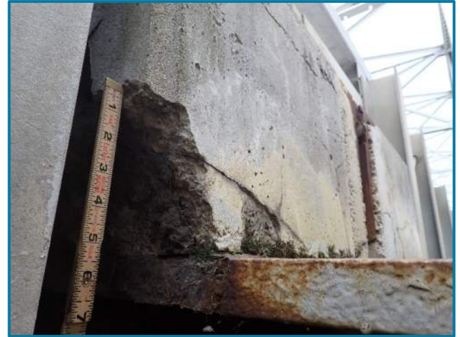
Photo 3 - 6" by 6" by 6" spall on edge of deck on north end, above FBO, in Span 3
