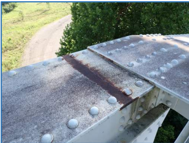
Photo 27 - 6" long by 4" wide paint failure in Span 4, North Truss, member U5U6, looking northeast
