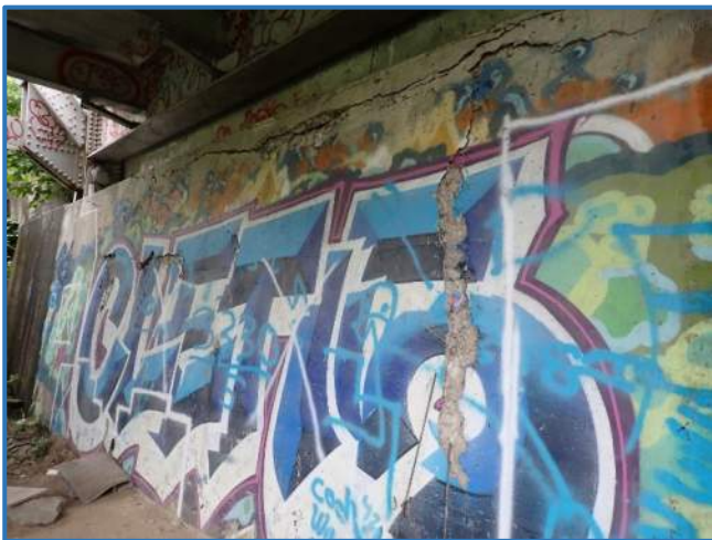
Photo 86 - Rear abutment with cracking and delaminations
