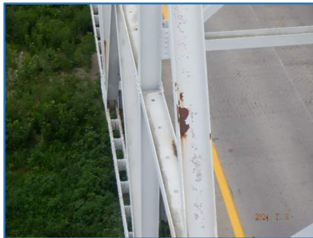
Photo 44 - Paint failure with active corrosion on web of diagonal in Span 3, South Truss, member U5L6, looking west
