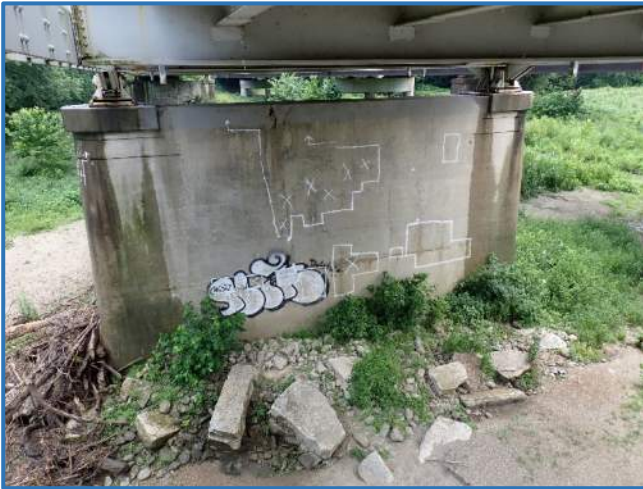
Photo 77 - Large delaminated area at the top of west face of Pier 3
