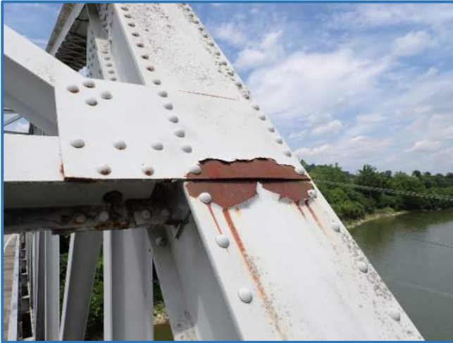
Photo 35 - Paint failure with surface corrosion on top face of end post in Span 1, North Truss, between Panel Points 7 and 8, looking west
