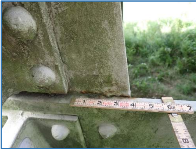
Photo 20 - Broken tack weld between lower chord and gusset plates, Span 4, North Truss, at Panel Point 1, looking south
