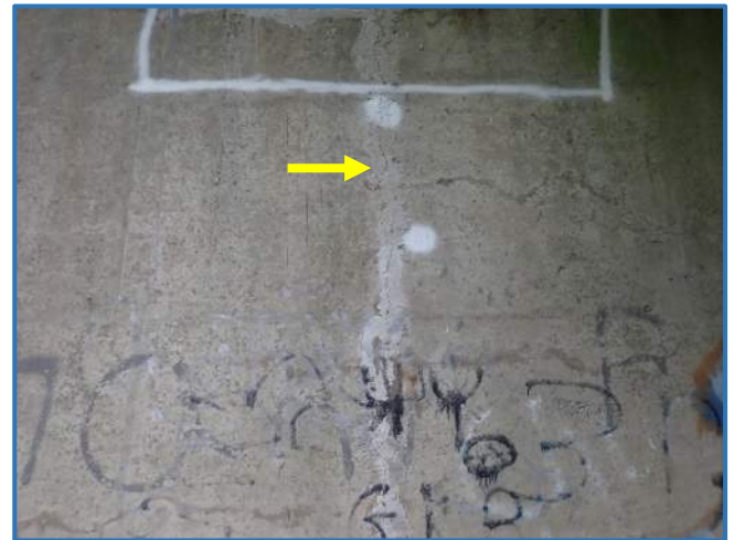
Photo 83 - Crack up to 1/8" wide by full width under Stringer 4 on west face of Pier 4, previously sealed
