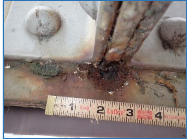
Photo 23 - 2" wide section loss on the web of the lower chord below the vertical connection, Span 1, North Truss, at Panel Point 7, looking south
