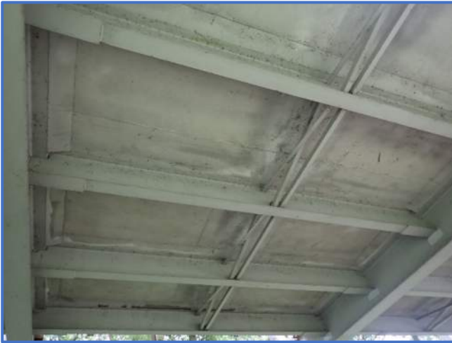
Photo 65 - Typical protective coating condition of floorbeam and stringers. Shown in Span 4
