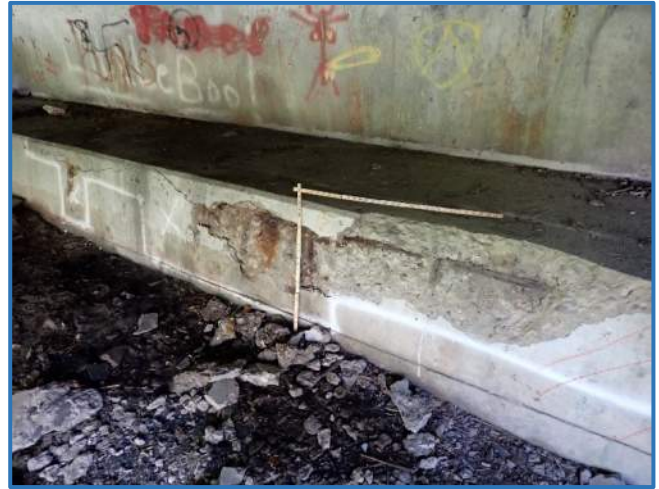
Photo 89 - Delamination and spalling with exposed rebar along bearing seat of forward abutment, looking southeast
