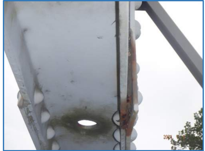
Photo 73 - Bowing of lower sway bracing connection plate due to pack rust in Span 3 at Panel Point 4, looking north
