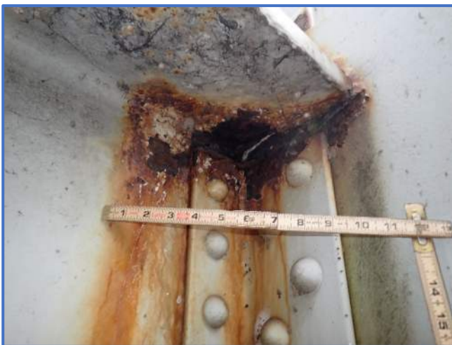
Photo 52 - Corrosion along top flange and clip angle in Span 1, Floorbeam 6 west face, north end, looking north
