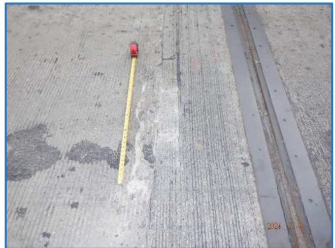
Photo 91 - Spalling in west approach slab, just west of rear abutment, looking north
