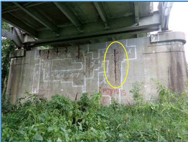
Photo 80 - Large spall under Stringer 4 on West face of Pier 4
