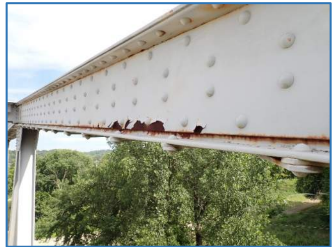
Photo 26 - Reactivated corrosion between the channel and web plate in Span 3, North Truss, member U7U8, looking northwest
