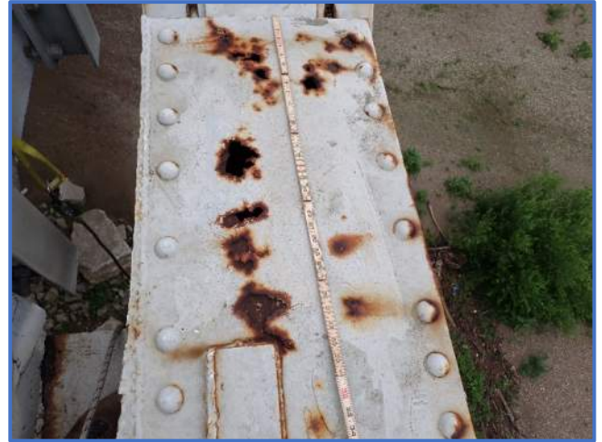
Photo 58 - Corrosion holes with 100% section loss on top cover plate in Span 2, North Truss, at Panel Point 10, looking west
