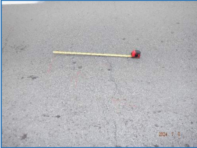
Photo 93 - Longitudinal cracks up to 1/8" wide in east approach pavement, looking north
