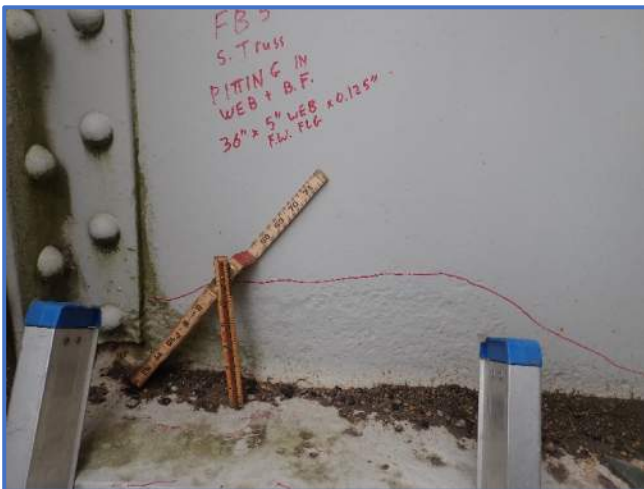
Photo 47 - Pitting along bottom of floorbeam web and top of bottom flange of Floorbeam 5 east face, Span 4, at Stringer 5, looking west
