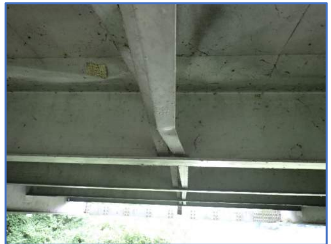
Photo 67 - Deformed diaphragm in Span 1 at Floorbeam 2, looking north
