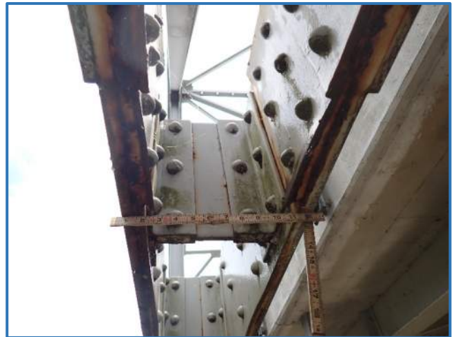
Photo 14 - 1/2" pack rust in lower chord plates in Span 2, North Truss, member L7L8, looking east
