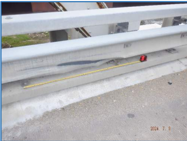
Photo 9 - Impact damage to metal railing, showing Span 3, south railing, between Panel Points 0 and 1
