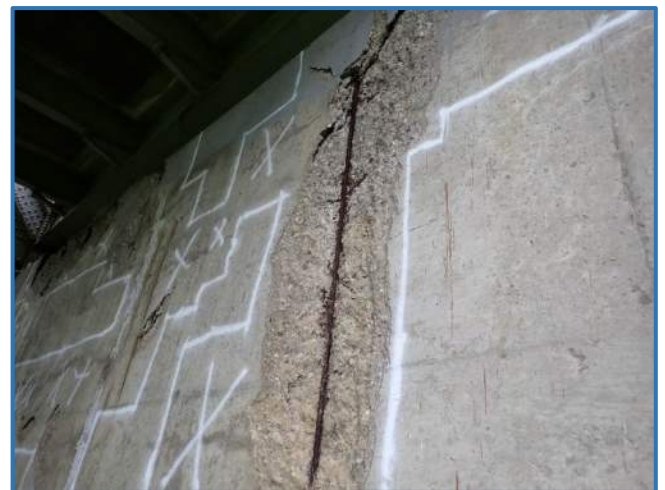
Photo 81 - Spall in west face of Pier 4, under Stringer 4 with exposed, debonded rebar
