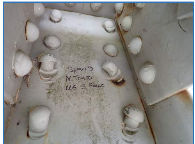
Photo 31 – Improperly installed rivets in stiffener plate, Span 3, North Truss, at Panel Point 6, looking north
