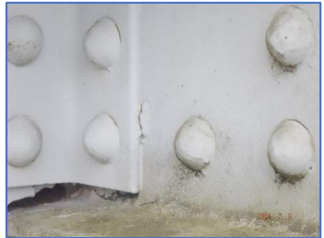
Photo 33 - Crack in tack weld between upper chord and sway bracing connection plate in Span 4, South Truss, at Panel Point 4, looking southeast
