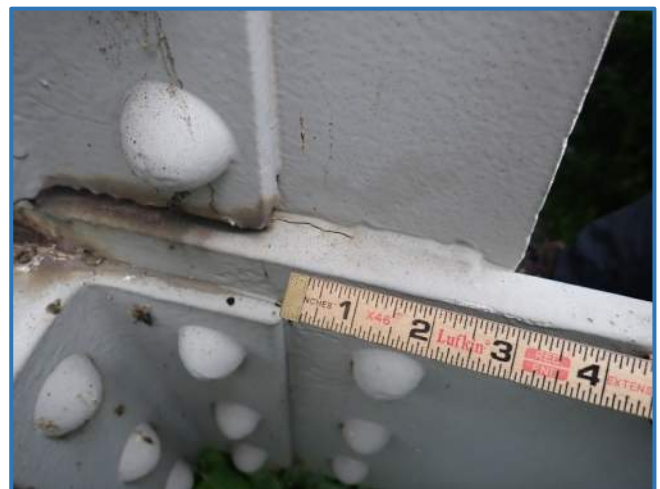
Photo 19 - Tack weld between lower chord plate and gusset plate, Span 1, South Truss, Panel Point 1, looking north
