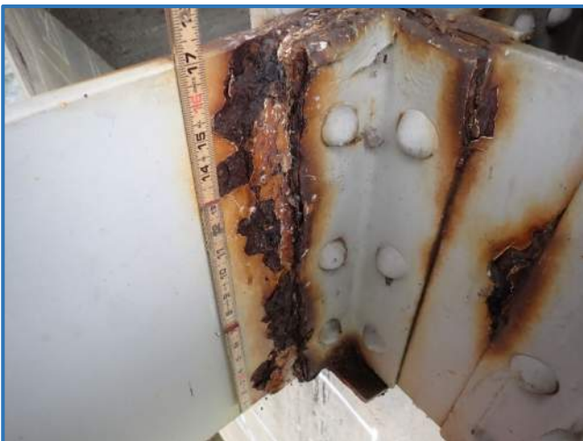
Photo 24 - Active laminar corrosion throughout the connection, Span 2, North Truss, at Panel Point 0, looking west
