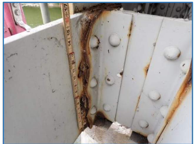
Photo 16 - 3/4" pack rust between lower chord and diaphragm, Span 2, South Truss, member L0L1
