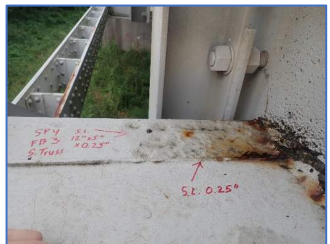
Photo 49 - Pitting with section loss along the top of top flange, at south end of Floorbeam 1, Span 4, looking west
