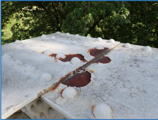
Photo 25 - Typical paint spot failure on top of upper chord, with active corrosion. Shown Span 4, North Truss, east of U1, looking northwest
