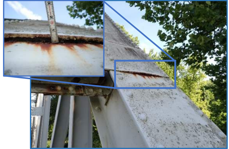
Photo 36 - 1/2" pack rust between portal bracing connection plate and edge post in Span 4, North Truss, on U7L8, looking west
