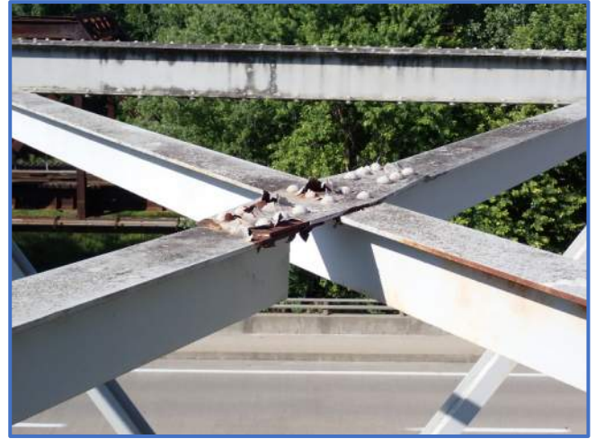
Photo 66 - Typical paint failure of top of upper lateral bracing connection plate with surface corrosion. Shown in Span 4, between Panel Points 3 and 4, looking south
