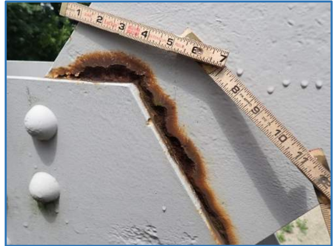
Photo 45 - 3/16" deep section loss along lower gusset plate on south face of diagonal in Span 2, North Truss, at Panel Point 8, looking north
