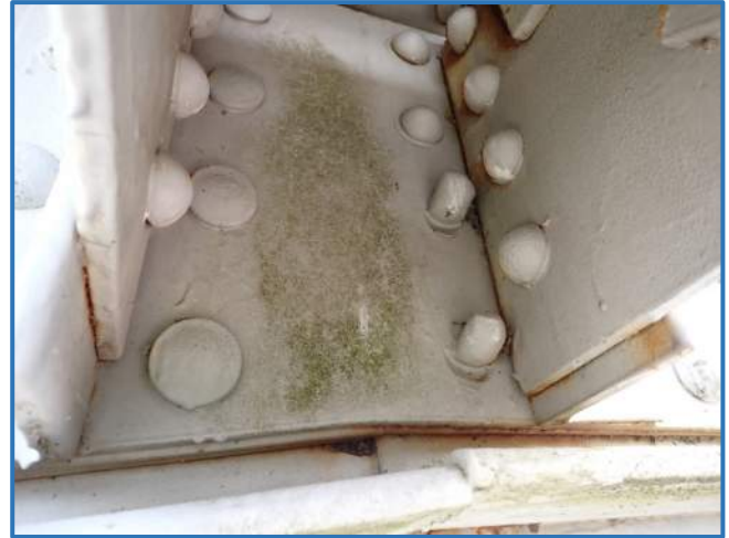
Photo 29 – Typical improperly installed rivet heads in stiffener plate, Span 3, North Truss, at Panel Point 3
