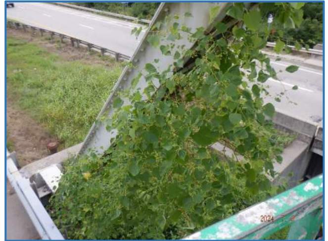
Photo 96 - Vegetation growth along underside of end post in Span 4, South Truss, between Panel Points 7 and 8, looking northeast
