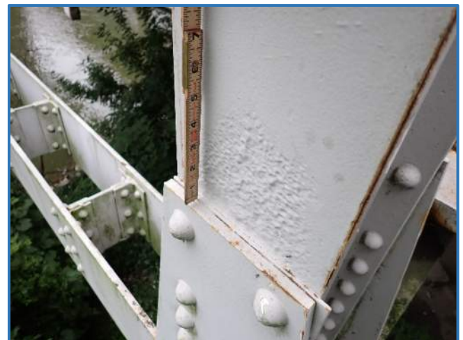
Photo 38 - Painted over pitting up to 3/16" deep on vertical just above lower chord connection, Span 1, North Truss, at Panel Point 1, looking northwest
