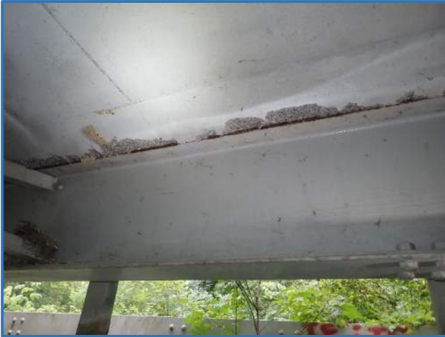
Photo 2 - Typical haunch spall. Shown 15' long by 6" high by 0.5" deep in Span 4, top of Stringer 1, looking north
