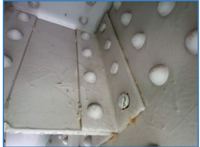
Photo 30 - Typical missing rivet heads on south diaphragm clip angle, Span 3, North Truss, at Panel Point 4, looking southeast
