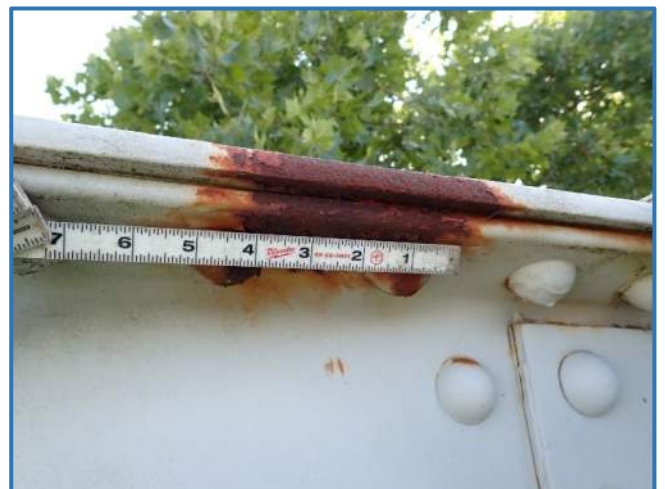
Photo 28 - 6" long by 4" wide paint failure in Span 4, North Truss, member U6U7, looking north
