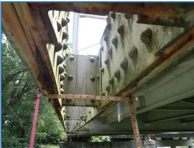
Photo 15 - 3/4" pack rust in lower chord plates in Span 3, North Truss, member L7L8, looking east
