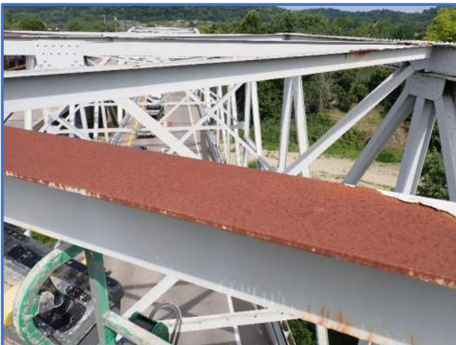
Photo 63 - Upper lateral bracing paint failure with surface corrosion. Shown is worst case in Span 3, North Truss, between Panel Points 5 and 6, looking southeast
