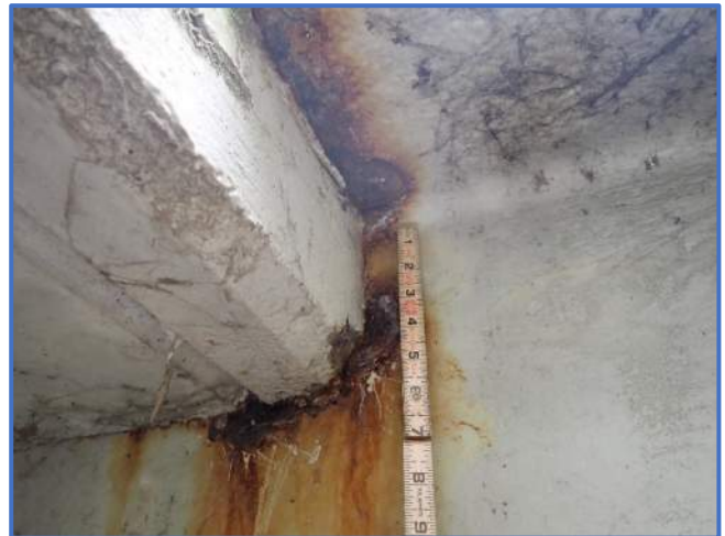
Photo 51 - Corrosion at deck and Floorbeam top flange interface. Shown Span 3, Floorbeam 8, north end, looking west
