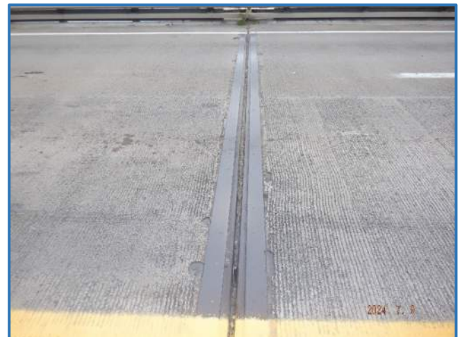
Photo 7 - Typical expansion joint with debris and surface corrosion. Shown is Pier 2 joint, looking north
