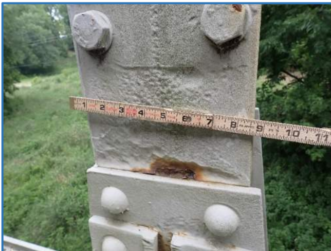
Photo 37 - Pitting with active corrosion and section loss (2" high by 6" wide by 3/8" deep) on vertical just above lower chord connection in Span 3, North Truss, at Panel Point 9, looking west
