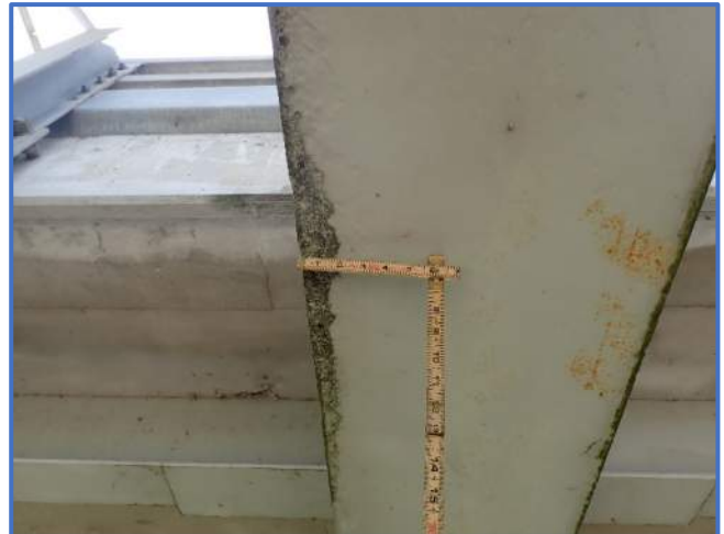
Photo 50 - Pitting along underside of Floorbeam 1, Span 3, looking south
