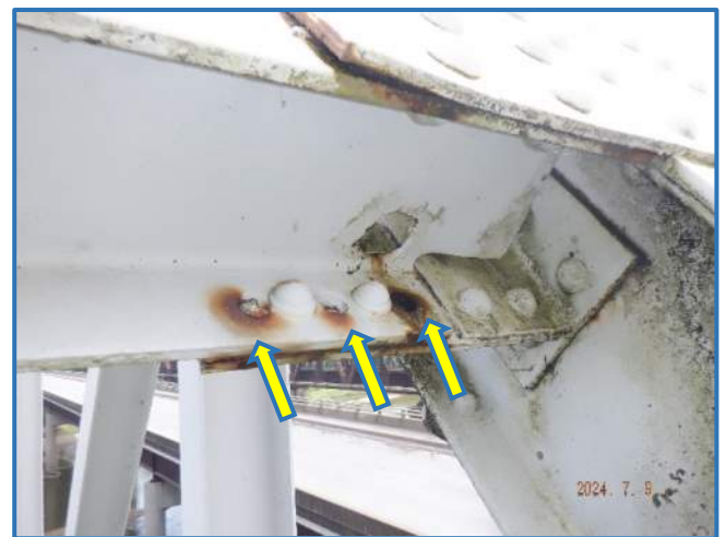
Photo 71 - Misdrilled holes on lower sway brace in portal frame in Span 1, at Panel Point 1, at South Truss connection, looking east
