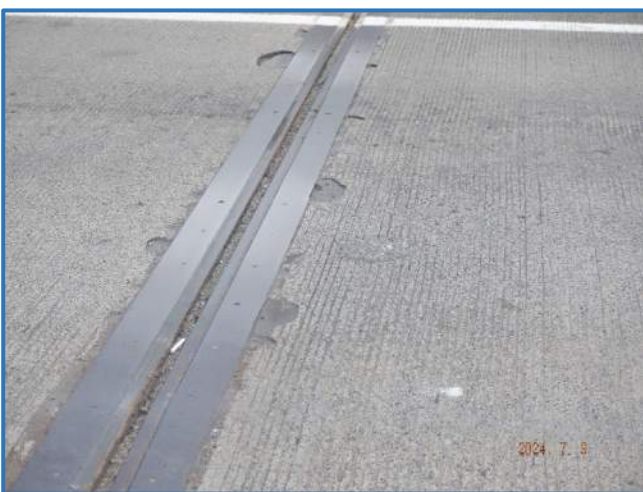
Photo 4 - Spalling along Pier 2 joint
