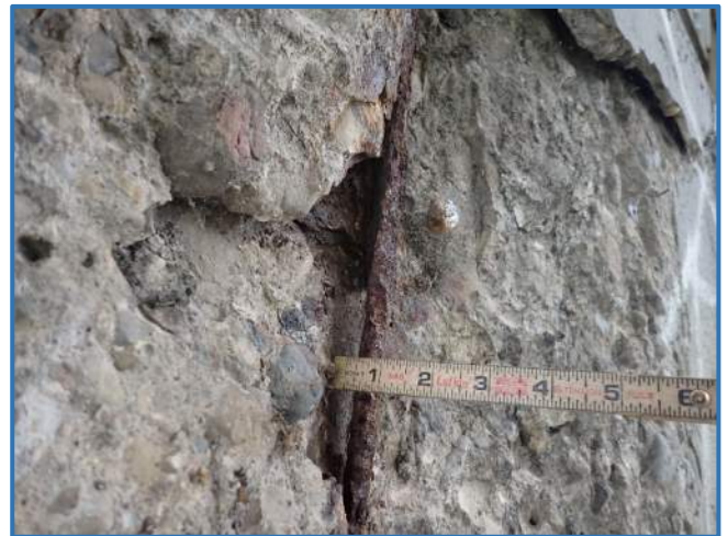
Photo 75 - Spall in west face of Pier 2 with exposed debonded rebar under Stringer 5
