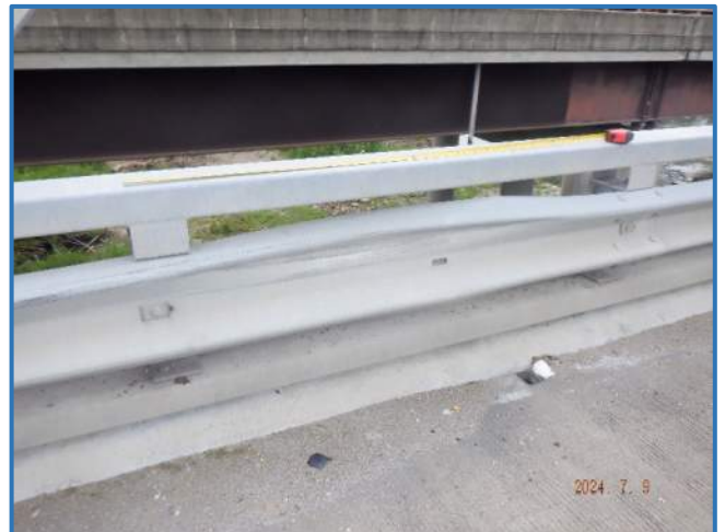
Photo 10 - Impact damage to metal railing, showing Span 3, south railing, between Panel Points 1 and 2
