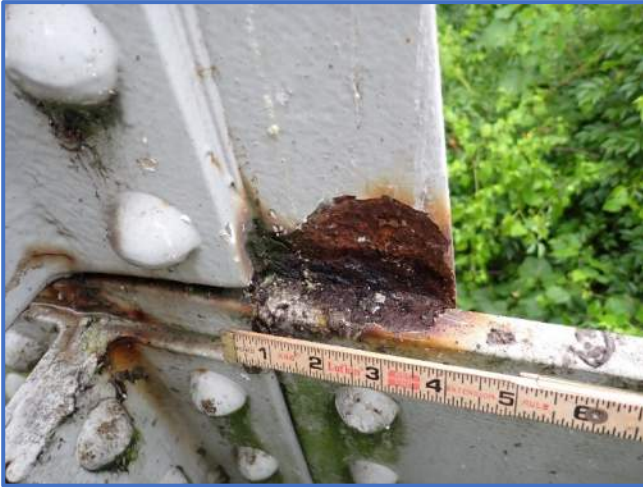
Photo 57 - Section loss on east edge of lower gusset plate at top of lower chord, Span 1, North Truss, at Panel Point 1, looking north
