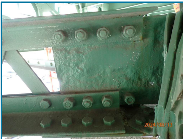
Photo 81 – Painted over pitting up to 3/16" (L0, Center Truss, Span 5, looking northeast).
