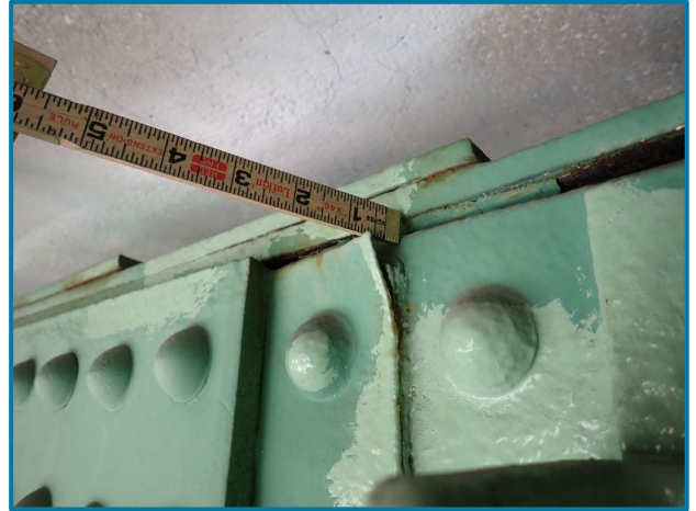
Photo 45 – Pack rust at the top splice plate and distortion at the fill plate (U12U13 of the Center Truss, Span 6).
