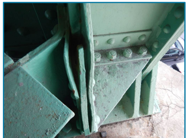
Photo 68 – 1" pack rust between the lower lateral bracing fill plate and the gusset plate (L0, South Truss, Span 5).
