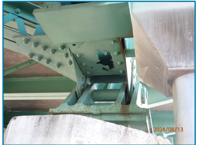
Photo 41 – 10” H x 6” W corrosion hole in the lower batten plate at the bearing (L0 of the North Truss, Span 5).
