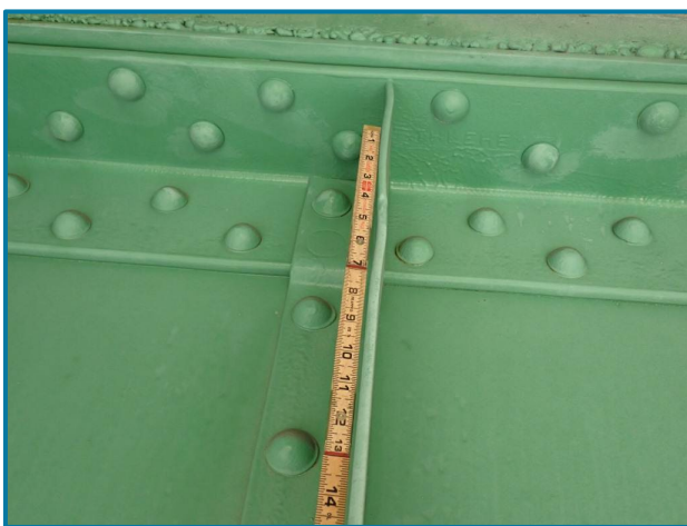
Photo 25 – 1/4" distortion over 4" at the stiffener (North Girder, Span 15, looking south).
