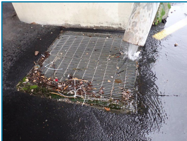
Photo 19 – Grate partially obstructed and drainpipe not directly aimed at grate center (Pier 5 shown, looking north).
