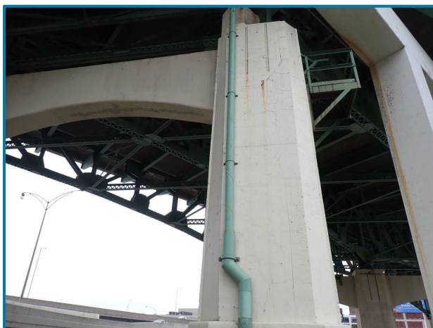
Photo 91 – Hairline cracking with rust staining (Pier 12, North Column, East Face, looking west).
