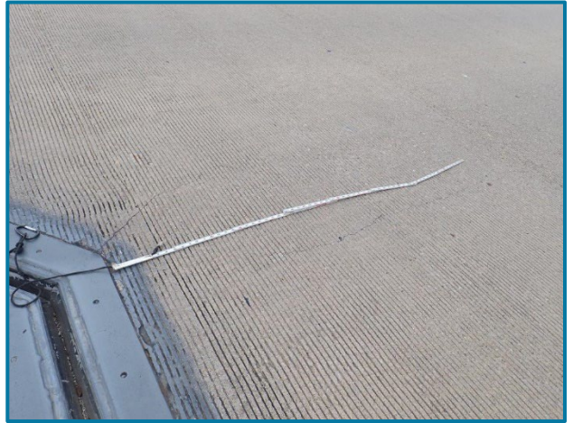
Photo 6 – Moderate to wide cracks near where the expansion joint armor bends (near Pier 10).
