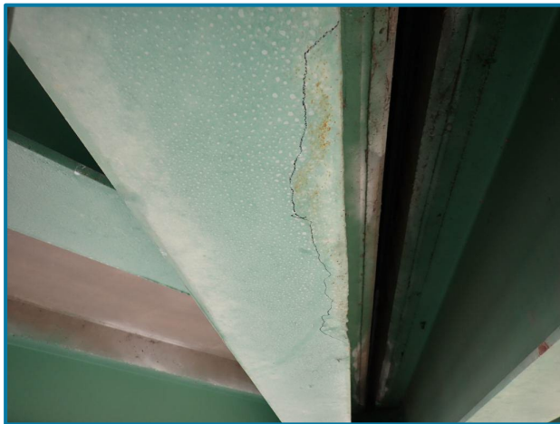
Photo 62 – 2' L x 3" W area of light surface corrosion to the bottom flange (Span 6 over Pier 7).
