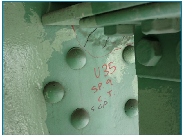
Photo 47 – 6" L x 2" H x 1/8" D pitting underneath the floorbeam connection (U35 of the Center Truss, Span 9).
