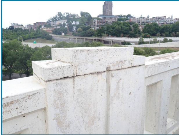
Photo 8 – Crack with delamination at the decorative post cap (looking southwest).
