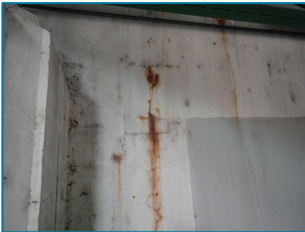
Photo 93 – Hairline cracking with rust staining (Abutment 1, East Face, looking west).
