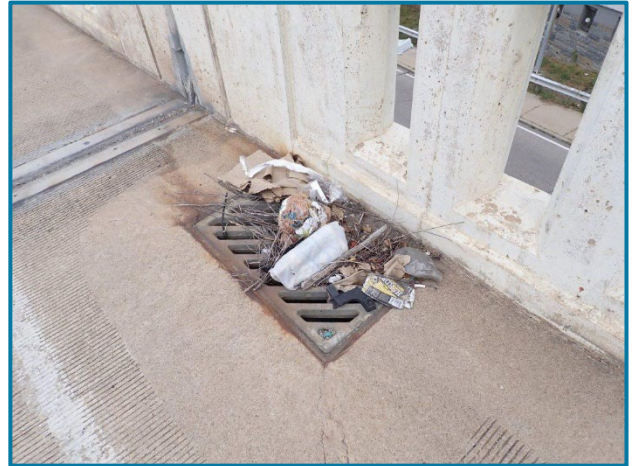
Photo 18 – Debris/Trash build-up at isolated deck scuppers (Pier 17 shown, looking north).
