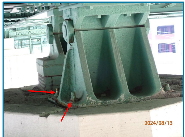
Photo 79 – Up to 40% section loss to the anchor nuts (Pier 4, Center Girder, Span 3, looking southeast).
