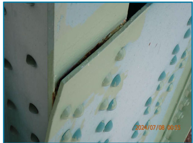
Photo 67 – Typical pack rust at the gusset plate causing distortion (L33, North Truss, Span 9).
