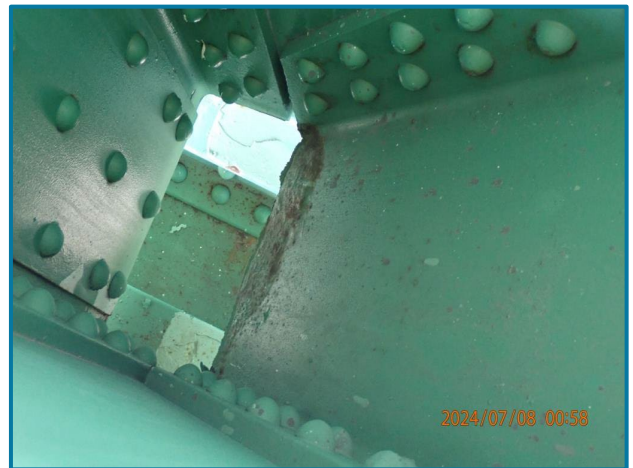
Photo 60 – Surface corrosion at the diagonal end with pack rust forming (U32L33 of the North Truss, Span 9).
