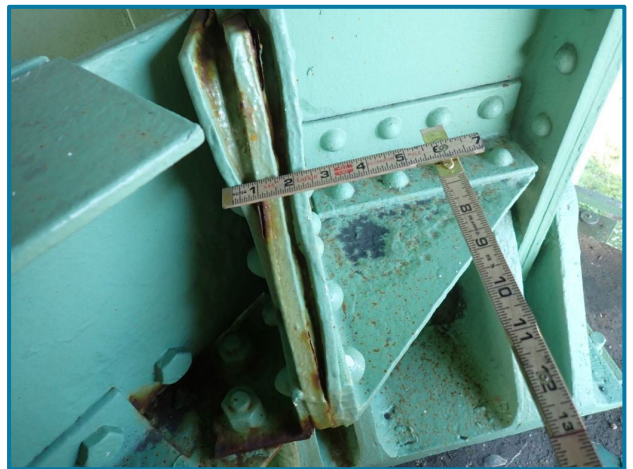
Photo 85 – Up to 1" pack rust at the connection to the truss (L20, North Truss, Span 11, looking northwest).
