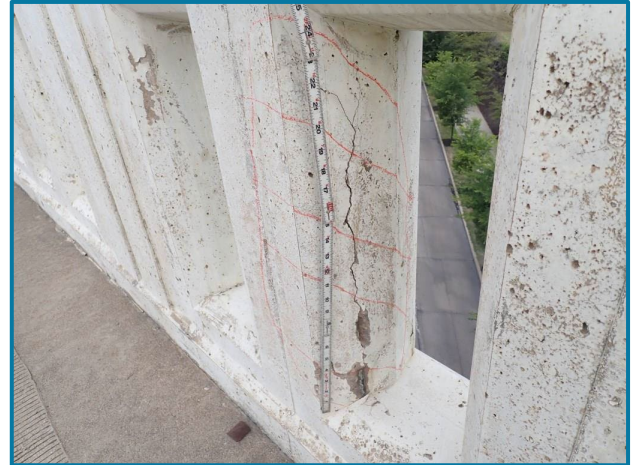
Photo 9 – 2' H x 1' W delamination with a crack in the north railing stem (looking southeast).
