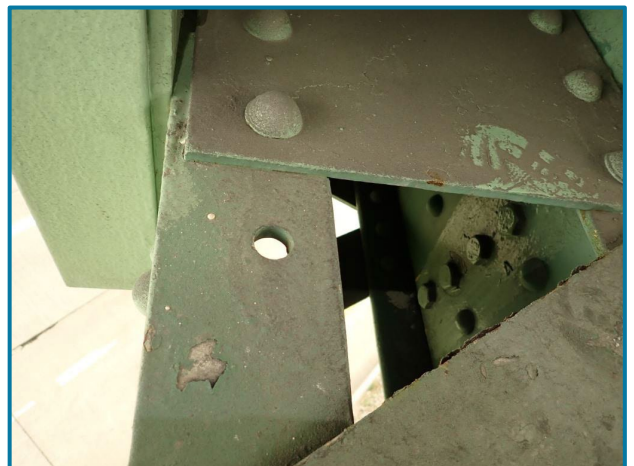
Photo 42 – Blind hole in the lower chord top flange near (L27L28 of the Center Truss, Span 8).
