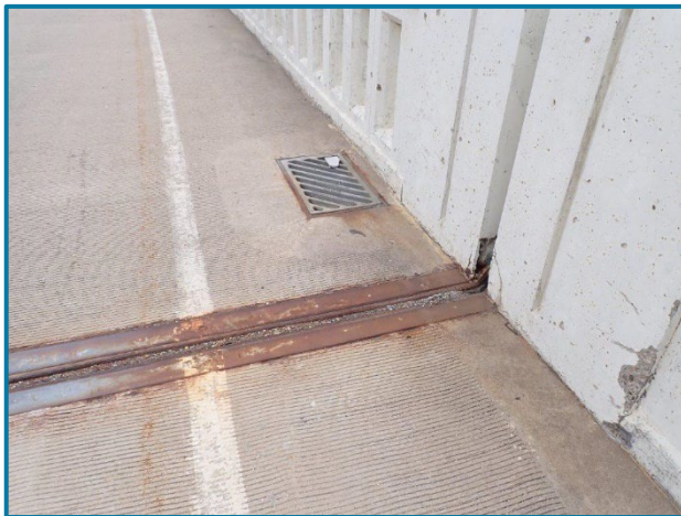
Photo 14 – Surface corrosion to the deck joint armour in the shoulder (Pier 16 shown, looking east).
