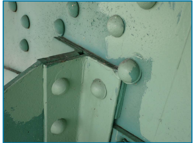
Photo 70 – Rivet deformation due to conflict with the sway bracing connection (L28, Center Truss, Span 8).
