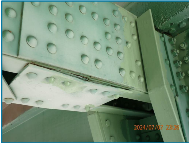
Photo 44 – 3/4" pack rust at the bottom batten plate (U42U43 of the North Truss, Span 9).
