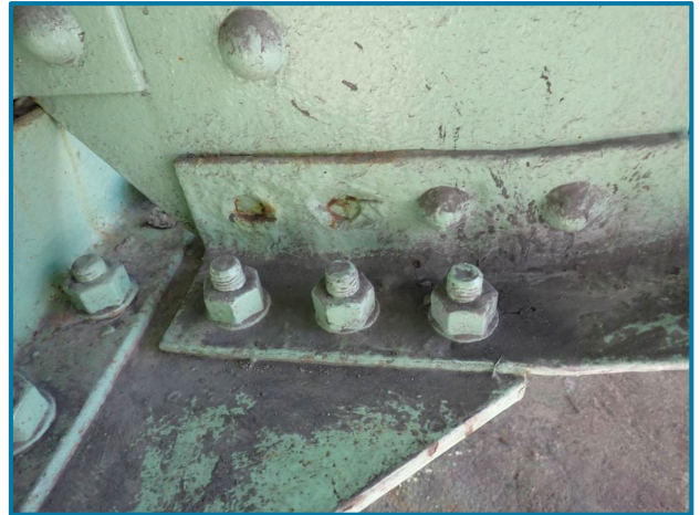
Photo 83 – 2 sheared off rivet heads at the sway bracing bottom strut (L0, Center Truss, Span 10, looking west).
