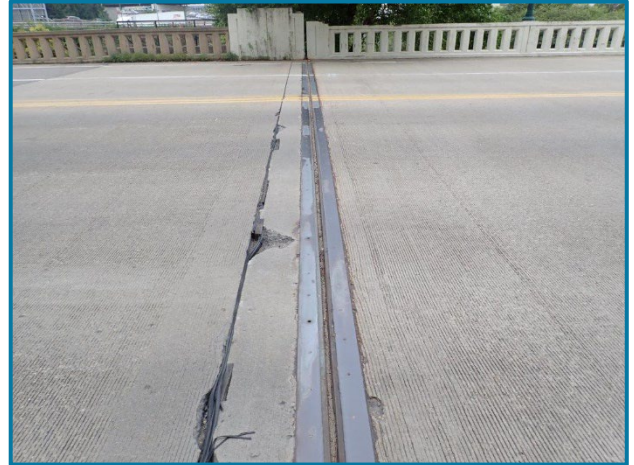
Photo 17 – Spalls in the joint header with damaged construction joint material (Abutment 1 shown, looking north).
