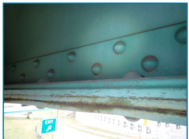
Photo 31 – 1/16" pack rust between the bottom flange cover plates (Span 16 shown, looking northwest).
