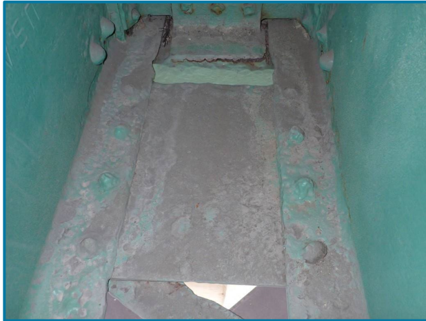
Photo 40 – Up to 50% section loss to the rivet heads inside the lower chord (L0L1 of the Center Truss, Span 7).
