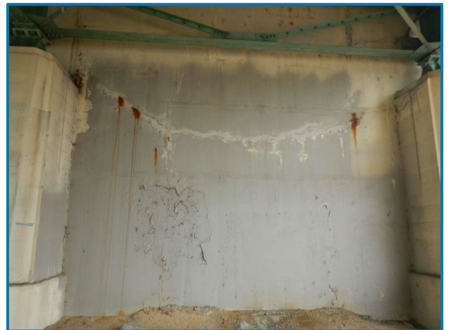
Photo 96 – 18' L horizontal sealed crack with rust staining and efflorescence (Abutment 18, West Face, looking east).
