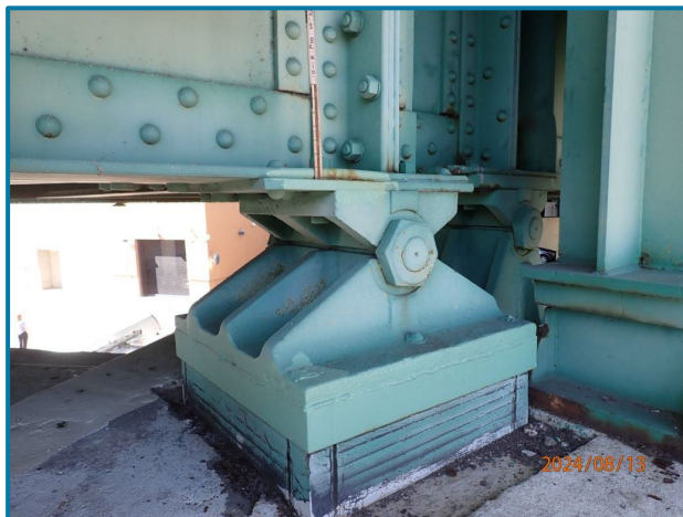
Photo 75 – 3/16” pack rust between the lower chord and the bearing (North Truss, Span 4, looking southwest).
