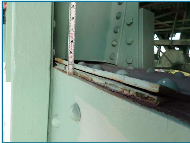
Photo 36 – Pack rust prying up the lower chord batten plate (L5L6 of the South Truss, Span 7).
