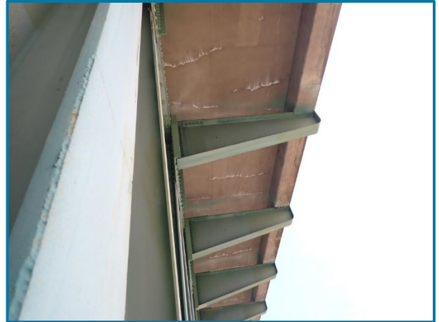
Photo 4 – Transverse cracking with efflorescence in the deck overhang (Span 9 shown).
