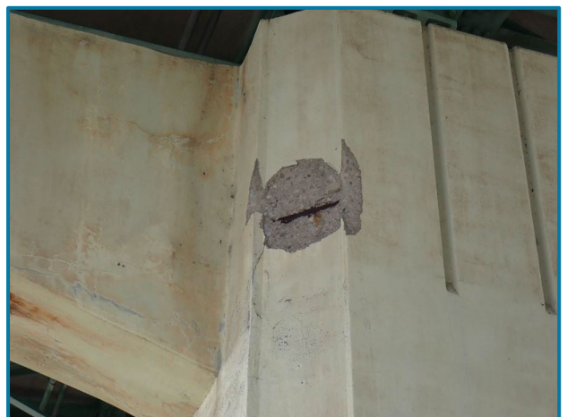
Photo 92 – 2' L x 2' H x 2" D spall with exposed rebar (Pier 13, Center Column, SE Corner, looking northwest).
