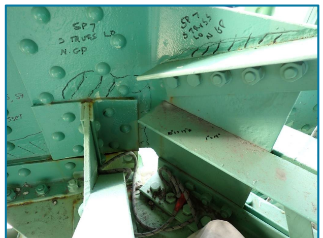
Photo 72 – 3/16" painted over pitting to multiple locations on the gusset plate (L0, South Truss, Span 7).
