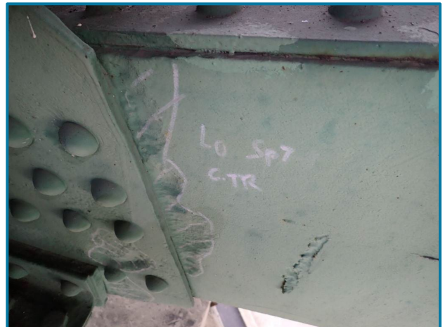
Photo 39 – 3/16” deep section loss to the lower chord adjacent to the gusset plate (L0L1 of the Center Truss, Span 7).
