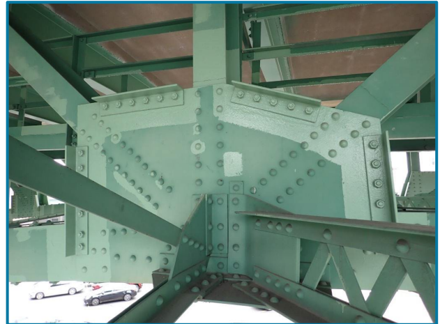
Photo 65 – Rehabilitation work to stiffen the gusset plates that were bowed (looking west).
