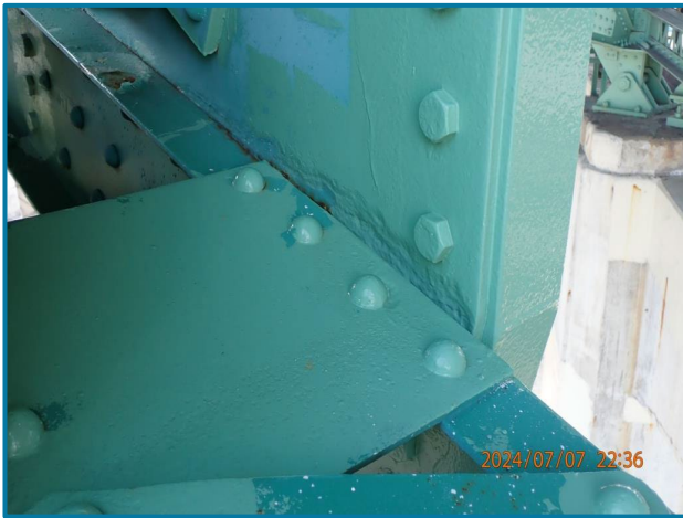
Photo 73 – 3/16” painted over pitting adjacent to the lower chord (L1, North Truss, Span 10).
