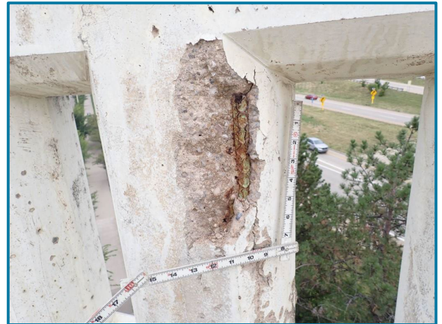
Photo 10 – Spall with exposed rebar in the railing stem (looking northwest at north railing).
