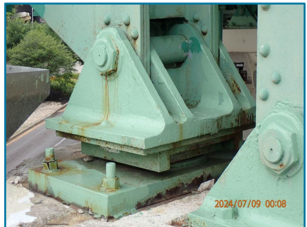
Photo 80 – Surface corrosion and rust staining to the bearing (L14, North Truss, Pier 8, looking southeast).
