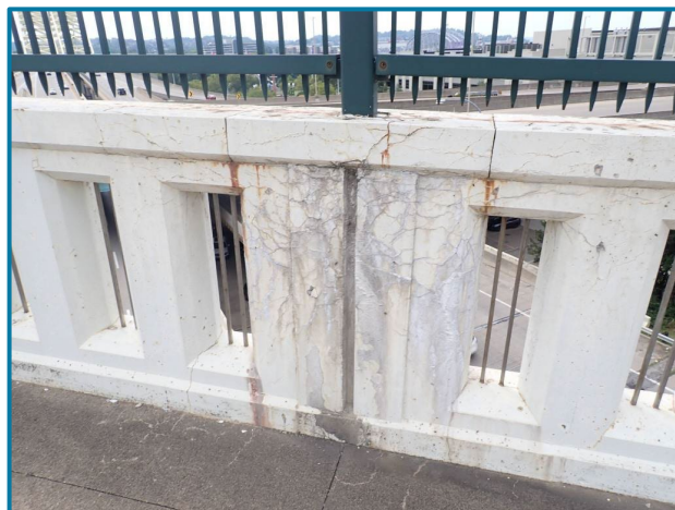
Photo 11 – Map cracking with efflorescence (possible ASR) in the concrete railing (looking south at the south railing).
