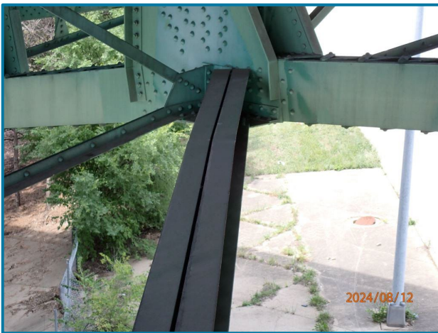
Photo 84 – Impact damage to the lower lateral bracing (6' south of L18, Center Truss, Span 8, looking north).
