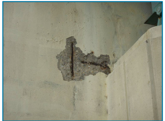
Photo 94 – 3' L x 2' H x 1" D spall with exposed rebar (Abutment 18, West Face, looking east).
