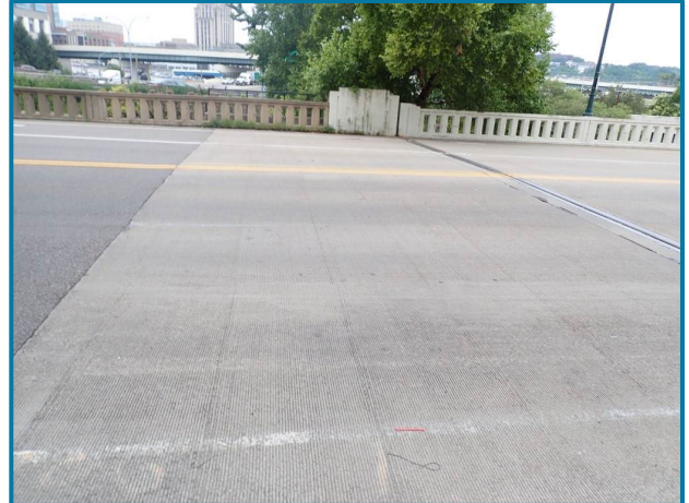
Photo 103 – Wear in the wheel lines of the approach slab (West Approach Slab, looking north).
