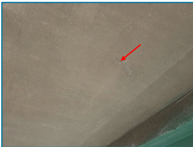
Photo 2 – Typical hairline longitudinal cracks in the deck between the floorbeams (Span 10 shown).
