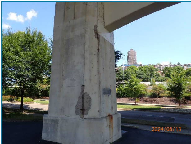
Photo 89 – Two spalls with exposed rebar (Pier 7, North Column, South and West Faces, looking northeast).
