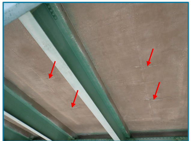
Photo 3 – Longitudinal cracking with efflorescence in the deck between floorbeams (Span 9 shown).
