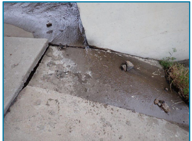
Photo 20 – Slope protection is broken and undermined (Pier 11 shown, looking south).
