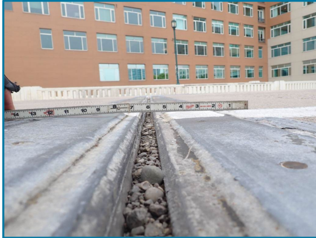
Photo 16 – 1/2" vertical offset in the deck joint (Pier 3 shown, looking south).
