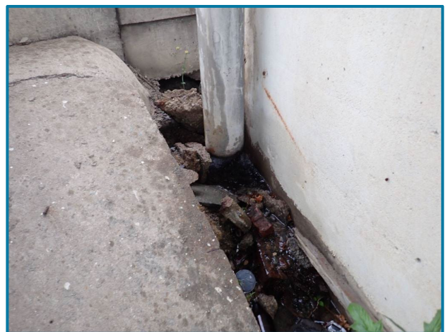
Photo 22 – Slope protection and adjacent approach slab are undermined (Pier 13 shown, looking west).
