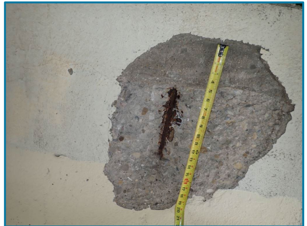
Photo 102 – 1'-8" diameter x 2" D spall with exposed rebar (Pier 16, West Face, looking east).
