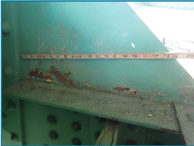
Photo 69 – Failed protective coating system with surface corrosion (L44, Center Truss, Span 9).
