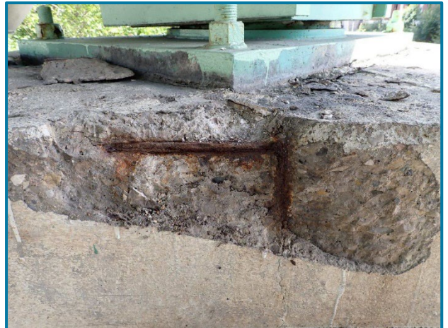
Photo 90 – 1'-9" L x 8" H x 2" D spall with exposed rebar (Pier 8, South Column, North Face, looking south).
