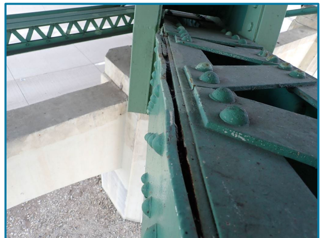
Photo 34 – Pack rust causing warping of the web plate (L28L29 of the Center Truss, Span 8, looking east).
