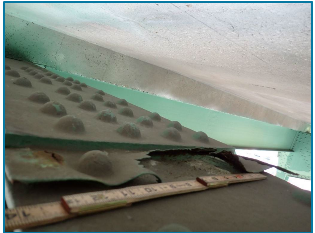
Photo 48 – 8" L x 2" W area of 100% section loss to the fill plate (U9U10 of the Center Truss, Span 6).
