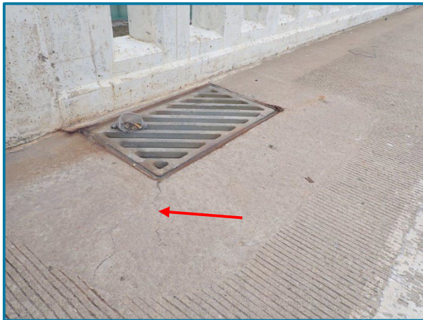
Photo 5 – Moderate to wide cracks propagating from the scupper grate corner (near Pier 10).
