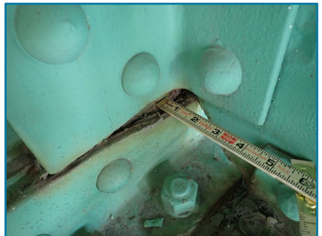
Photo 82 – 3/4" pack rust at the bottom strut flange angle (L20, North Truss, Span 6, looking northwest).
