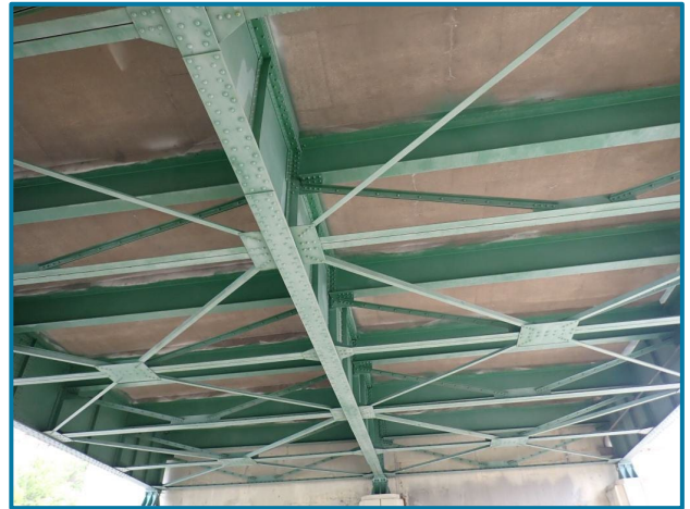
Photo 1 – Typical condition of the deck underside (looking up and east in Span 17).
