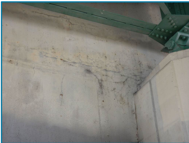
Photo 95 – Hairline map cracking over an area of 5' L x 2' H (Abutment 18, West Face, looking east).
