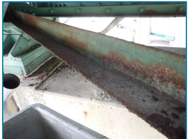
Photo 86 – Paint failure at the lower lateral bracing (Floorbeam 0, South Girder, Span 14, looking west).
