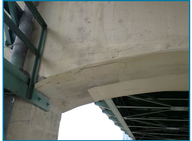
Photo 100 – 10' L section of cracked repair patch that extends 1' underneath (Pier 15, East Face, looking west).
