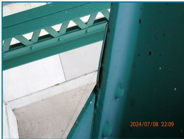
Photo 59 – 1/8” pack rust at the fill plate causing distortion to the plate (U16L17 of the North Truss, Span 8).
