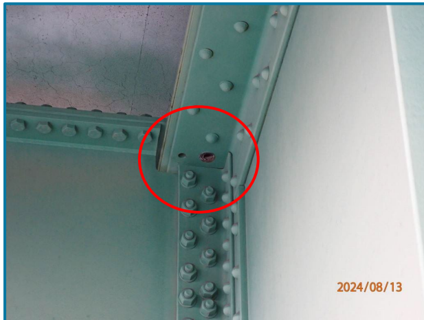
Photo 28 – Blind hole and missing rivet (Span 3 shown, looking east).
