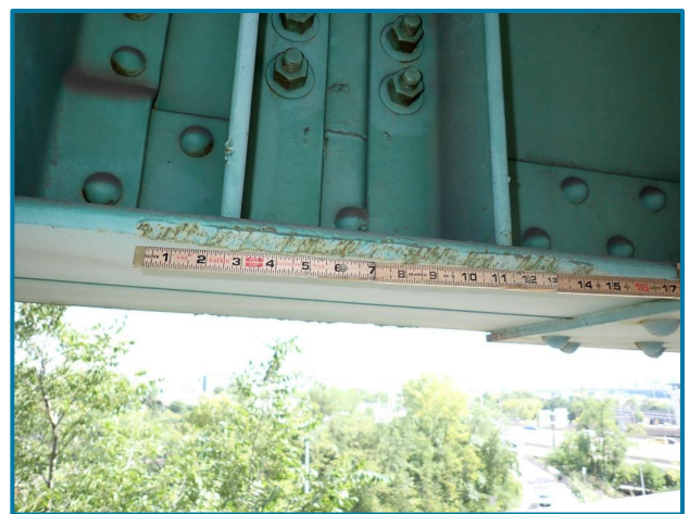
Photo 26 – 1'-2" torch cut bottom flange (Span 14 shown, looking south).
