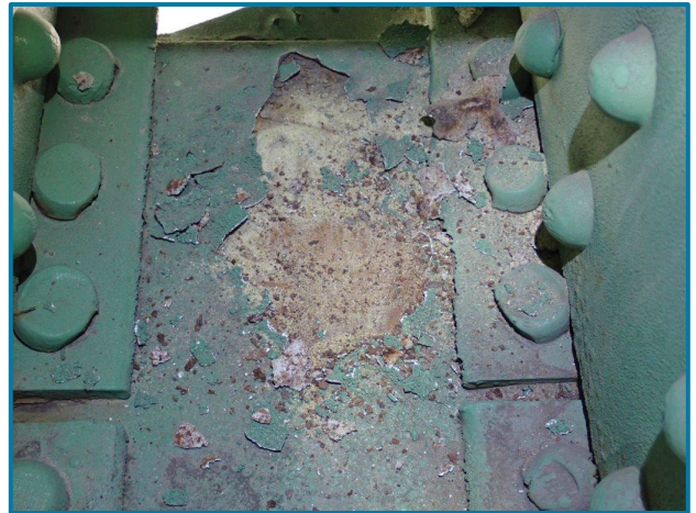
Photo 37 – Peeled paint with exposed bare metal and surface corrosion (L38 of the Center Truss, Span 9).
