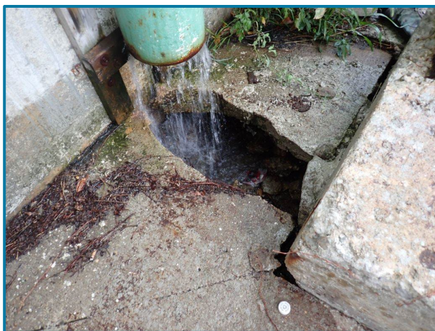
Photo 21 – Broken slope protection with a void underneath drainpipe (Pier 12 shown, looking northeast).
