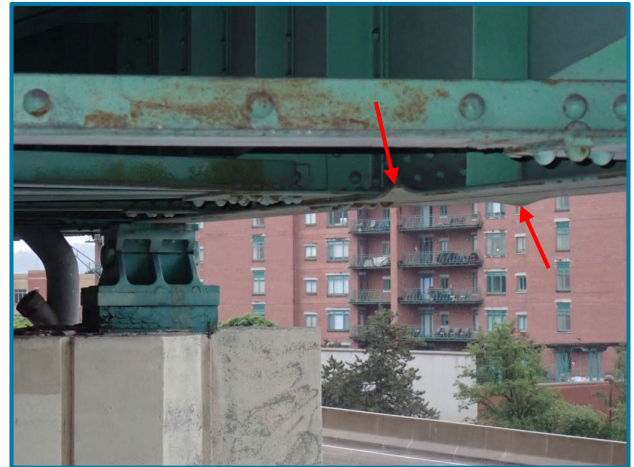
Photo 27 – Bent bottom flange (Span 12 shown, looking southeast).
