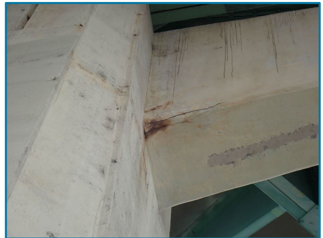
Photo 98 – 4' L wide crack with rust staining (Pier 12, West/Bottom Face, looking east).
