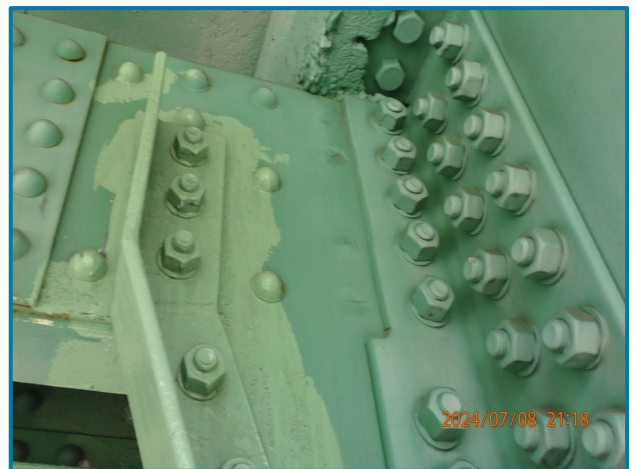
Photo 50 – Four plug welds on each side of the upper chord member (U25 of the North Truss, Span 8).
