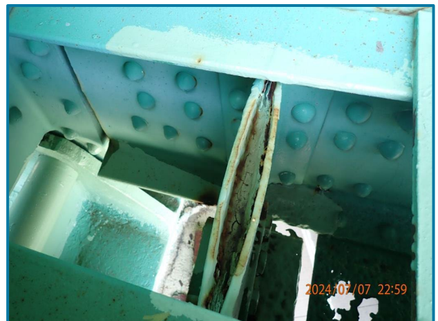
Photo 35 – Pack rust up to 1-1/2” wide at the internal stiffeners (L43L44 of the North Truss, Span 9).
