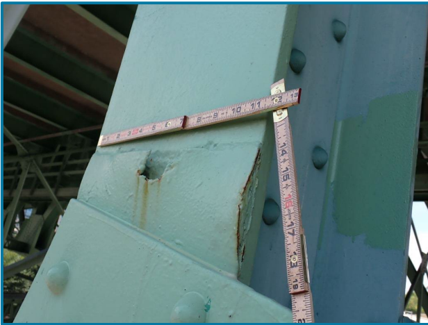
Photo 51 – 9/16” pack rust at the fill plate causing distortion to the plate (U13L13 of the South Truss, Span 7).
