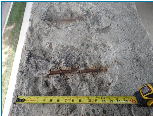
Photo 97 – (2) 1'-4" diameter x 1-1/2" D spall with exposed rebar (Pier 8, Top Face, looking down and north).
