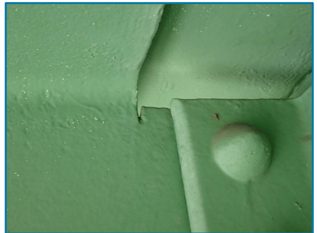
Photo 64 – 3/8" overcut in the floorbeam cope (south side of U39, Center Truss, Span 9).
