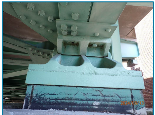
Photo 76 – Missing bolt attaching the sole plate to the girder (North Girder, Floorbeam 0, Span 4, looking west).
