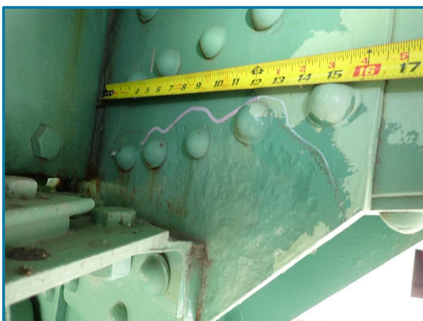
Photo 71 – 2'-4" L x 6" H x 3/16" D painted over pitting adjacent to the bearing (L20, South Truss, Span 6).
