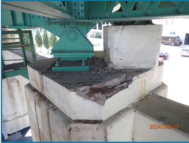
Photo 87 – 4' L x 8" W x 6" D spall with exposed rebar (Pier 5, Center Column, North Face, looking southwest).
