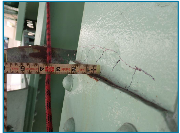
Photo 52 – 1/8” section loss across the flange width at the lower gusset plate (U44L44 of the Center Truss, Span 9).
