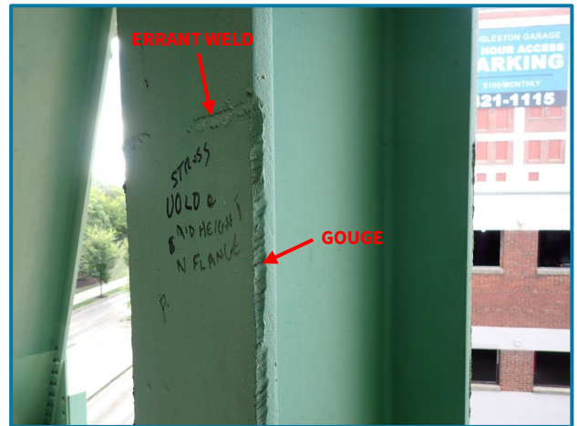
Photo 54 – Errant weld attached to the vertical flange (U0L0 of the South Truss, Span 7).
