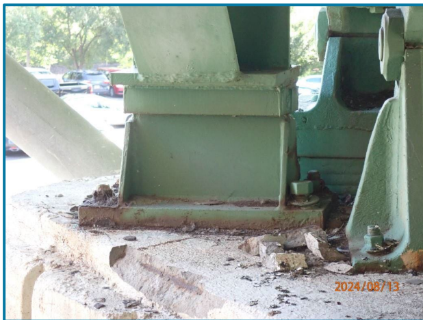
Photo 78 – 1 loose anchor nut and 2 with 30% section loss (Pier 4, North Girder, Span 3, looking east).
