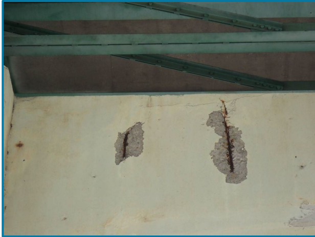
Photo 99 – 1' L x 3' H x 1" D and 1' L x 1' H x 1" D spalls with exposed rebar (Pier 13, East Face, looking west).
