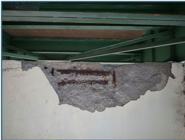
Photo 101 – 3'-8" L x 1'-1" H x 3" D spall with exposed rebar (Pier 16, East Face, looking west).
