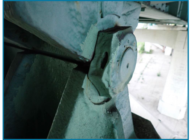
Photo 77 – Gouge in the pin nut with painted over pitting (Pier 12, Center Girder, Span 12, looking southwest).
