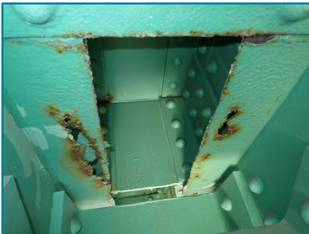
Photo 46 – Corrosion holes, pitting, and active corrosion to the bottom flanges (U0 of the Center Truss, Span 10).
