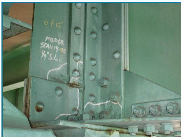
Photo 30 – 1/4" pitting at the Center Girder end (Span 14 shown, looking southwest).
