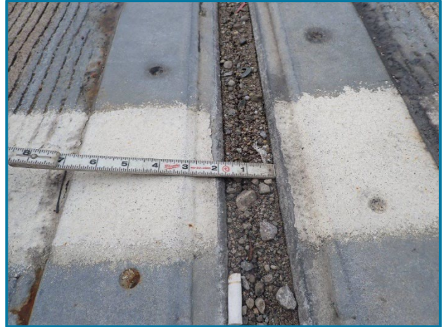
Photo 13 – Debris accumulation in the deck joint (Pier 4 shown, looking south).
