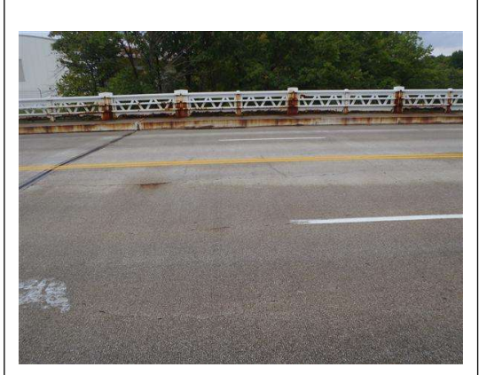
Photo 6 | Wearing surface cracking 2
