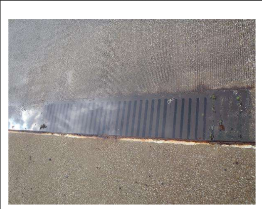
Photo 1 | Ponding and clogged scupper along south curb, Span C (typical of multiple locations)
