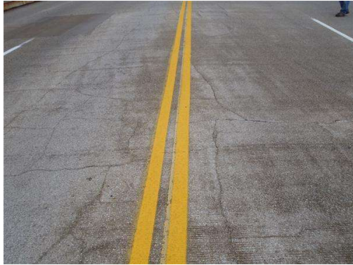
Photo 7 Wearing surface cracking
