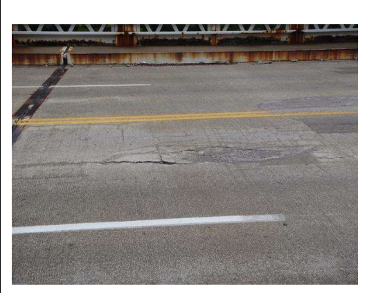
Photo 5 | Wearing surface deterioration
