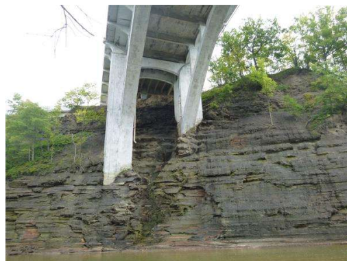
Photo 12 Continued slow erosion of the east shale banks.
