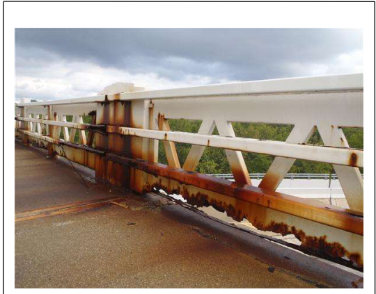
Photo 4 | Typical poor condition of railing.
