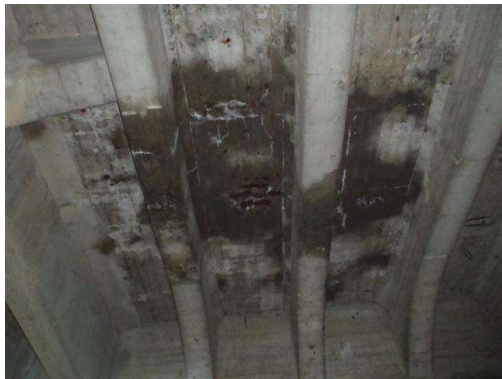
Photo 9 Typical cracking, leakage, efflorescence and spalls in approach span deck soffit.
