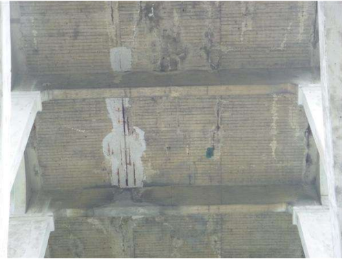
Photo 8 Typical spalls with exposed rebar in arch span deck soffit.
