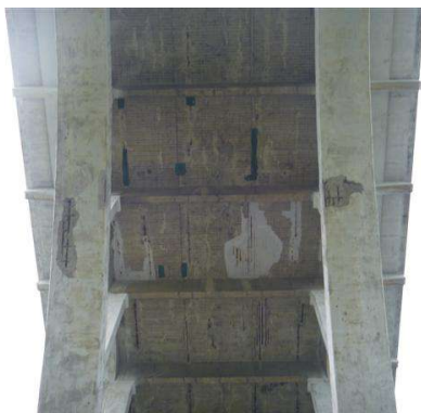
Photo 11 Typical spalls on arches.
