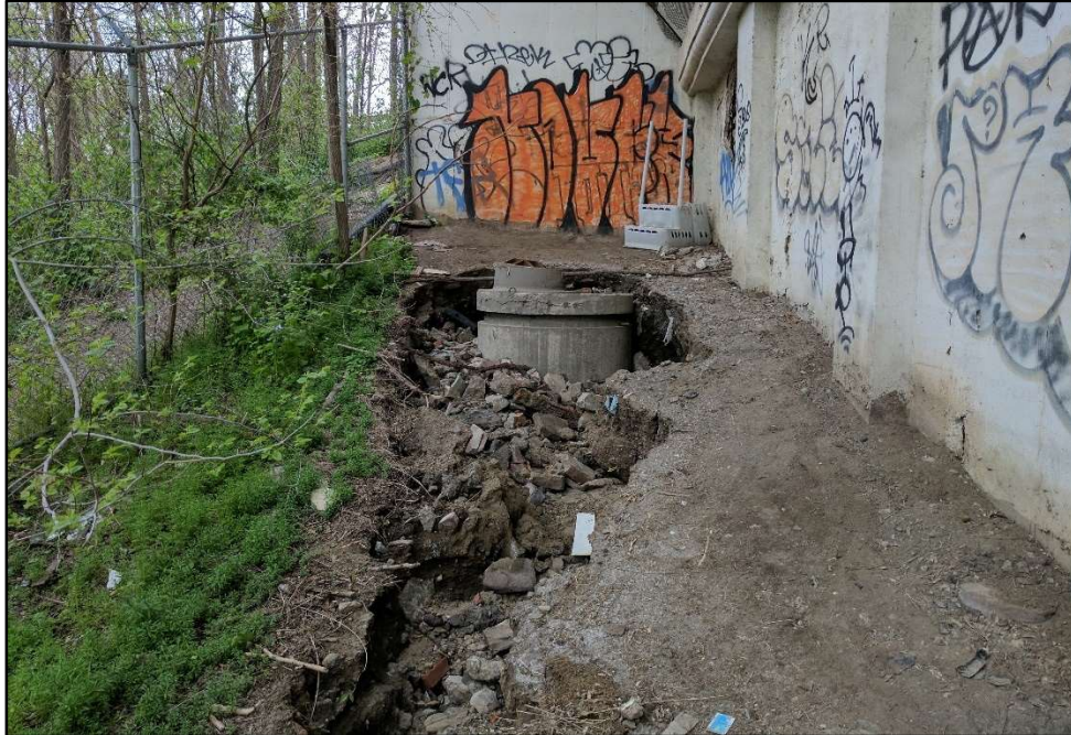
Photo 60 – Embankment Erosion at Span 1A Manhole, North of Tower A South.
