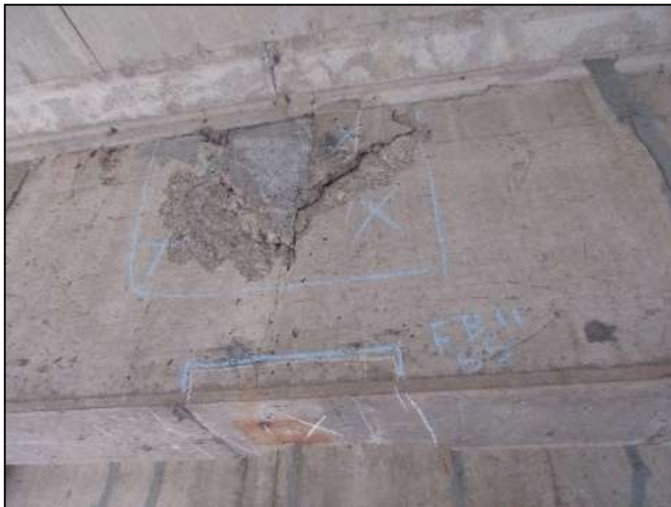
Photo 34 – Deterioration of Newer Upper Deck Floorbeam 11, Span 5.
