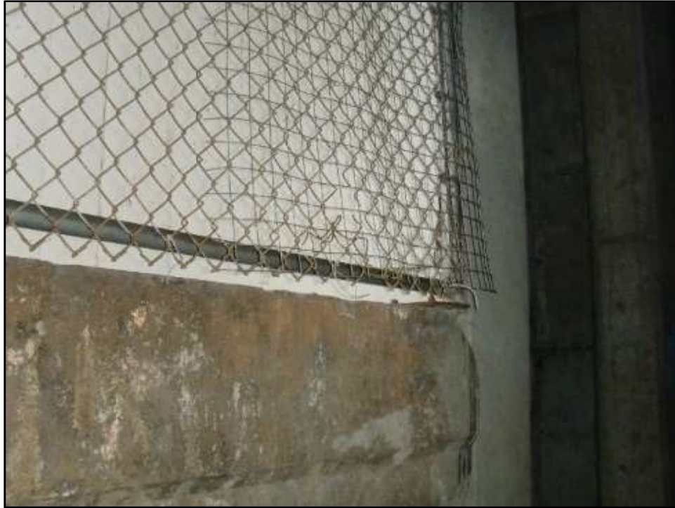
Photo 62 – Broken Ties to Fencing, Span 1A at Tower A.
