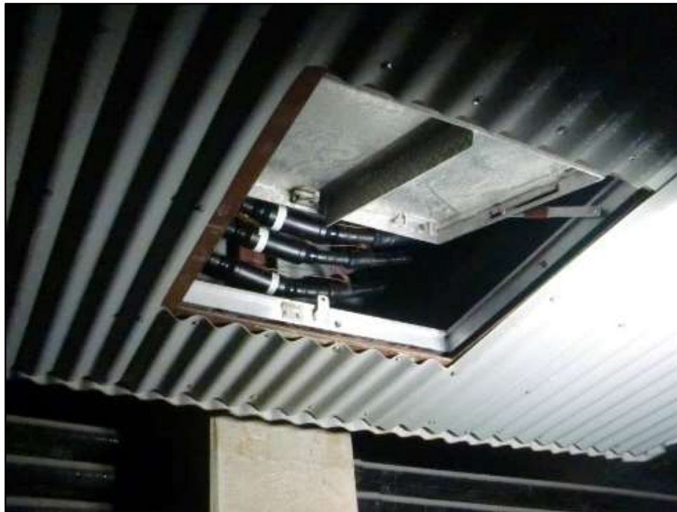
Photo 66 – Unsecure Telephone Junction Chamber, Near Column D12, West Station.
