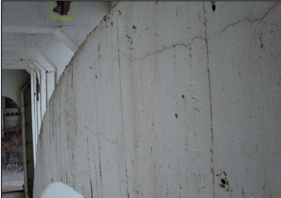
Photo 23 – Typical Horizontal Crack, Span 3 NE Arch Rib Shown.
