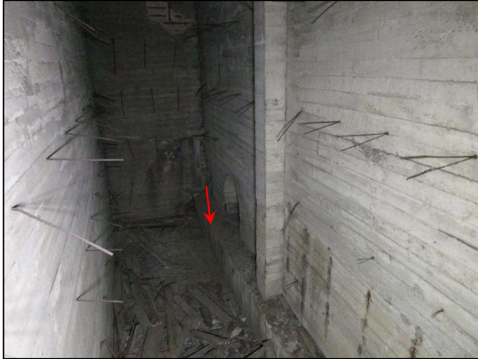
Photo 55 – Location of Tower B Footing Crack (at Arrow), Looking South in Cellular Construction, Panel 2, Span 1B.
