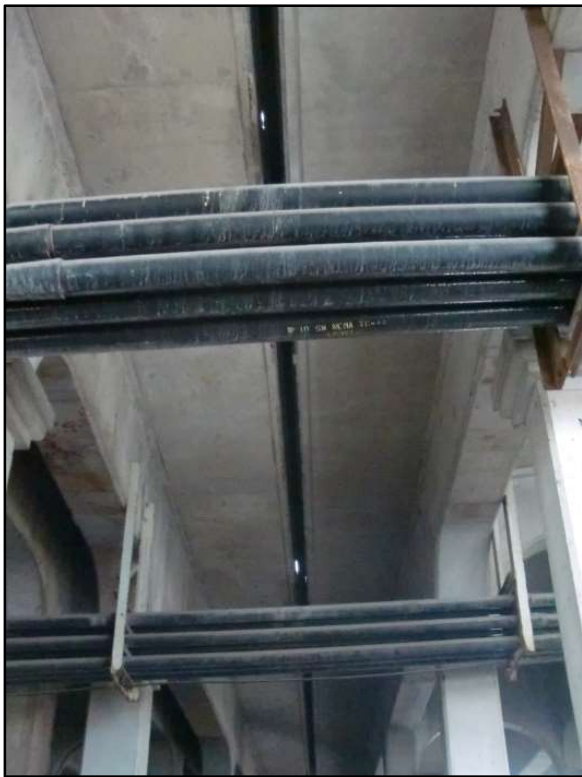
Photo 18 – Daylight Highlighting Two Broken Extrusion Welds, Tower B Expansion Joint.
