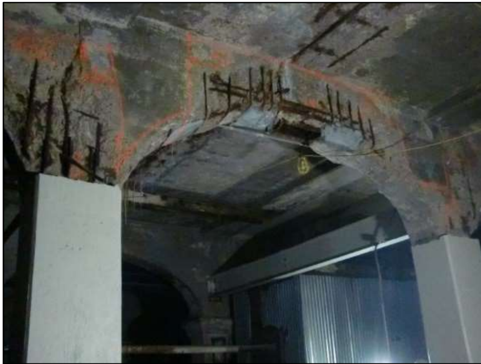
Photo 39 – Spalled Beam D21-D22, West Station.
