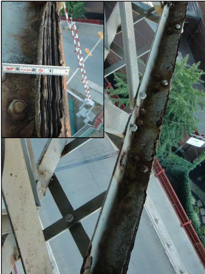
Photo 44 – Active Corrosion & Section Loss of Lower Lateral Bracing, Panel 3'.
