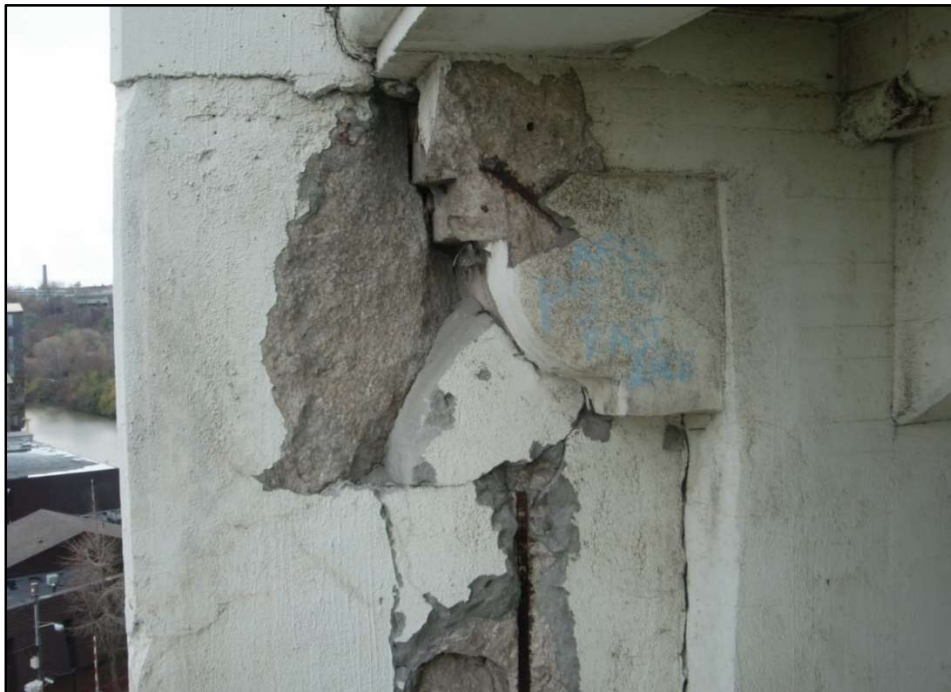
Photo 54 – Spalled & Loose Concrete Due to Ineffective Bond Breaker, Pier 5 Lower Deck Pier Shaft & South Lower Deck Corbel 1, Span 6.
