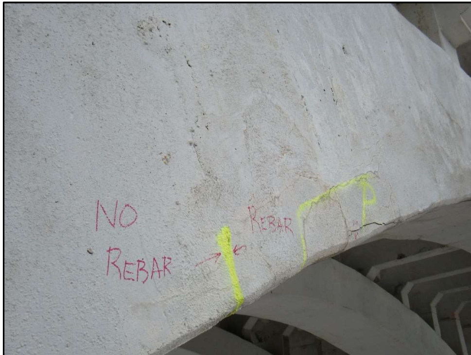
Photo 25 – Sound 1996 Shotcrete Patch (Left of Paint Line) & Cracked and Unsound Patch, Span 6 NE Arch Rib.
