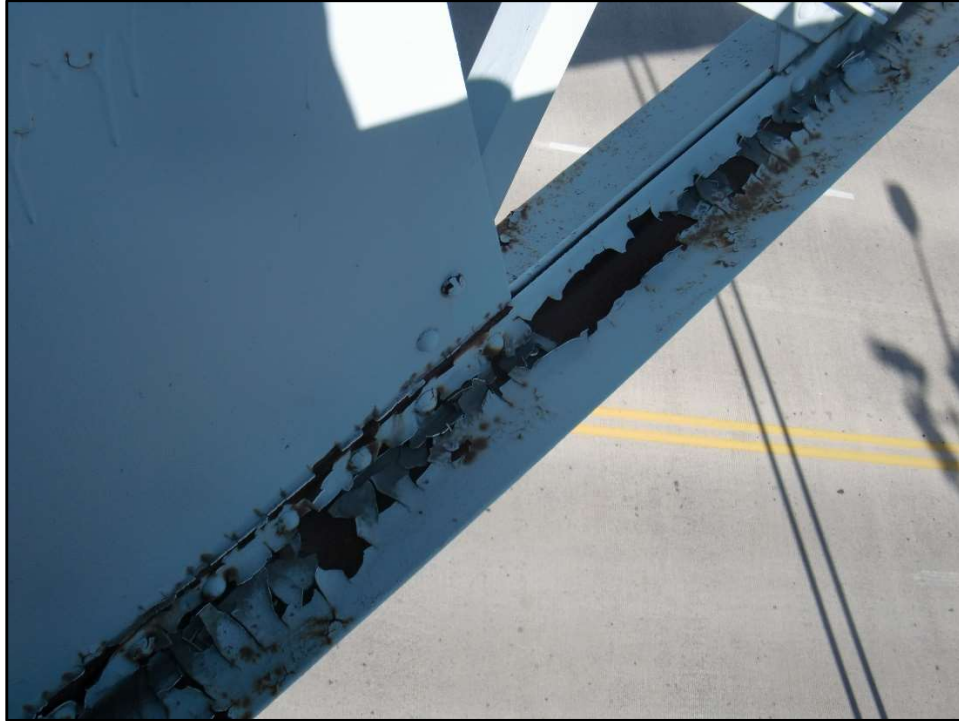
Photo 48 – Oxidized Top Coat & Peeling Paint Above Upper Deck.
