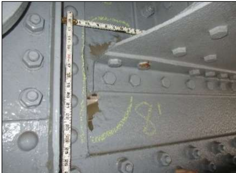
Photo 41 – Web Perforation on Upper Deck Floorbeam 8', Span 4.
