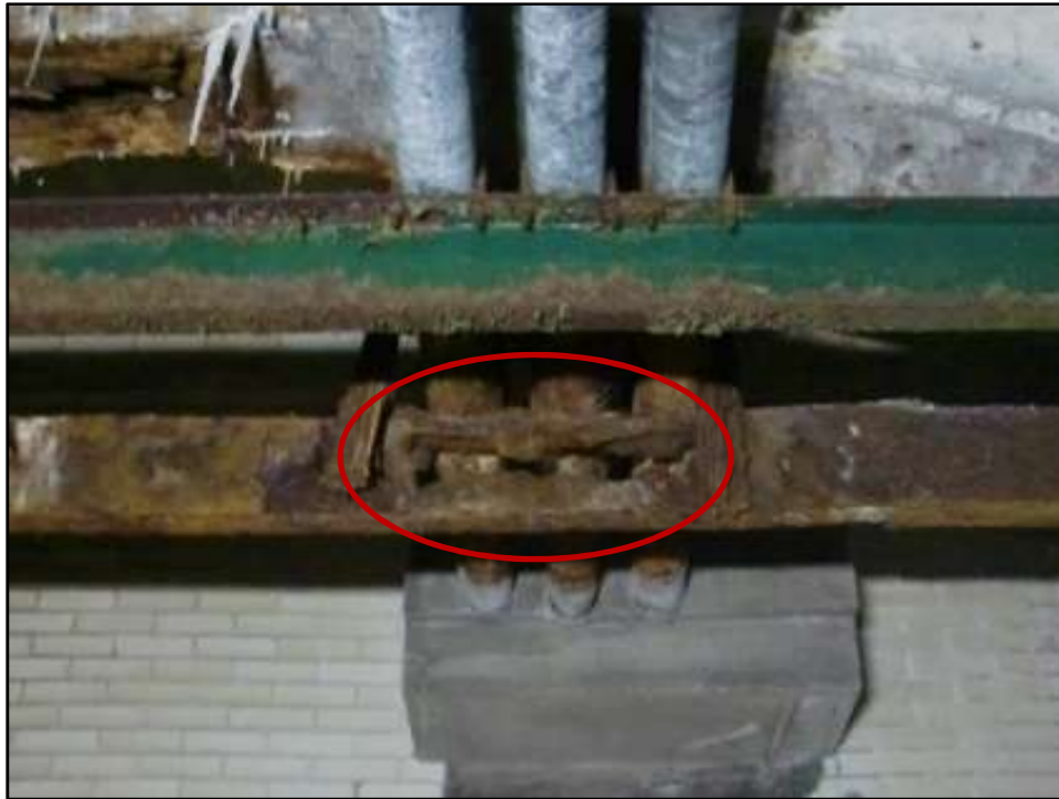
Photo 65 – Failing Utility Bracket (Channel Web Hole Circled), Panel A3-A4, West Station.
