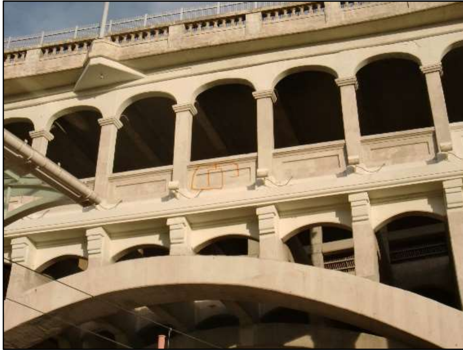
Photo 64 – New Graffiti Vandalism, Span 11, North Face.
