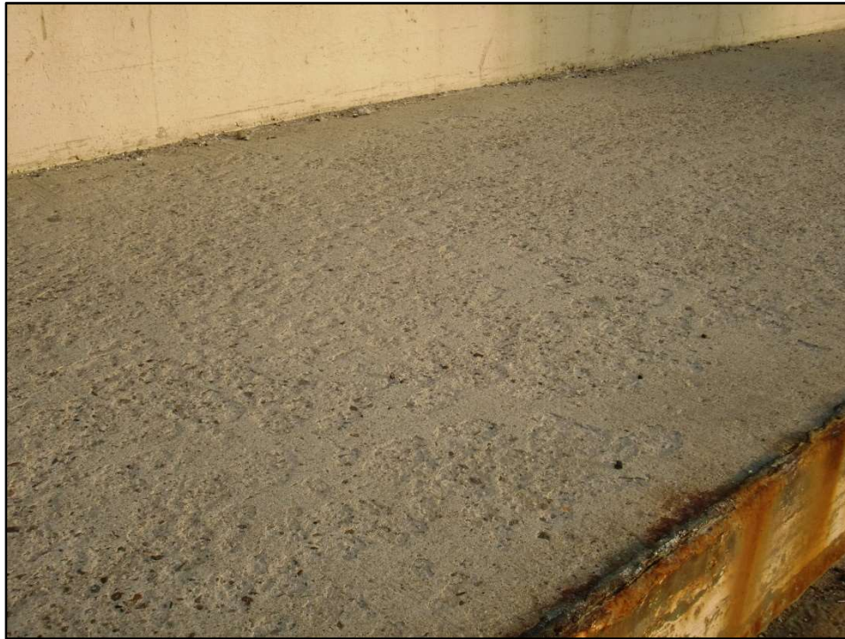
Photo 9 – Scaling of Lightweight Sidewalk Concrete, Span 4 South Sidewalk.
