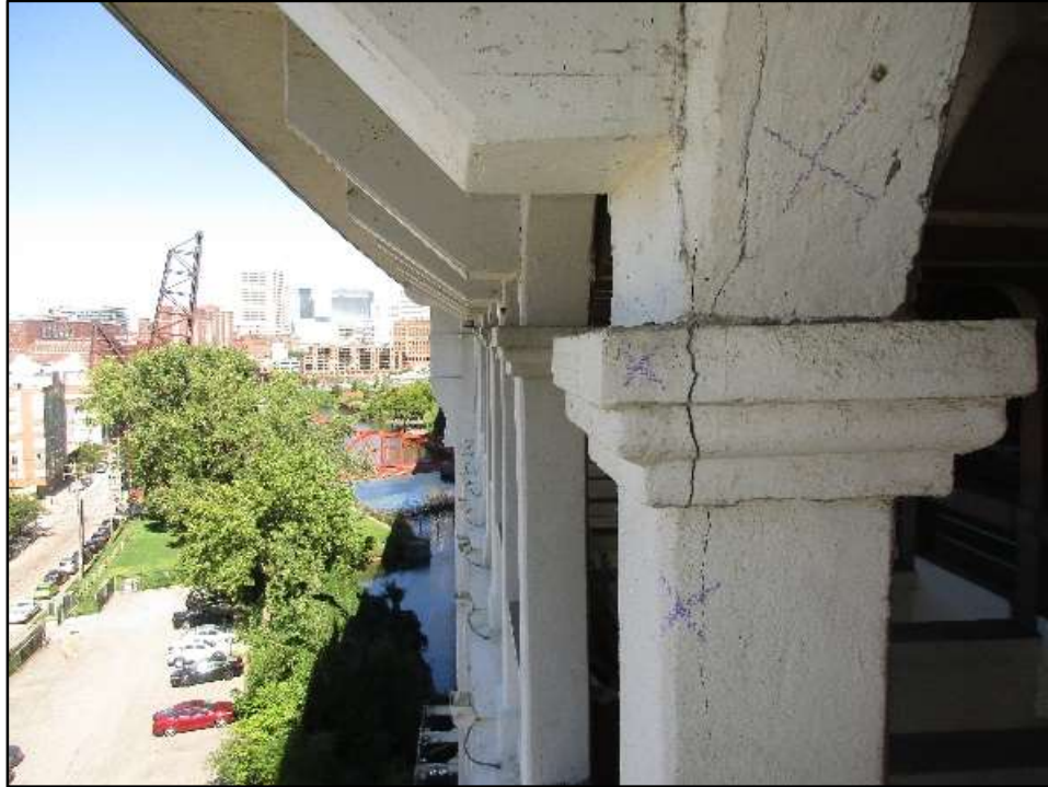
Photo 27 – Cracked Capital & Column Corner, NE Column 10, Span 3.
