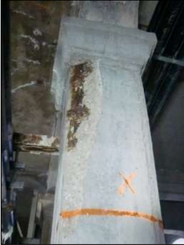
Photo 29 – Corner Spall with Corrosion to Epoxy Coated Reinforcement, Column D3, West Station.
