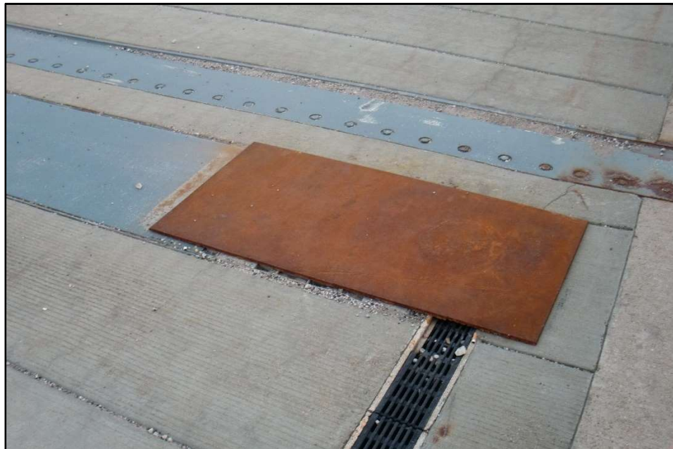
Photo 15 – Steel Cover Plate over Missing Sidewalk Drain Grate, Span 3.
