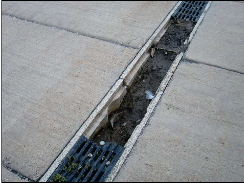
Photo 14 – Missing Sidewalk Drain Trough Cover with Debris Build-Up, North Sidewalk.
