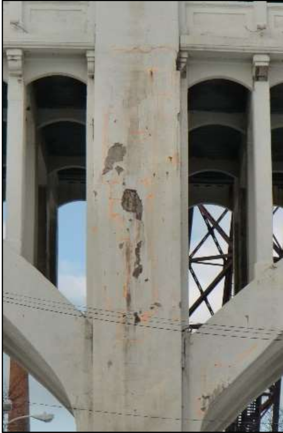
Photo 53 – Deeply Scaled & Delaminated Area (Highlighted in Paint), SE Lower Deck Pier Shaft, Pier 6.
