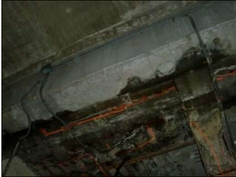
Photo 35 – Delaminated & Spalled Surfaces of Upper Deck Floorbeam 31, between Lines B & C and below Tower A Expansion Joint. (Note: This floor beam was cast during the 1995 rehabilitation.)
