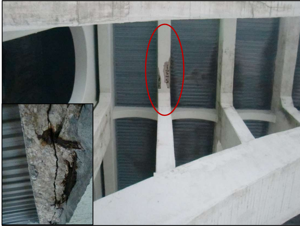
Photo 37 – Loose Concrete (Circled) over Parking Lot Removed, Lower Deck Floorbeam 2, Center Bay, Span 5. (Inset: Active corrosion of reinforcement steel present.)
