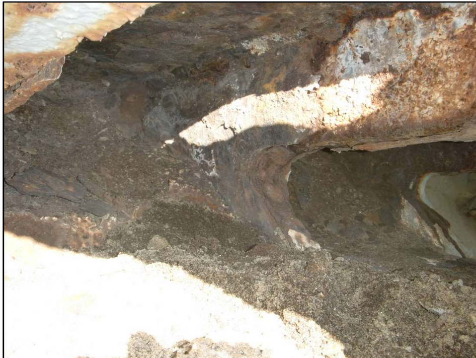
Photo 46 – Typical Steel Shot Blast Material & Corrosion within Truss Bearing.
