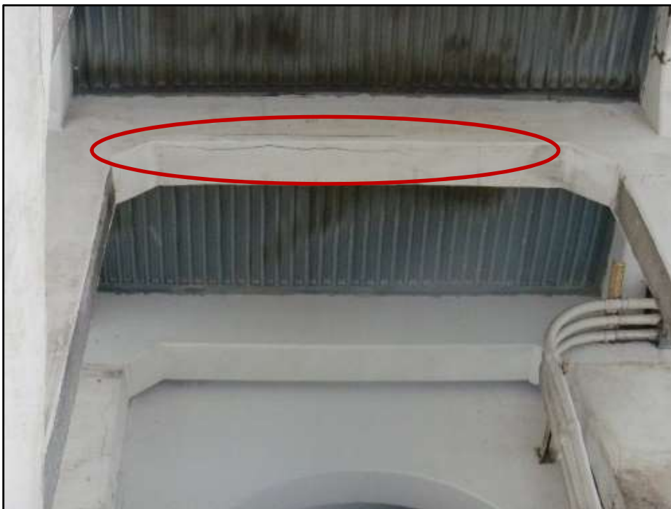
Photo 36 – Common Cracked & Delaminated Lower Deck Floorbeam Surface (Circled).
