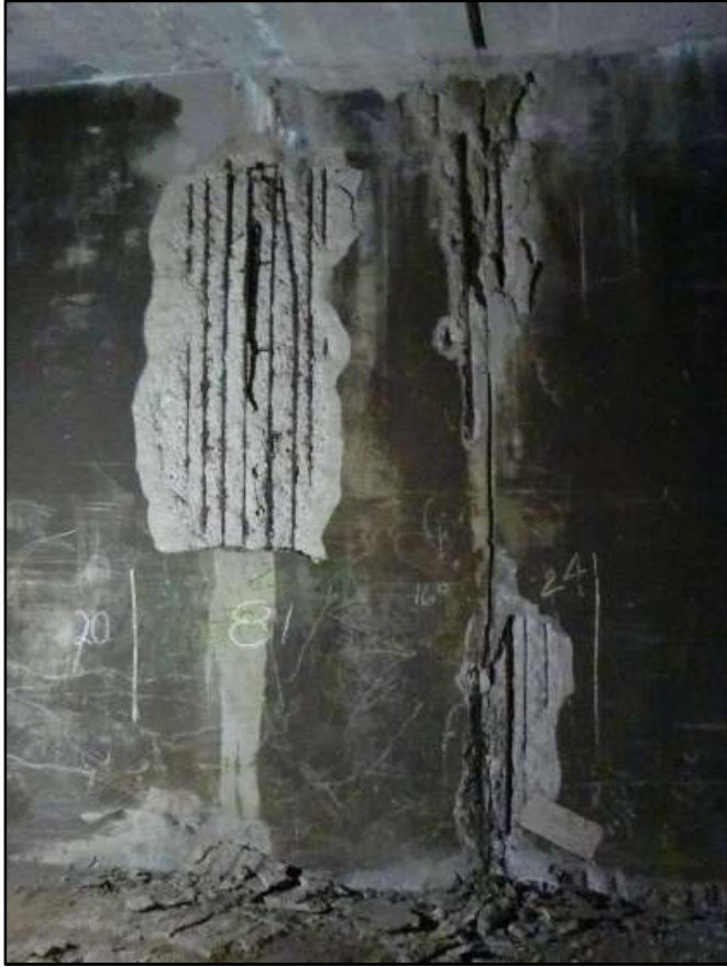
Photo 50 – Deep & Slow-Growing Spalls on Wall Joint, West 25 th Street Tunnel.
