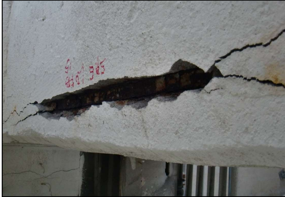
Photo 24 – Outline of Delaminated Arch Rib Corner, SI Arch Rib, Span 7. (Inset: Active rebar corrosion present.)
