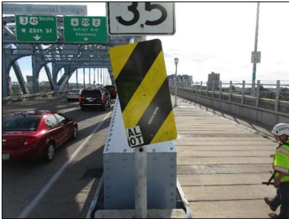
Photo 61 – Misaligned Chevron Sign, East End of Span 4 North Truss.
