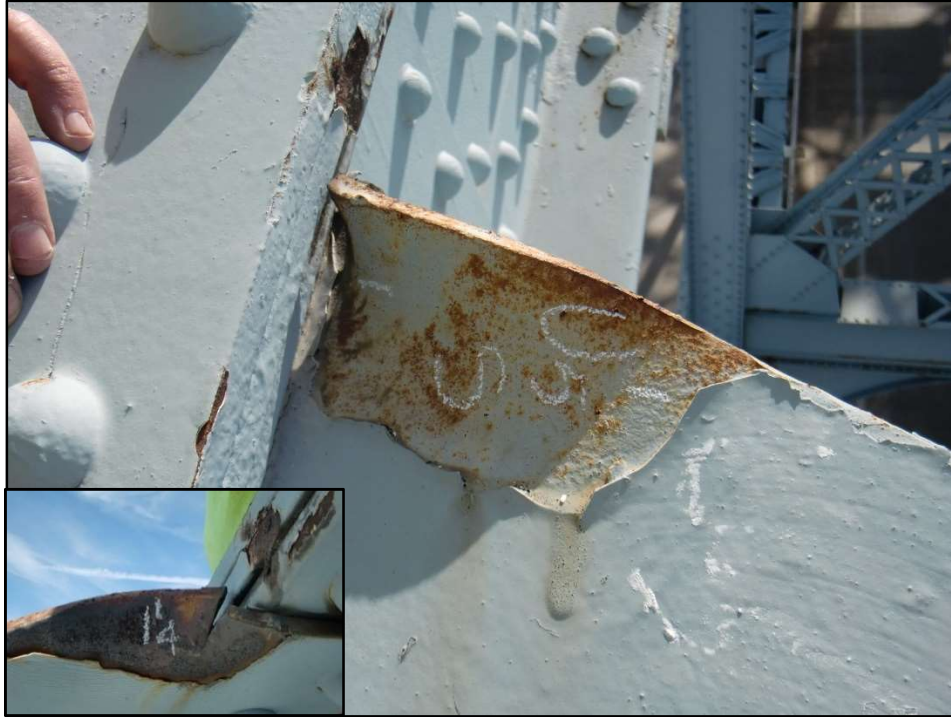
Photo 45 – Upper Lateral Gusset Plate Tear at Panel Point U 5 '. (Inset: View of tear looking up.)
