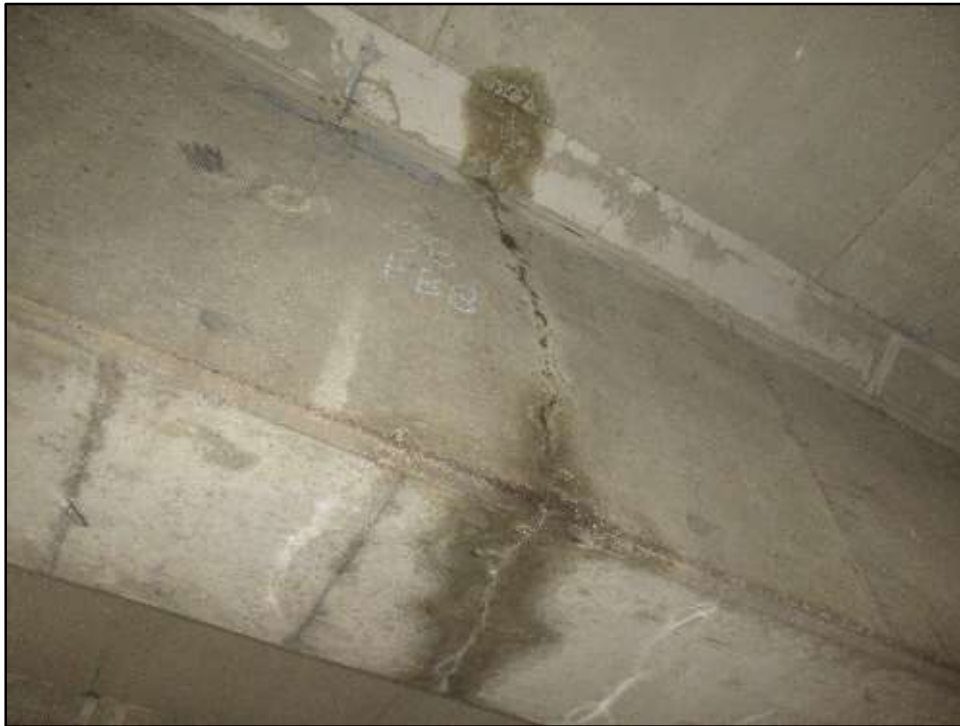
Photo 6 – Active Infiltration Through Upper Deck Floor, Floor Beam 8, Center Bay, Span 8.
