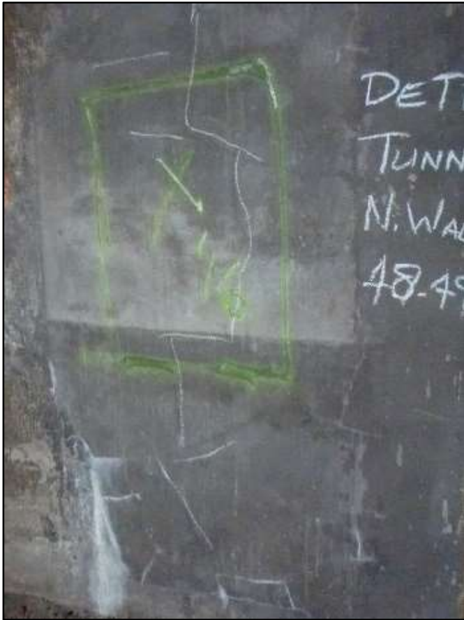
Photo 52 – Delaminated Area (Highlighted in Paint) on New Wall Patch, Detroit Avenue Tunnel.
