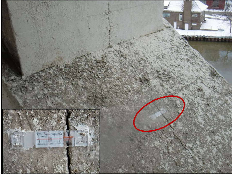
Photo 22 – Crack Monitor Set Across Vertical Arch Rib Crack, NE Arch, Span 5. (Inset: Close-up of Crack Monitor installed December 23, 2016.)
