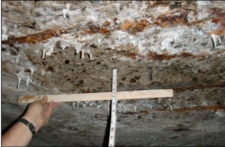
Photo 5 – Floor Spall with Infiltration, Bay C25, West Station.
