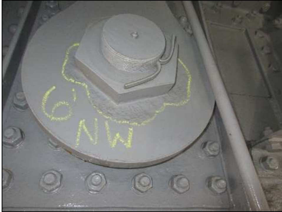
Photo 49 – Common Minor Pitting on Hangers Below Upper Deck Pin.
