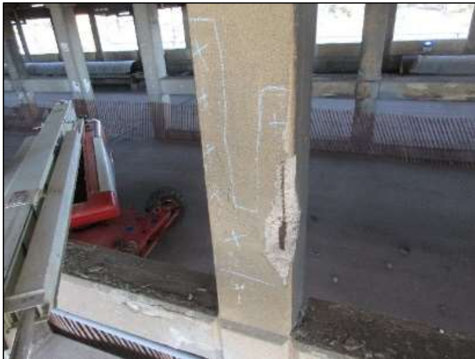
Photo 28 – Occasional Delamination & Spall of Original Upper Deck Columns.
