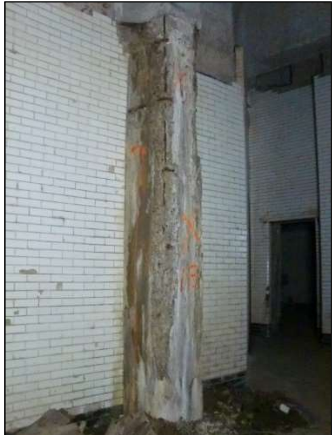
Photo 30 – Advanced Deterioration to Column G18, East Station.
