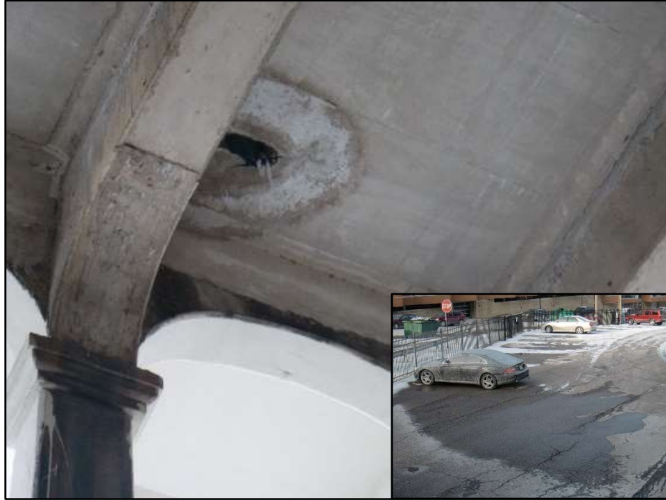
Photo 16 – Leaking Sidewalk Subdrain, Span 3 North Exterior Column Line. (Inset: Salt spray on car in private parking lot below.)
