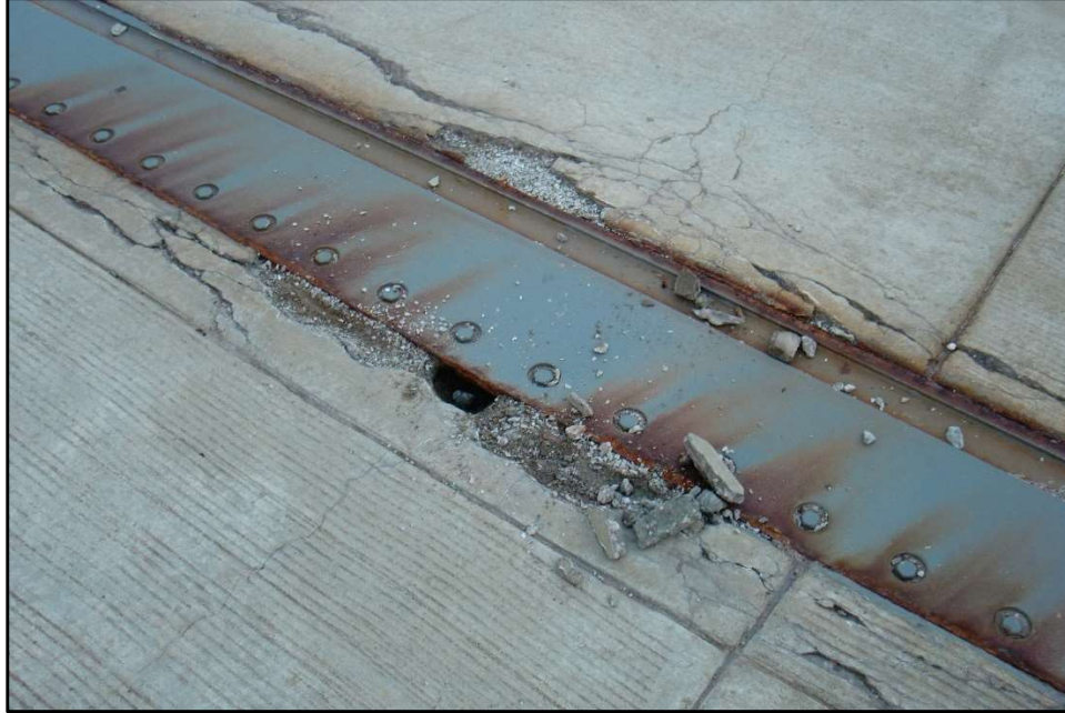
Photo 19 – Spalled Concrete Beneath Joint Armor, Pier 4, North Sidewalk.
