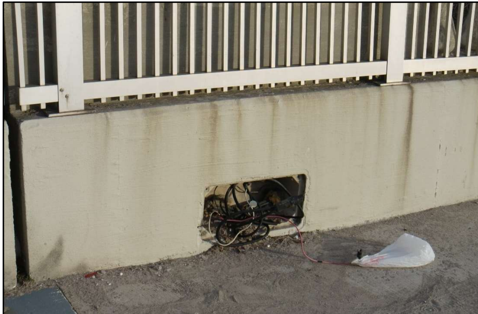
Photo 21 – Missing Junction Box Cover, Span 1 South Rail.
