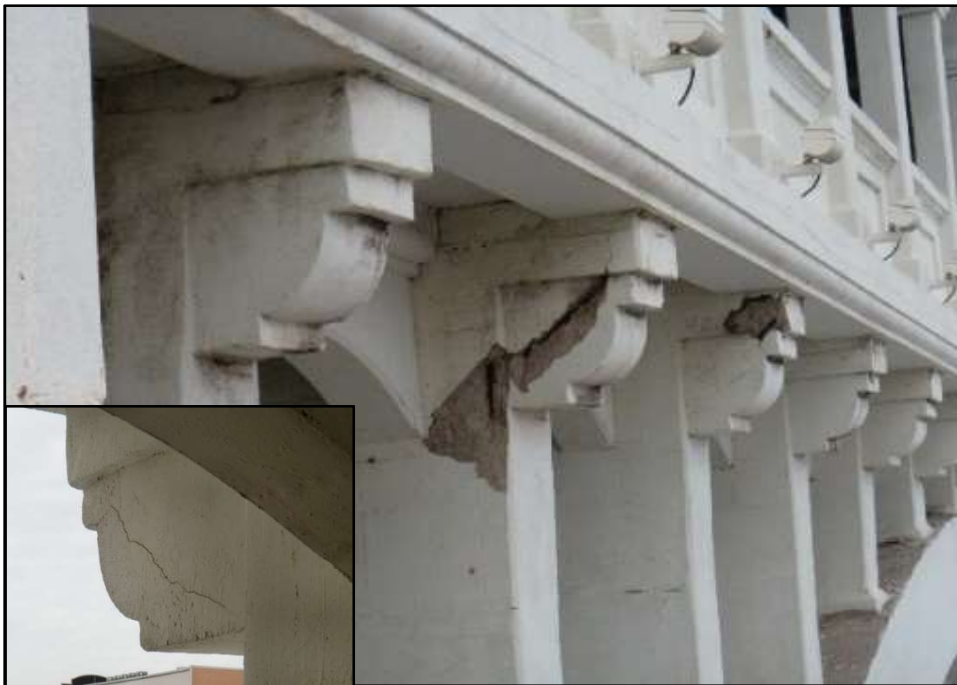
Photo 38 – Common Spalls on Lower Deck Corbels. (Inset: Diagonal crack indicating concrete corrosion present.)
