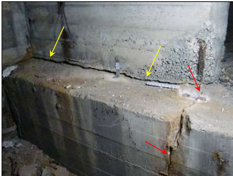
Photo 56 – Tower B Footing Crack (Highlighted with Red Arrows), and Footing Rotation & Drop with Respect to Transverse Wall (at Yellow Arrows), Looking South.
