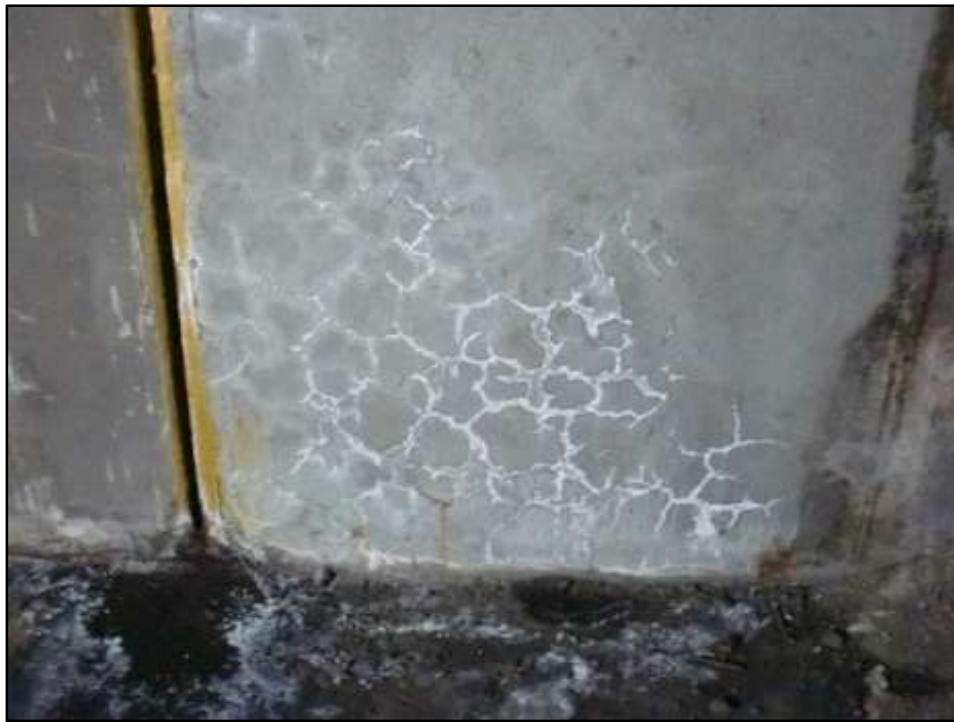
Photo 51 – Hairline Cracks on New Wall Patch, Detroit Avenue Tunnel.
