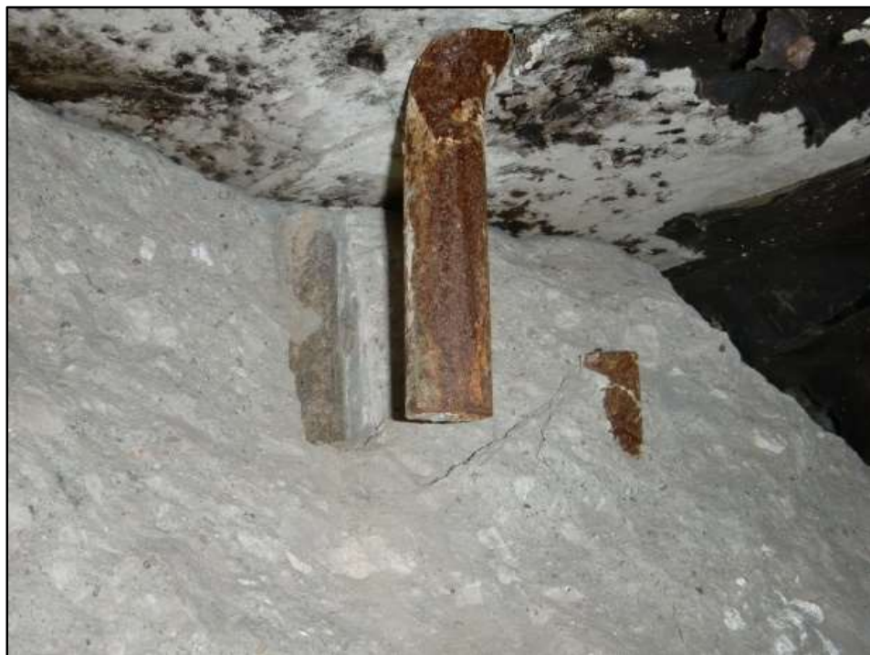
Photo 58 – Four-Inch Movement of Embedded Pipe Between Tower B Wall Shaft & Sidewalk Cantilever Above.
