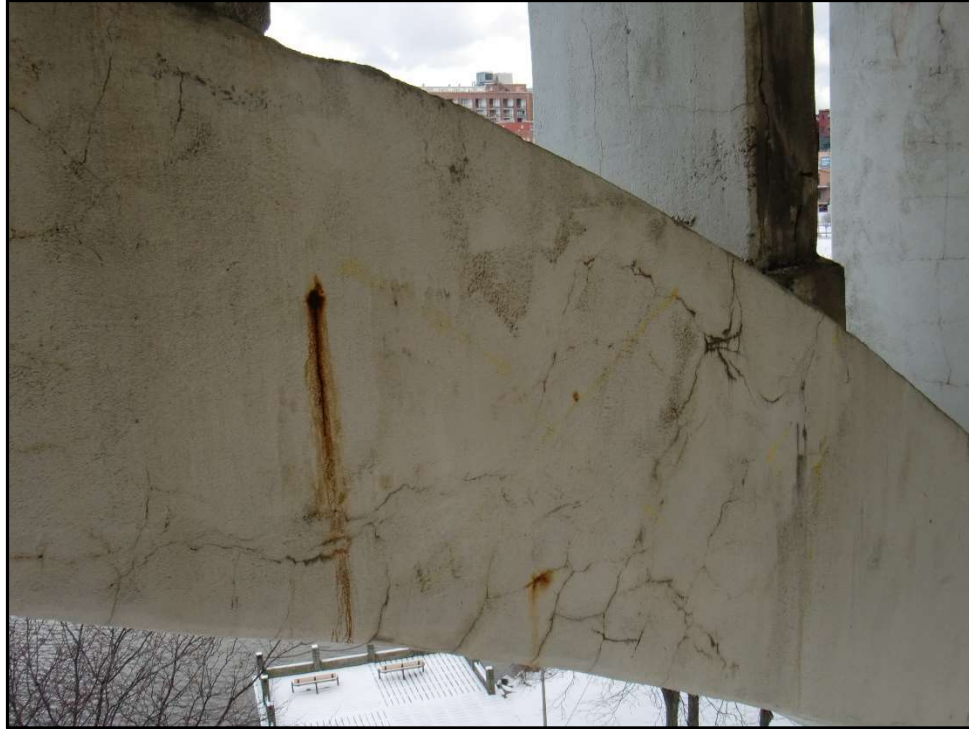
Photo 26 – Cracked Concrete at Location of 1915 Arch Repair, NE Arch Rib, Span 6. (Note: Rust staining likely from steel form connectors or discarded nails.)
