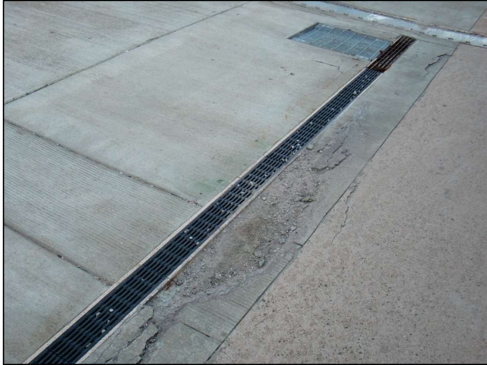
Photo 10 – Spalls Along Longitudinal Drain, 2003 Linear Park Sidewalk, Span 4.
