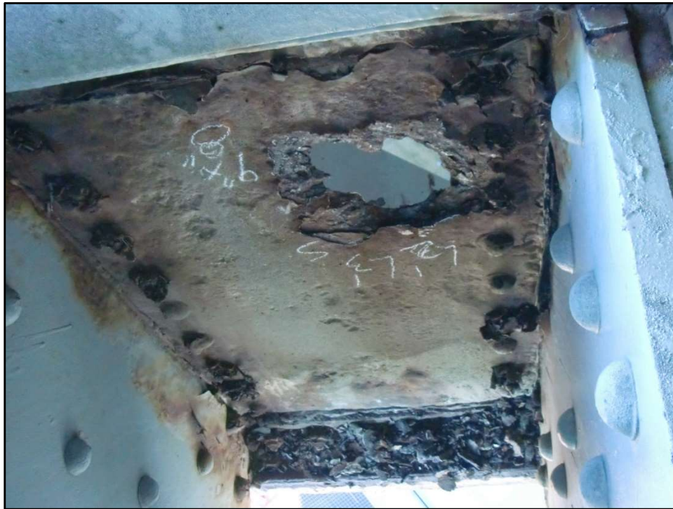
Photo 42 – Common Perforations of Lower Chord Diaphragm & Debris on Lower Transverse Angle.
