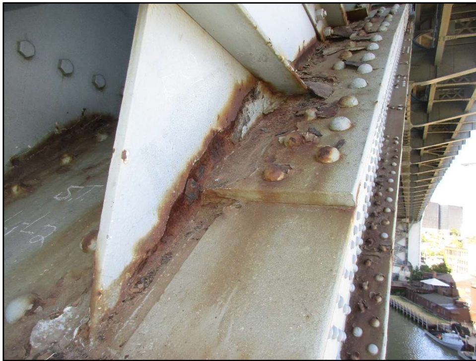
Photo 43 – Active Corrosion of Main Truss Gusset Plate above Lower Chord, Panel Point L2, South Truss.
