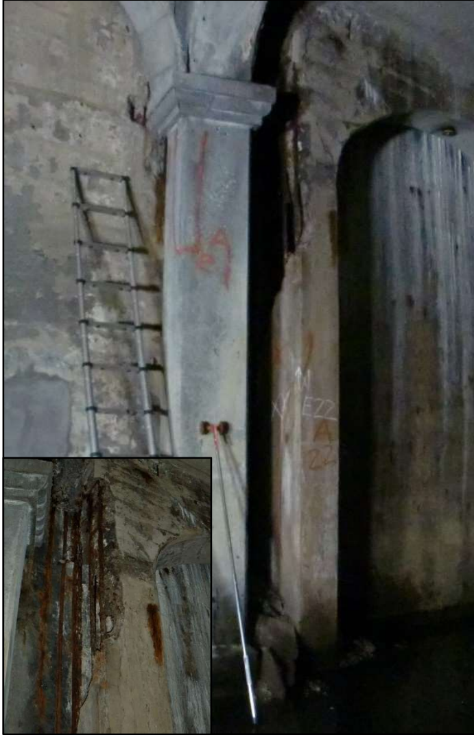
Photo 31 – Advanced Deterioration of Column M22, East Subway. (Inset: Exposed Reinforcement at top of column with 60% section loss.)
