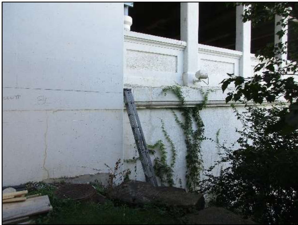
Photo 63 – Step Ladder Used for Vandal Access to Lower Deck, Span 13, North Face.
