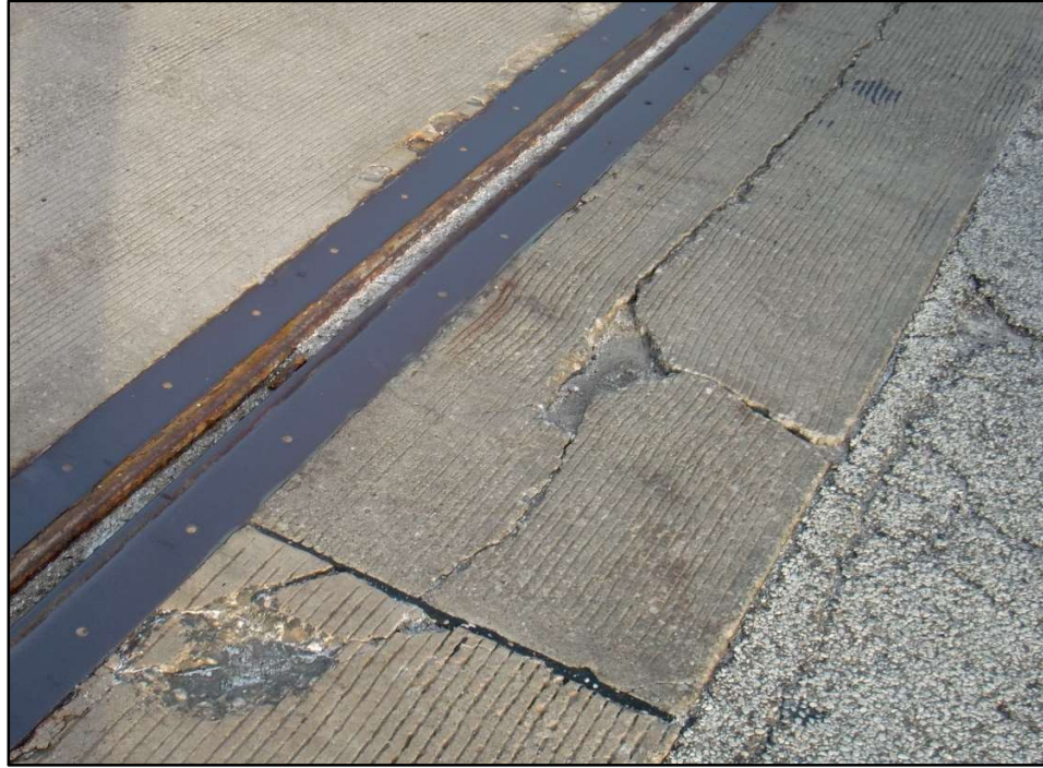
Photo 17 – Cracked Concrete Anchorage, Tower A Expansion Joint.
