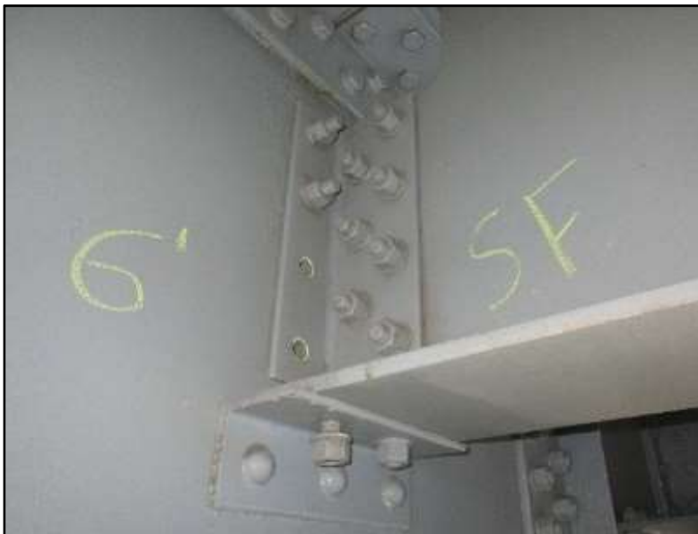
Photo 40 – Missing Bolts at Lug Connection, Stringer F, Panel 6'.
