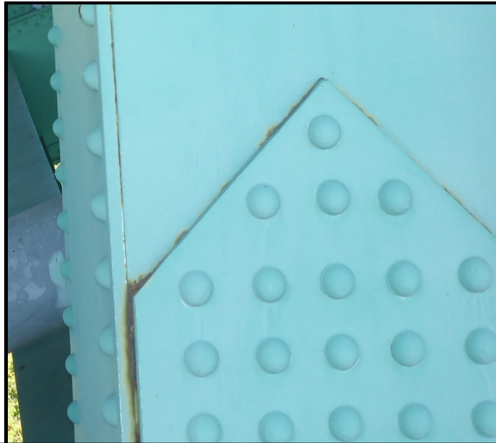
Photo 26 – Pack rust forming between plates of the Arch Column
