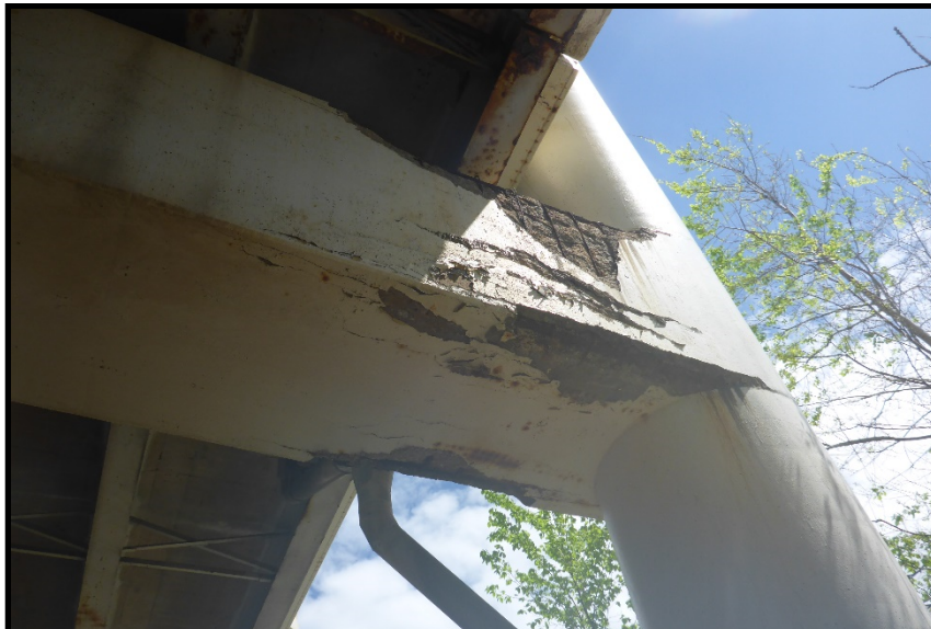
Photo 22 – Spalls with deteriorated rebar on bottom of Pier 13
