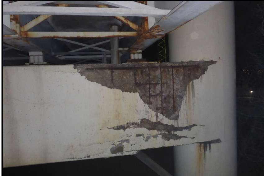
Photo 21 – Spalls with deteriorated rebar near end of Pier 13 cap
