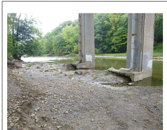
Photo 4 Drainage troughs at bases of Pier 6 columns. Localized scour that was occurring last inspection seems to have stabilized and is not progressing.
