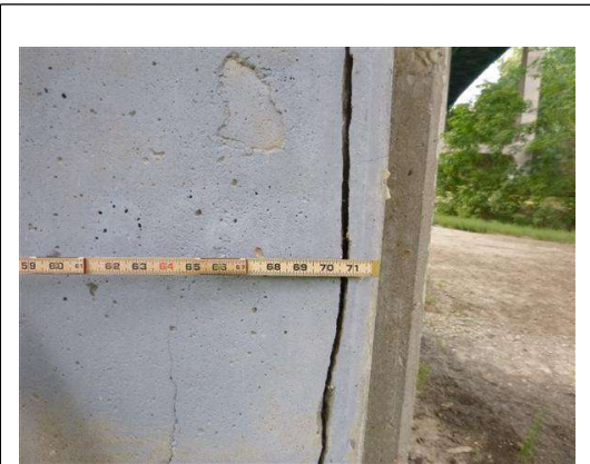
Photo 3 Corner crack on a pier column (wider than typical).
