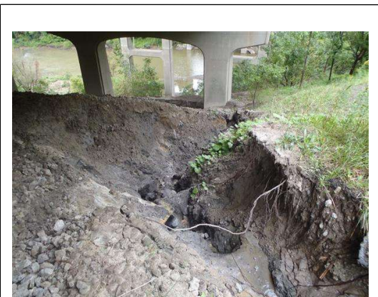
Photo 5 Erosion trough extending down East Abutment slope, getting deeper.
