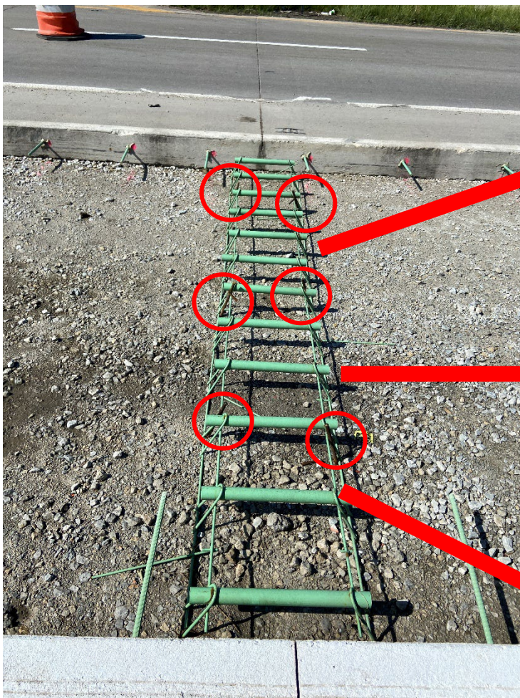
Lack of pins at basket assembly
