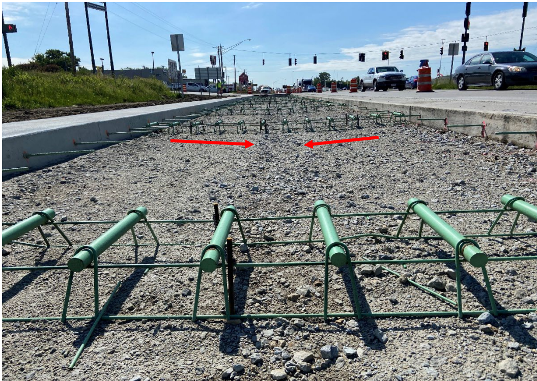
Inverted slope on 304 aggregate
