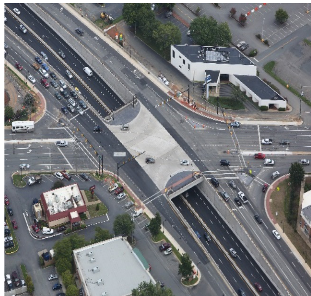
VADOT Route 29 Urban Corridor. LANE reached a significant project milestone by opening a grade-separated interchange seven (7) weeks ahead of schedule
