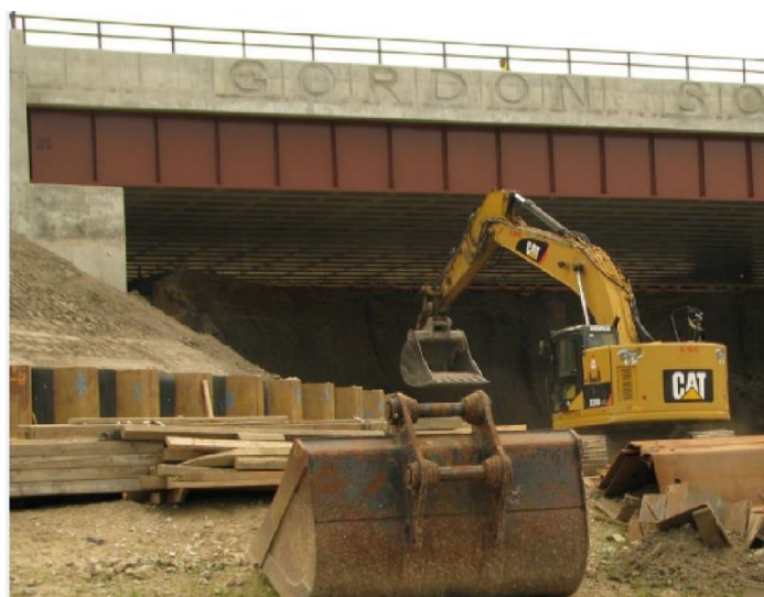
Figure B-3 – Excavation of W. 73rd St. under NS – Baker designed bridge using top-down construction approach
