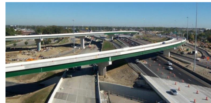
Figure A-4 – Kokosing utilized Quality Checklists and Hold Points for all major operations on the I-670/71 Columbus Crossroads Project
