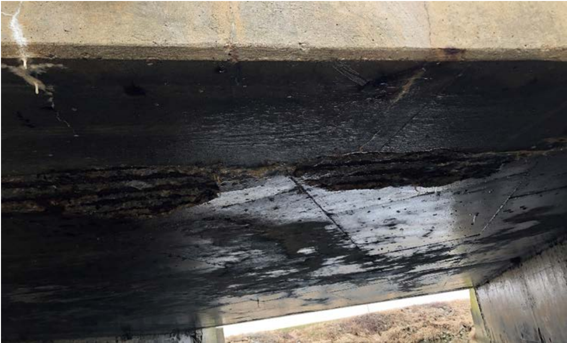
Photograph 2: Spalling of Bridge Deck with Reinforcing Steel Exposed
