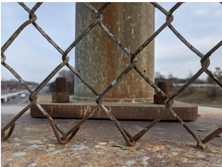
PHOTO 6 View looking east at lamp post. No gasket material on the underside of flange.
