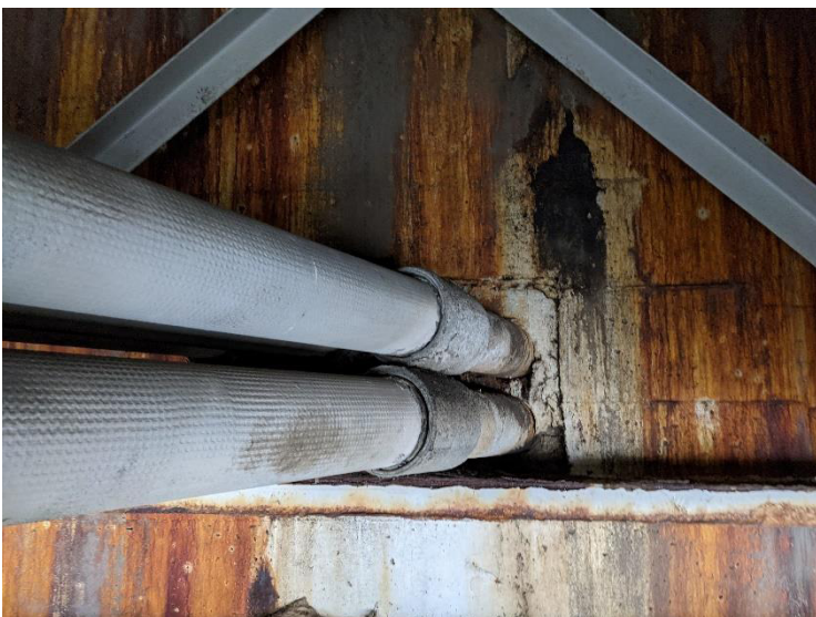
PHOTO 3 Looking north at underside of bridge. A bank of six 5" Transite conduits present. Assumed to be ACM. A verification sample taken at damaged coupler.
