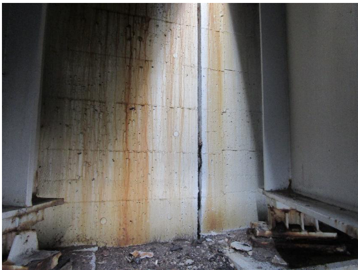
PHOTO 8 View looking at northside of backwall. Sample of expansion joint taken
