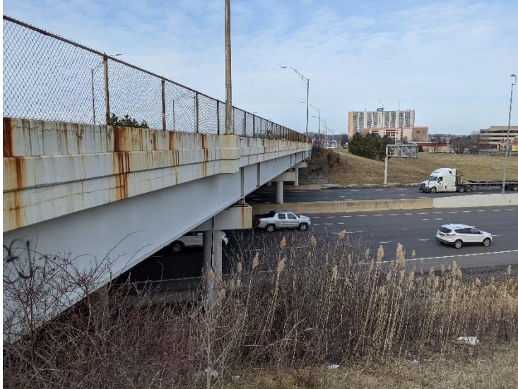
PHOTO 7 View looking north at the east side of the bridge showing vandal fencing, parapet railing, and light poles.
