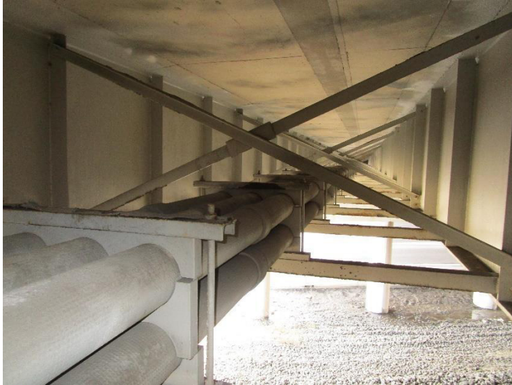
PHOTO 4 View looking south at underside of bridge and Transite conduit bank running the length of the bridge.
