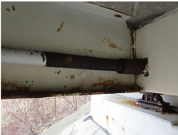
PHOTO 5 External pipe wrap around 4" PVC conduit at north beam. Sample taken here.
