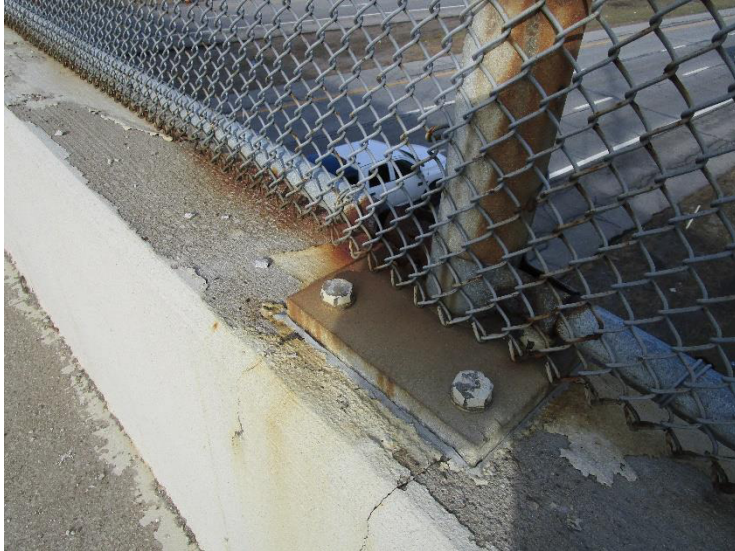
PHOTO 7 Vandal fence mounting flange. Caulking samples taken here.
