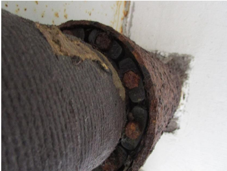
PHOTO 4 Internal mastic packing in coupler. Sample taken here.
