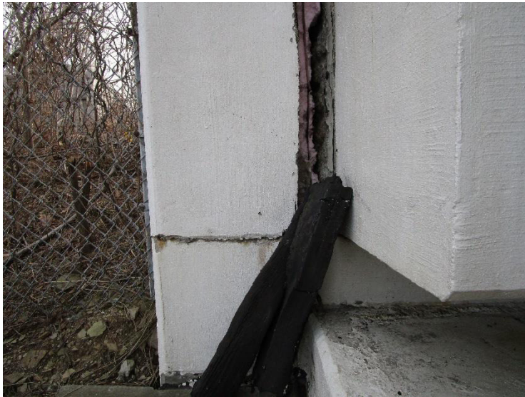
PHOTO 2 Looking at the north end east abutment 4"x4" mastic sealant. Sample collected here.
