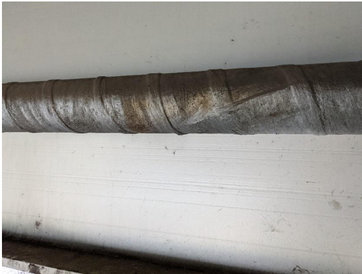
PHOTO 2 Looking at pipe wrap over 4" gas line affixed to the underside of the structure. Sample collected of wrap material.
