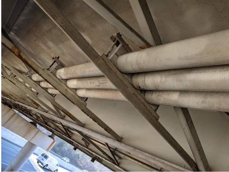
PHOTO 4 View looking at underside of structure. Bank of 3 Transite conduits are present.
