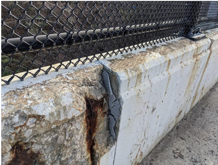
PHOTO 5 View looking at east wall parapet railing. Sample taken of joint caulking.
