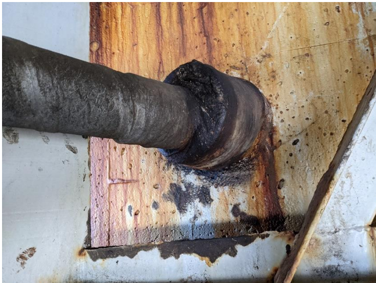
PHOTO 3 Gas line casing through backwall for 4 1/2" gas line. Sample taken of packing.
