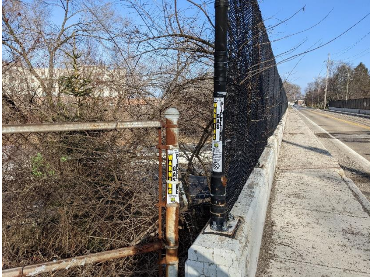
PHOTO 7 View looking north at the west side of the bridge showing fencing, sidewalk and gas line demarcation sign.
