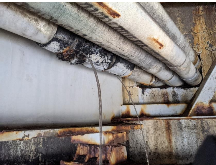
PHOTO 9 Bank of six PVC conduits on underside of structure.
