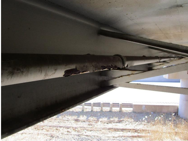
PHOTO 13 View of 6 5/8" O.D. gas line. Paint samples taken from here.
