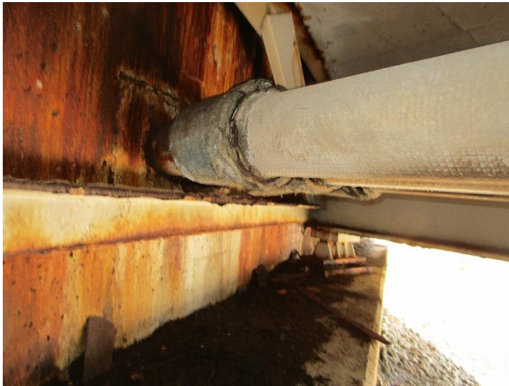
PHOTO 11 View looking at transite coupler. Sample taken here.
