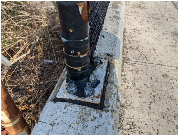
PHOTO 8 View looking down at vandal fence mounting flange. Joint caulking was sampled.
