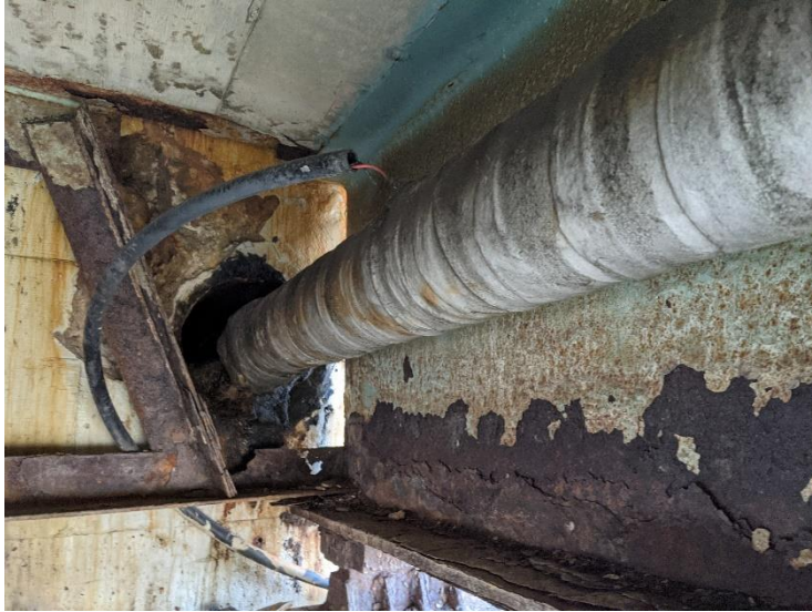
PHOTO 4 View looking at underside of structure. Samples taken at pipe wrap and mastic packing material.
