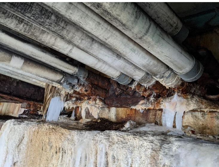
PHOTO 9 PVC pipe on underside of structure. Casings are rotted out.
