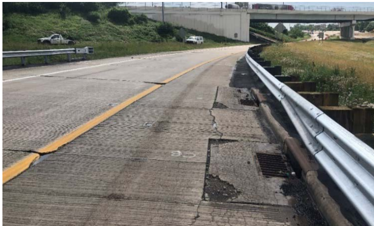
Photograph 10: Overall Pavement Condition of Ramp S-E
