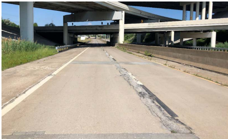
Photograph 3: Pavement Condition of IR-490 from Bridge No. CUY-490-0100 to the Eastern Project Limits
