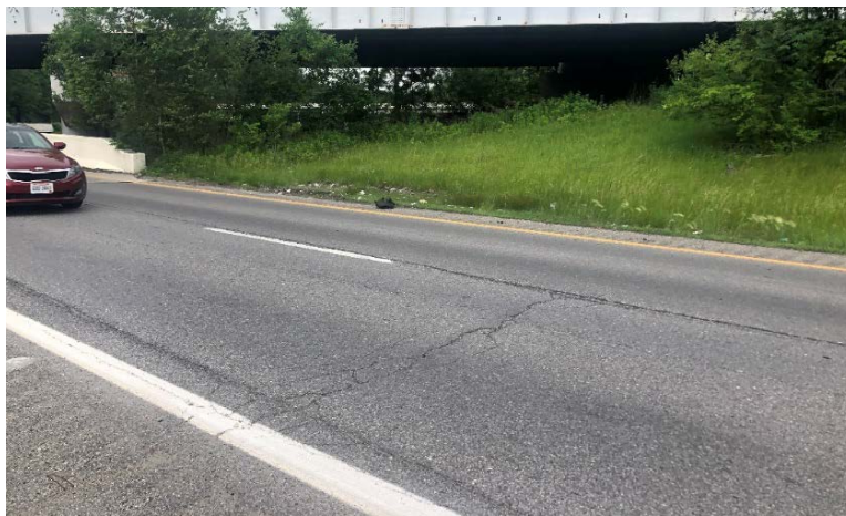
Photograph 5: Overall Pavement Condition of Lane E-S
