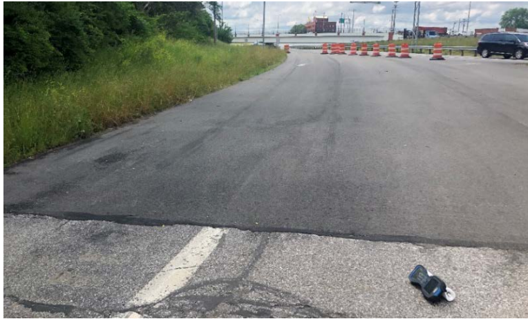
Photograph 12: Pavement Condition Transition of Ramp W-N
