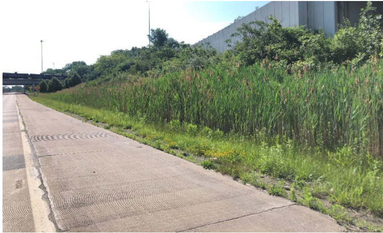
Photograph 4: Signs of standing water along IR-490
