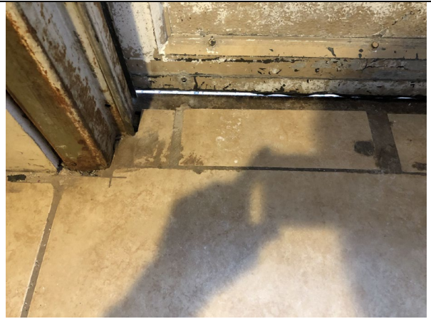
Photo 4: View of Tile Grout Located in the Operator's House
