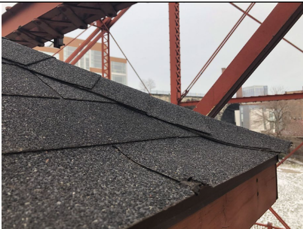
Photo 5: View of Roofing Shingles Located on the Operator's House
