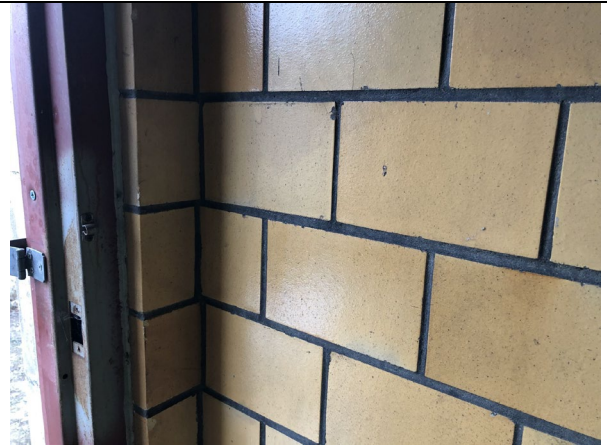
Photo 8: View of Yellow Tile and Grout in Bathroom of the Gateman's House
