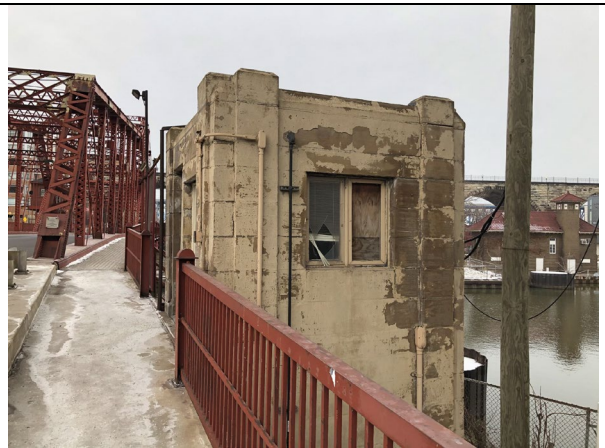
Photo 6: View of Gateman's House Located on the South Side of the Bridge
