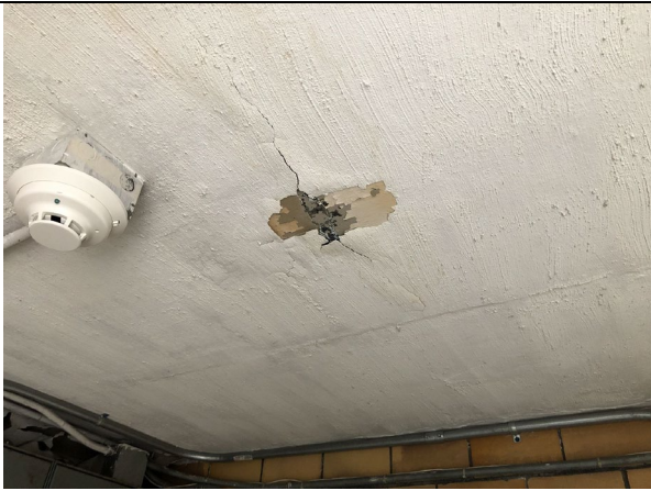
Photo 7: Skim Coat Located in the Office of the Gateman's House
