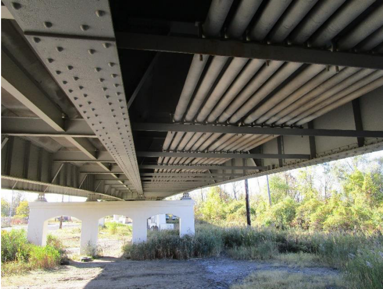
PHOTO 1 Looking south beneath the bridge at bank of PVC utility conduits
