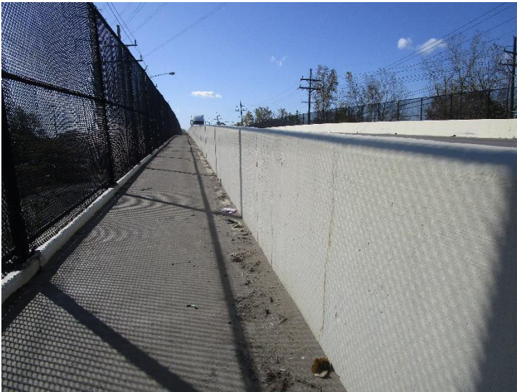
PHOTO 5 View looking at parapet, sidewalk, and vandal fencing along top of the deck.
