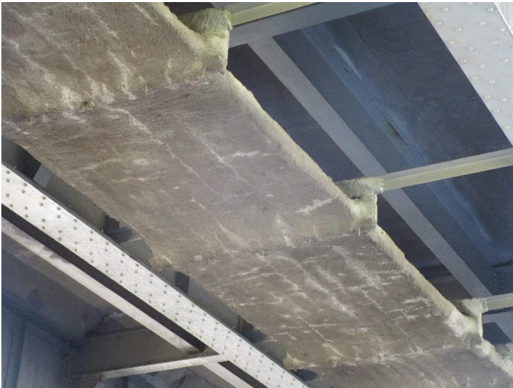
PHOTO 8 View looking up at pneumatically placed mortar (shot-crete) protection on utility conduits above railroad tracks.
