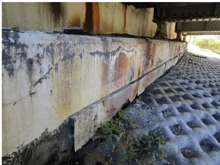
PHOTO 3 View looking at abutment and beam seats and grout filled slope protection matting.
