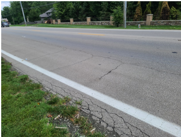
Photograph 1: SR-315 Pavement Wear
