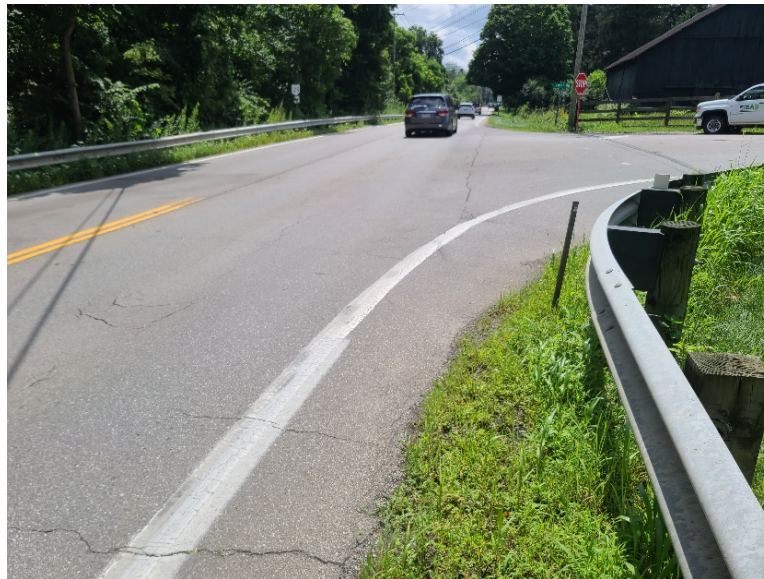
Photograph 2: SR-315 Pavement Wear
