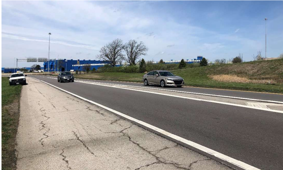
Photograph 1: Overall Pavement Condition of Exit Ramp
