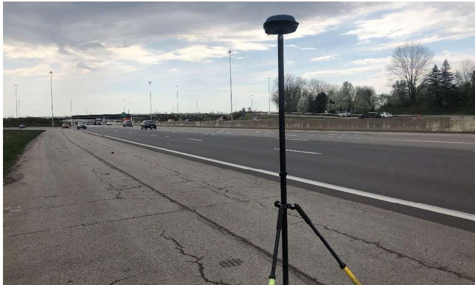
Photograph 3: Overall Pavement Condition of IR-71 NB
