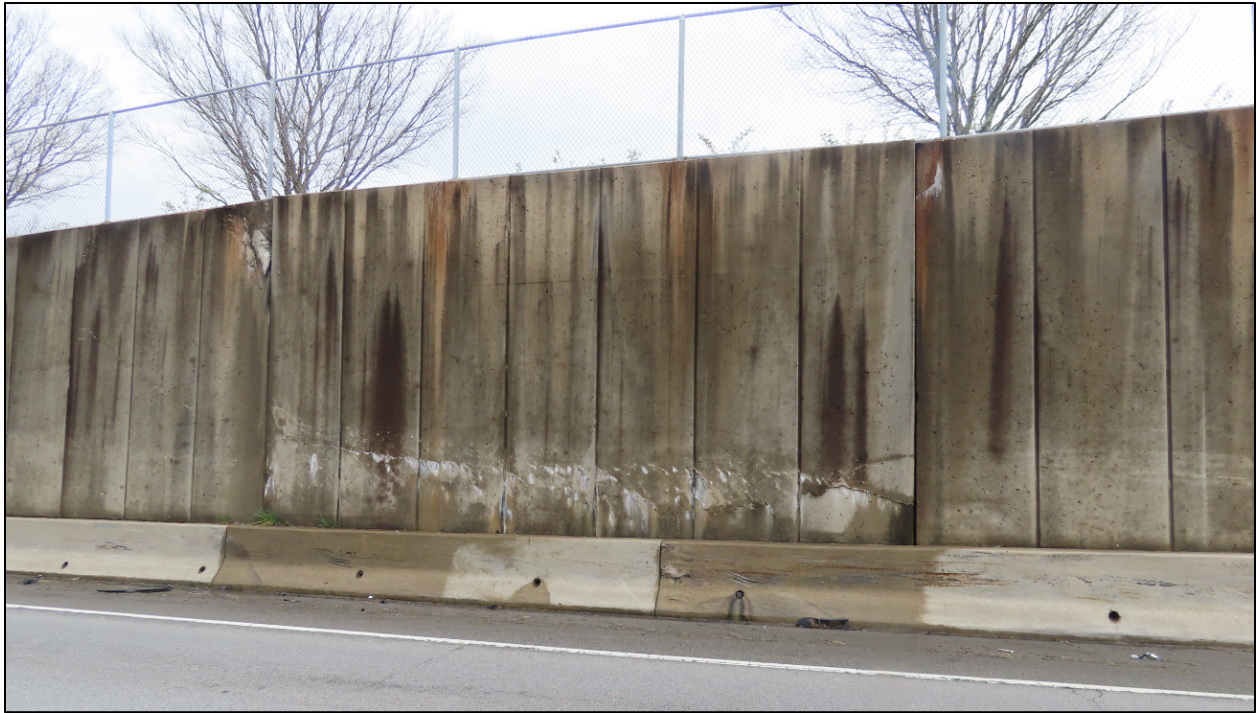
Figure 2: Photograph of Distressed Retaining Wall (from ODOT, looking from Ramp to Geier Drive)
