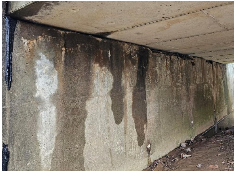
Photograph 2: Spalling and moisture intrusion around beam seat
