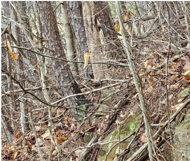
Photograph 5: Evidence of slope movement
