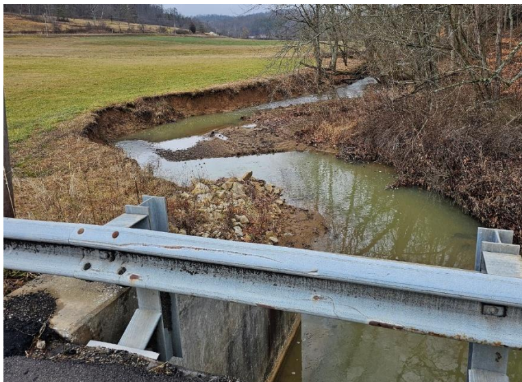
Photograph 3: Creek bank erosion
