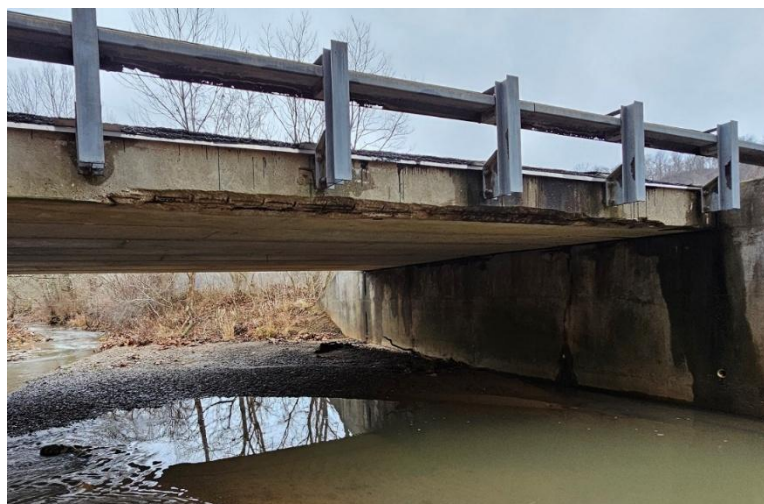
Photograph 1: Spalling and exposed steel on box beam
