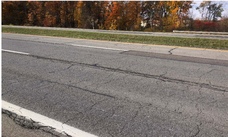
Photograph 1: Overall Pavement Condition of IR-680 NB
