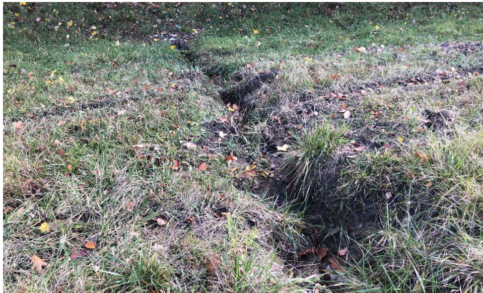
Photograph 5: Signs of Erosion at Drainage Basin Outlet
