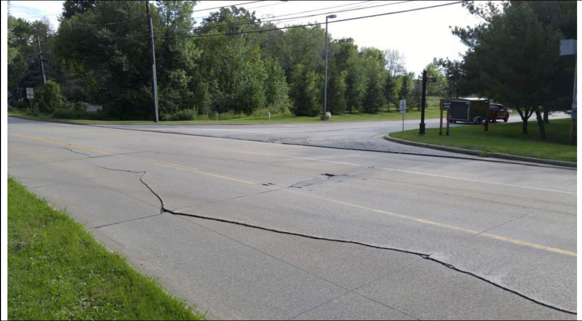
Photograph 35: Longitudinal crack along River Styx Rd near the creek to the east at ~Sta 912+00.
