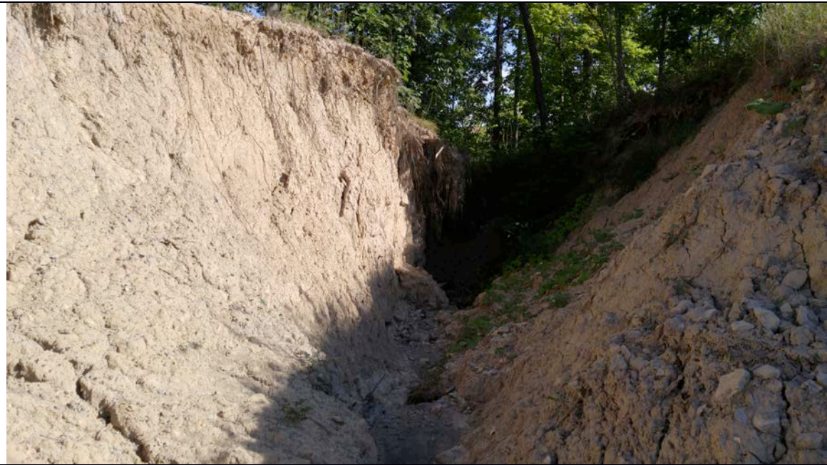
Photograph 22: Eroded channel at historical landslide near Sta 166
