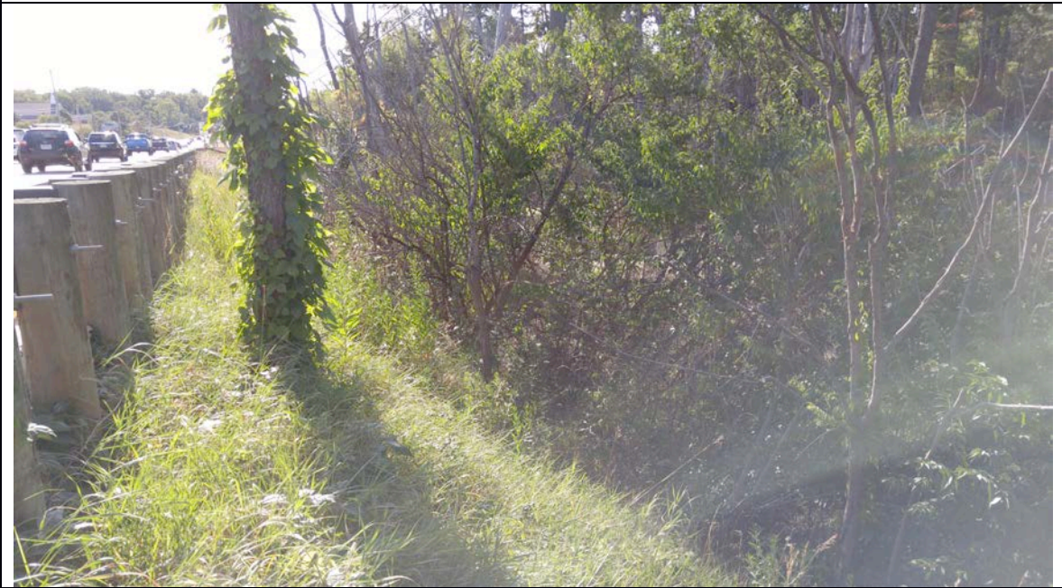
Photograph 20: Embankment at historical landslide near Sta 166
