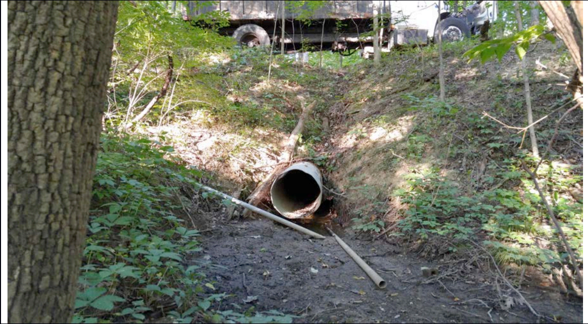
Photograph 27: View of culvert buried in sediment – northern Frontage Rd
