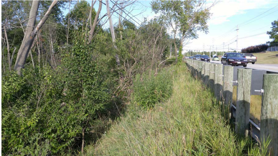
Photograph 7: Eroded channel at historical landslide near Sta 166+00
