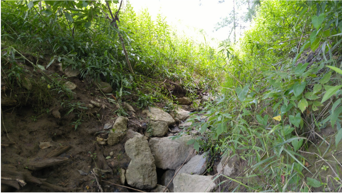
Photograph 3: Drainage ditches along proposed path.
