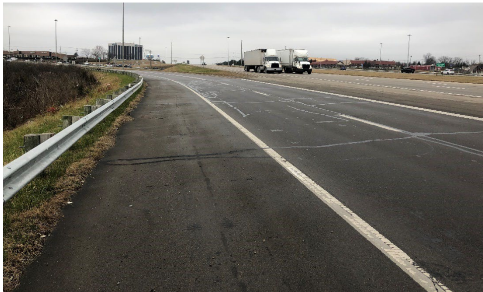
Photograph 11: Pavement Condition of Ramp D from where Ramp intersects with IR-75 to Northern Termination
