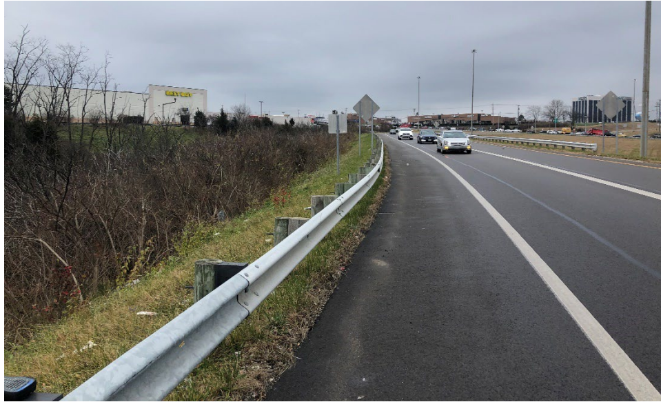
Photograph 10: Pavement Condition of Ramp from SR-725 to where Ramp intersects with IR-75
