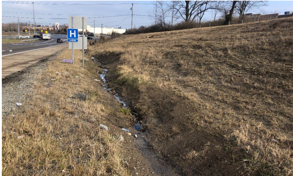
Photograph 9: Erosion Observed in Drainage Ditch past Eastern Shoulder of Ramp C
