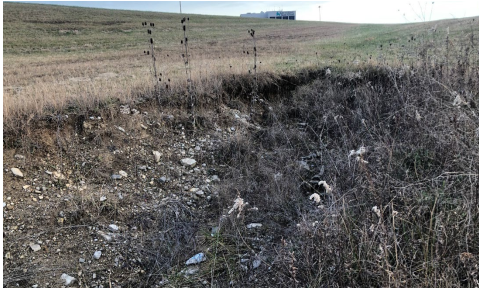
Photograph 6: Erosion Observed in Drainage Ditch encompassed by Ramp B and IR-75
