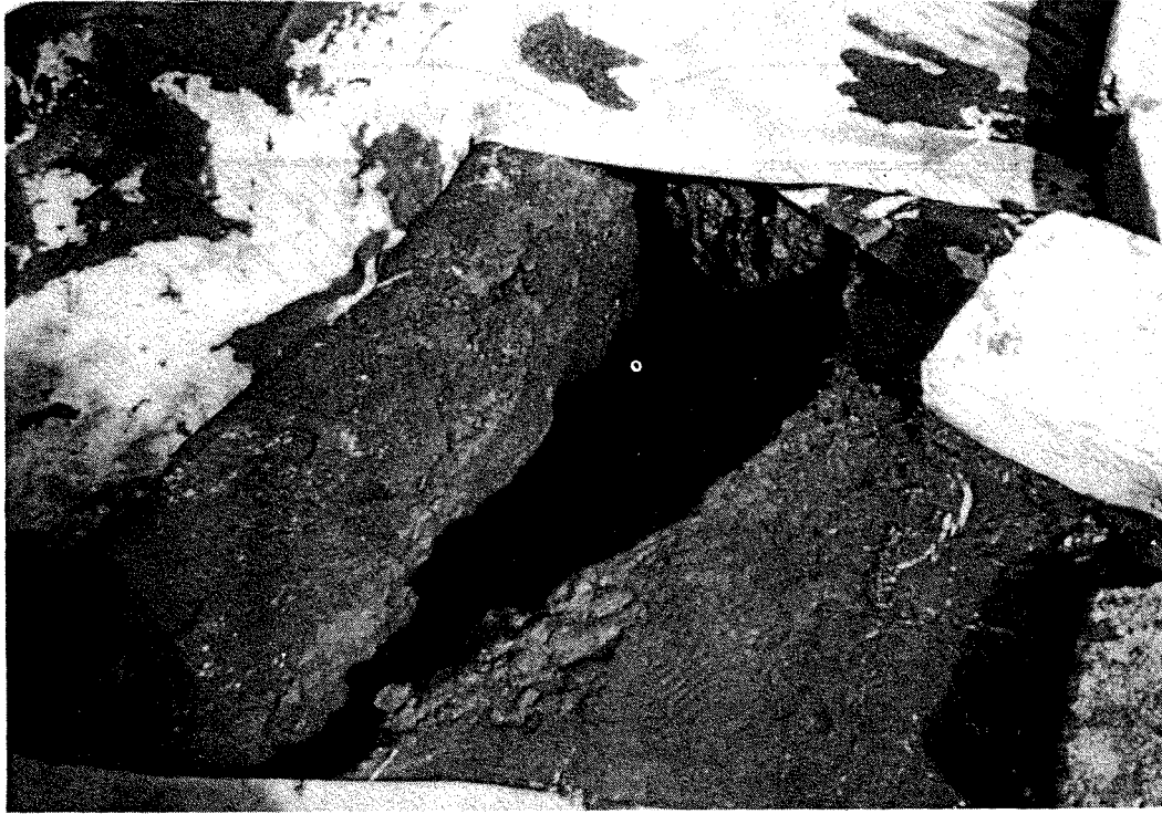
Fig. 2. Large tension crack formed under a geomembrane liner.
