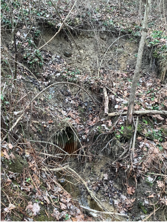
Photo 5 – UNT to Timber Run, slip material covering headwall to be removed, new headwall installed, pipe repaired, and RCP placed.
