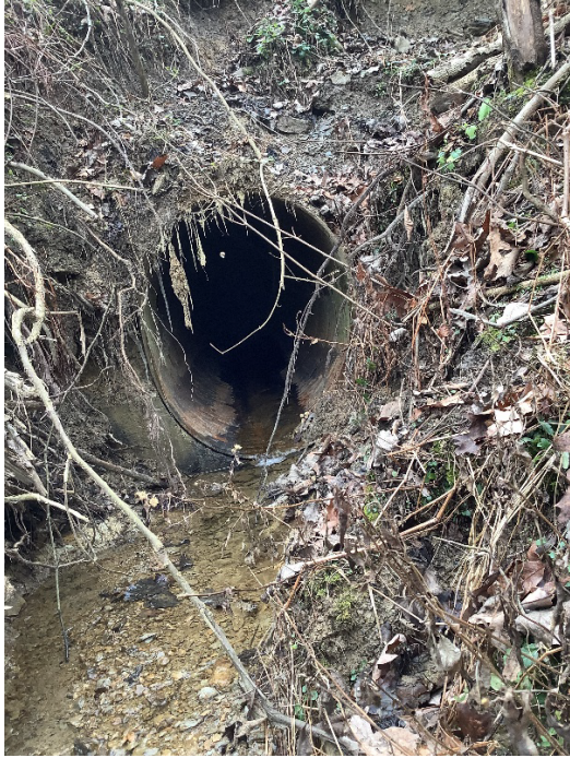
Photo 8 – compression of culvert due to material that has slipped
