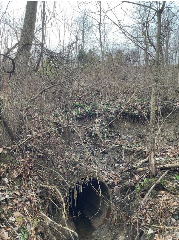
Photo 6 – Hillside uphill from culvert facing south toward IR-70, note slip material
