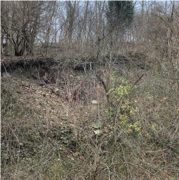
Photo 23 – Slip on hillside facing south toward IR-70
