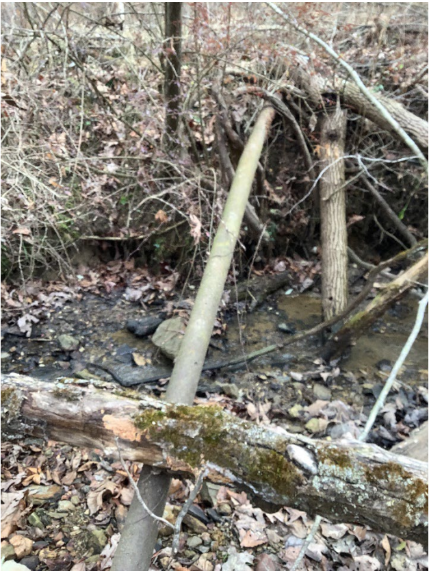
Photo 11- Corroded metal pipe crossing stream near ROW fence
