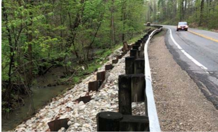
Photograph 4: Geohazard site between SLM 22.961 and SLM 23.035
