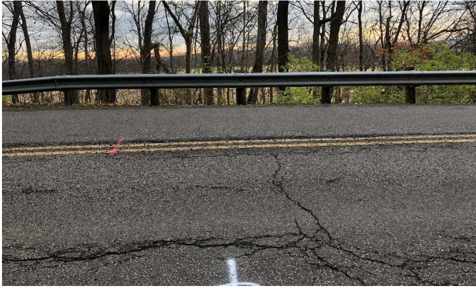
Photograph 1: Overall Pavement Condition of CR-222
